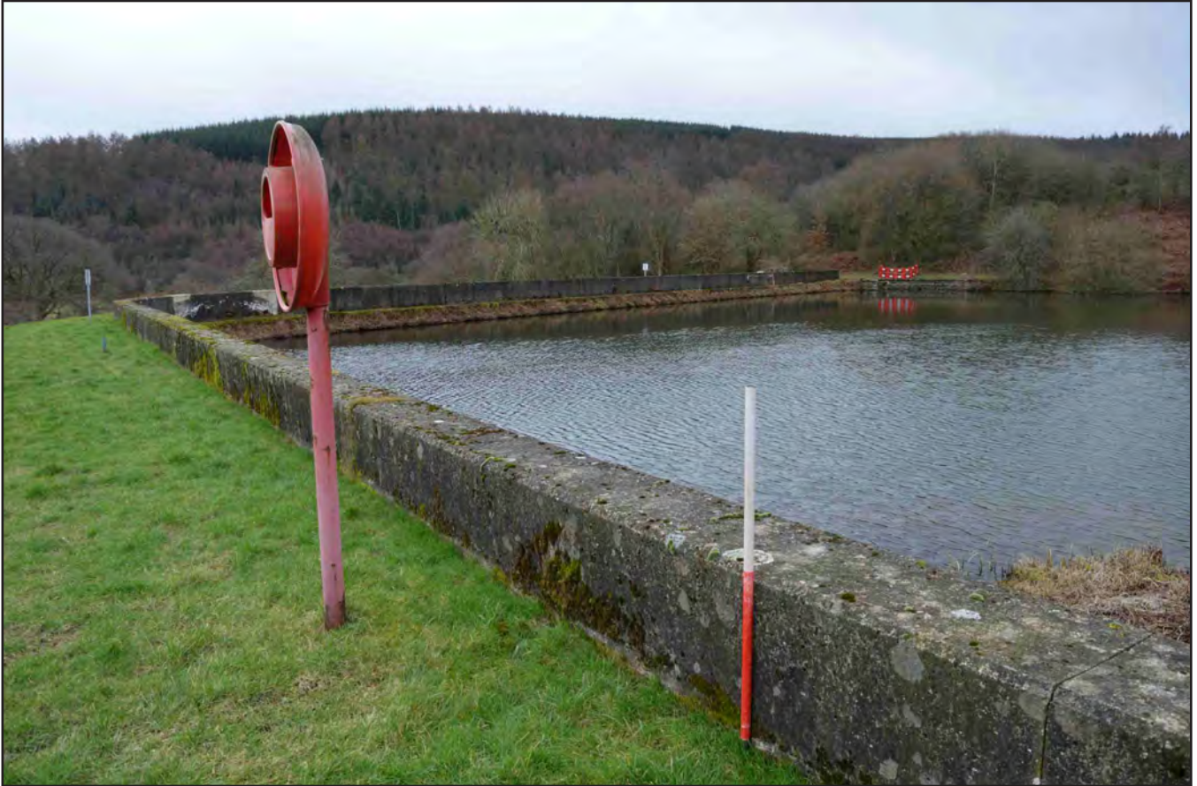
Plate 05: Concrete addition on top of Victorian retaining wall; scale 1x1m (archive reference: G2596_008)
