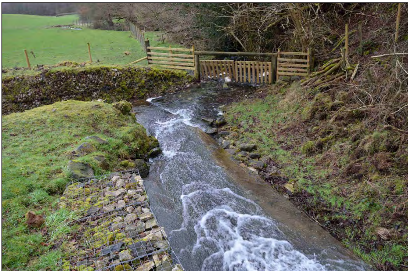
Plate 10: Gabion basket reinforcement at base of spillway; no scale (archive reference: G2596_019)
