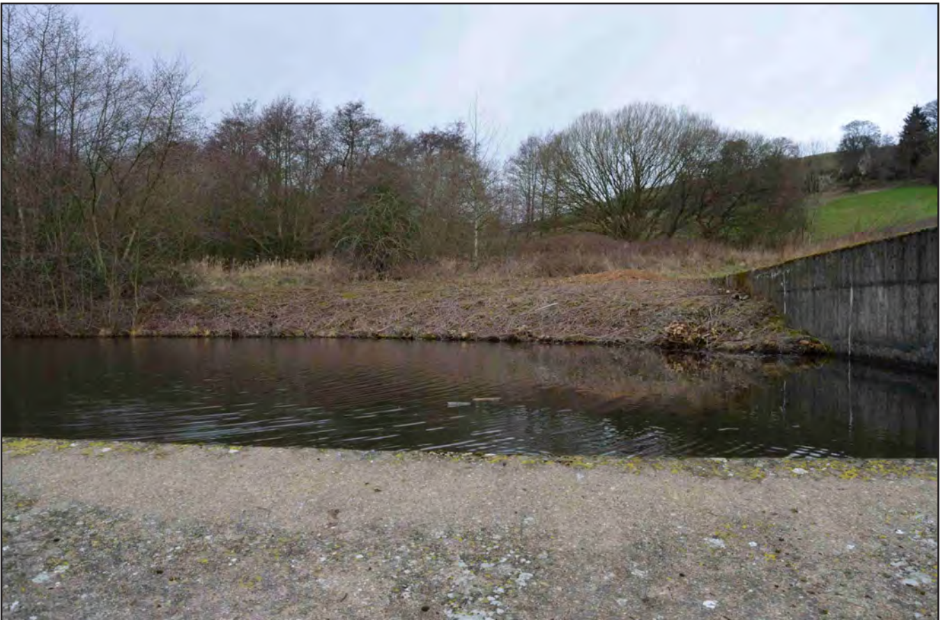
Plate 02: Concrete retaining wall adjacent to spillway access; no scale (archive reference: G2596_005)
