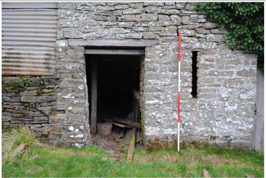
Plate 138. Entrance to looseboxes (or personnel door) and ventilation slit on the western elevation (Bay F). Looking east-southeast.
