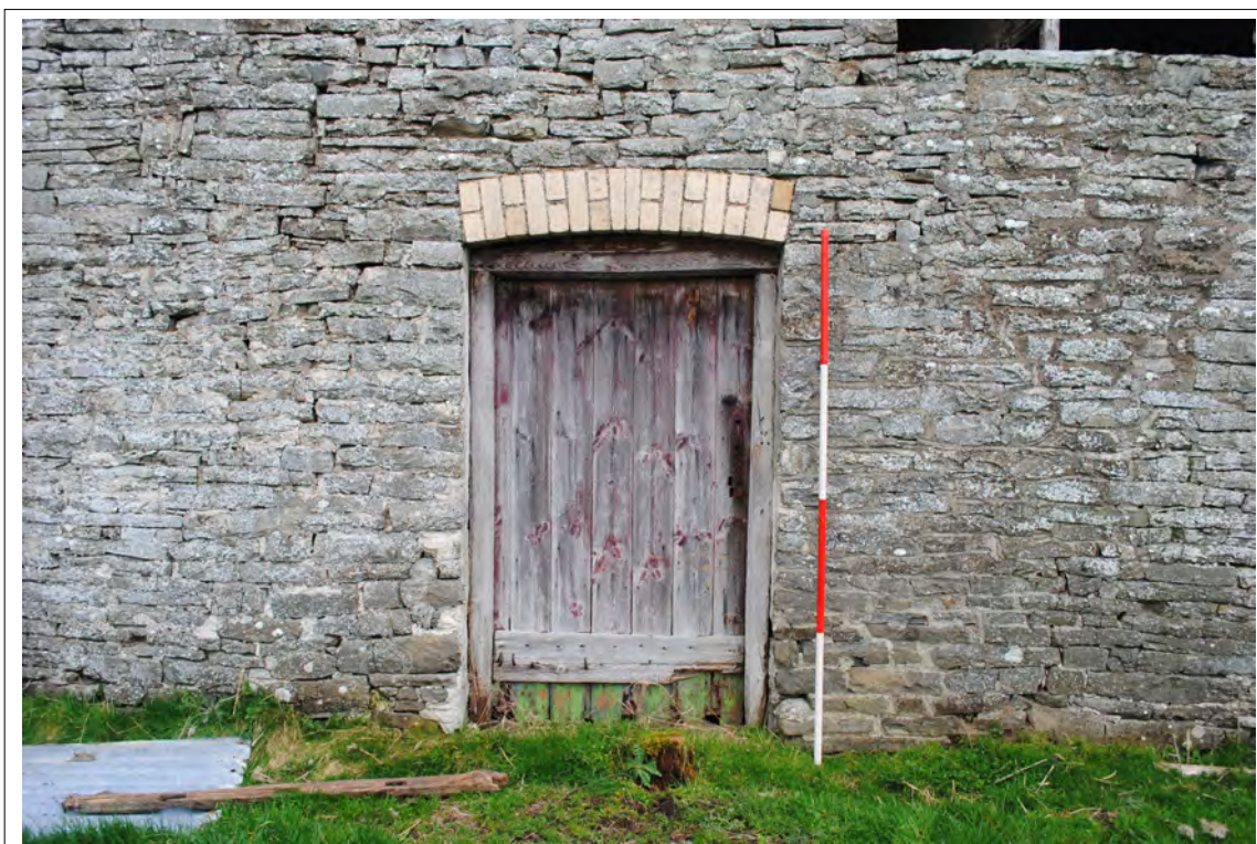
Plate 30. The front entrance to the western part of the farmhouse (southern elevation). Looking north.
