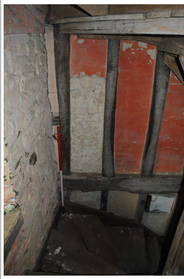
Plate 83. Detail of the exposed timber-framed wall on the eastern side of the staircase.
