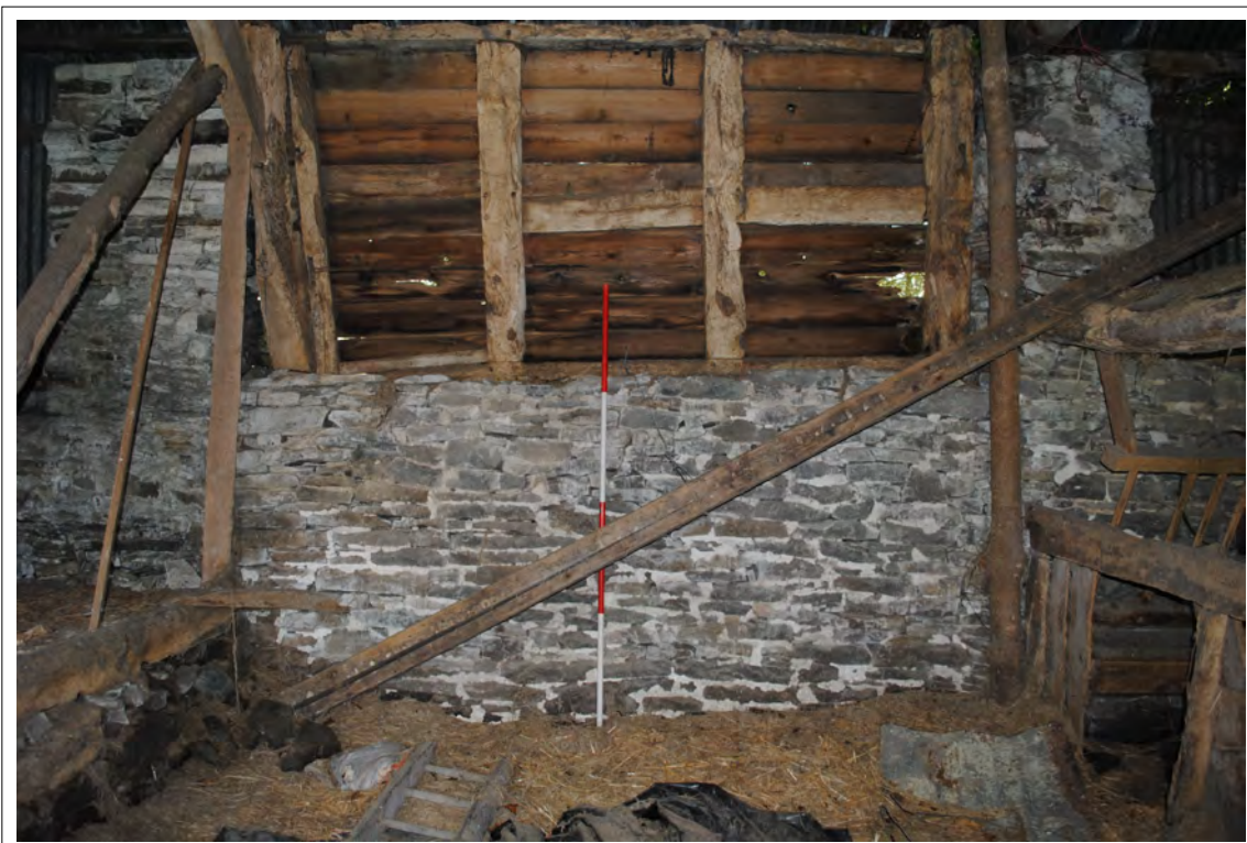
Plate 175. Lower section of the eastern elevation of Bay E, showing timber-framing over a masonry wall.
