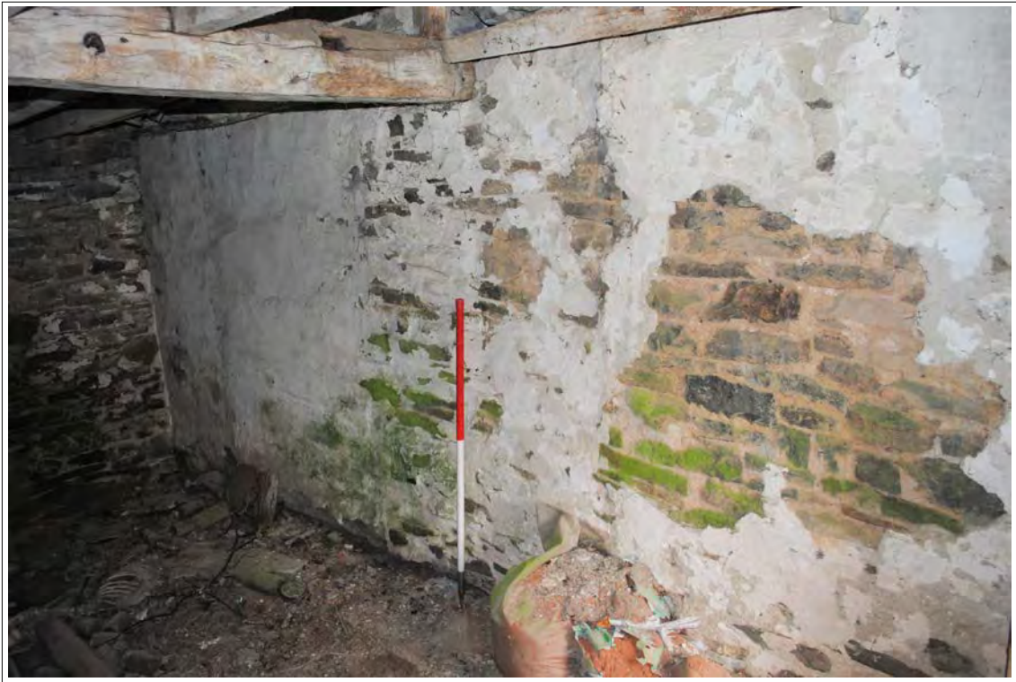
Plate 125. Oblique view of the southern wall, with sections of lime plaster. Looking east-southeast.
