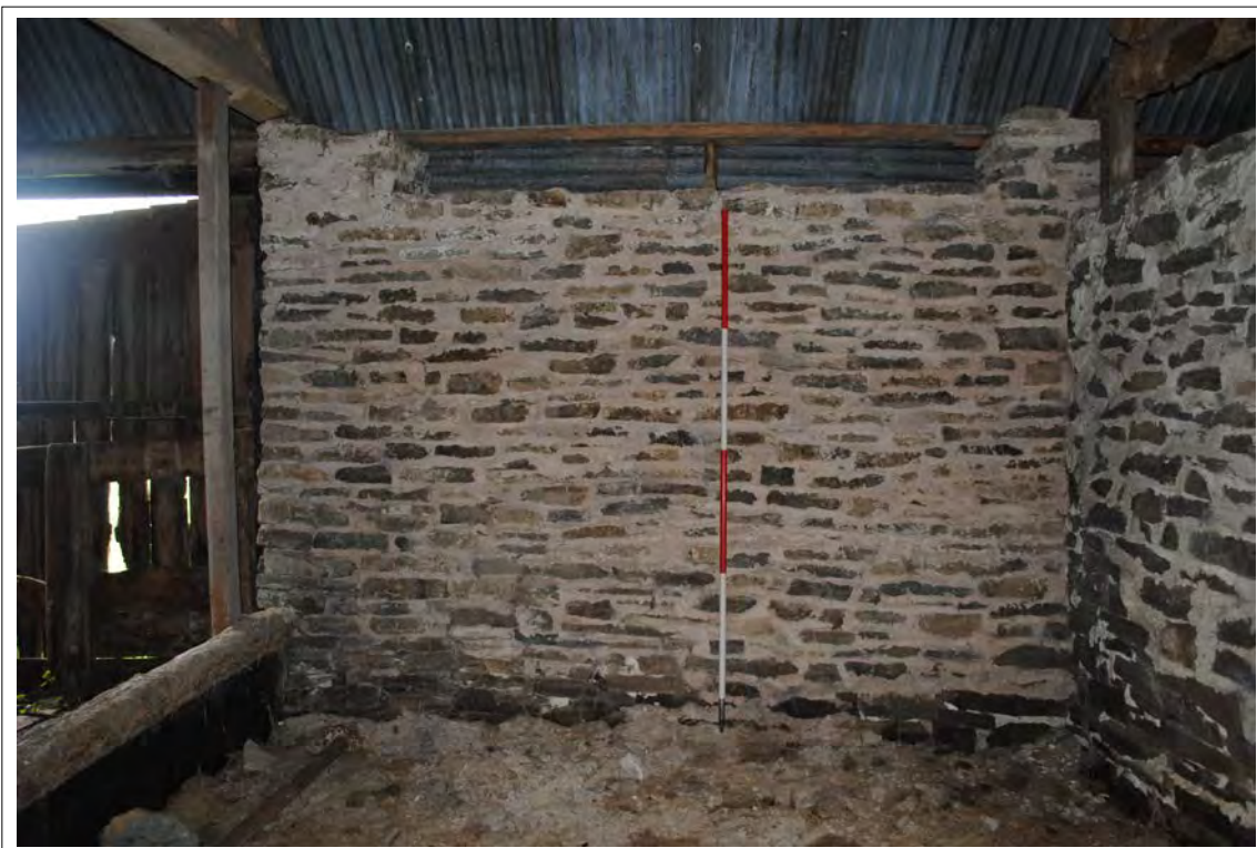
Plate 167. The western elevation of Bay C, showing a full-height masonry wall supporting Trusses B and C.
