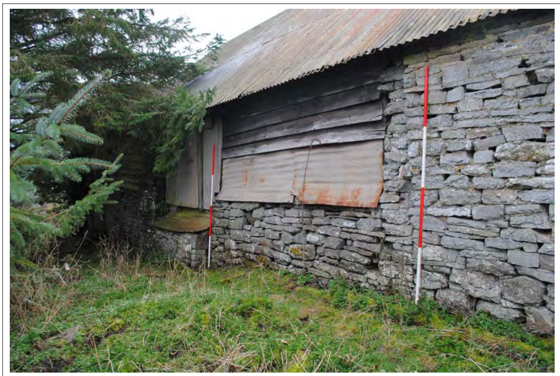
Plate 150. Oblique view of the back wall of Bay C of the barn (eastern elevation). Looking west-southwest.
