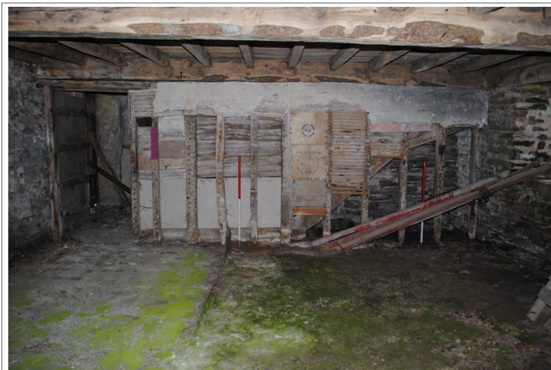
Plate 63. Western side of Room 1, showing lath-and-plaster over timber-framed internal wall, with a doorway (to the hall) on the left.
