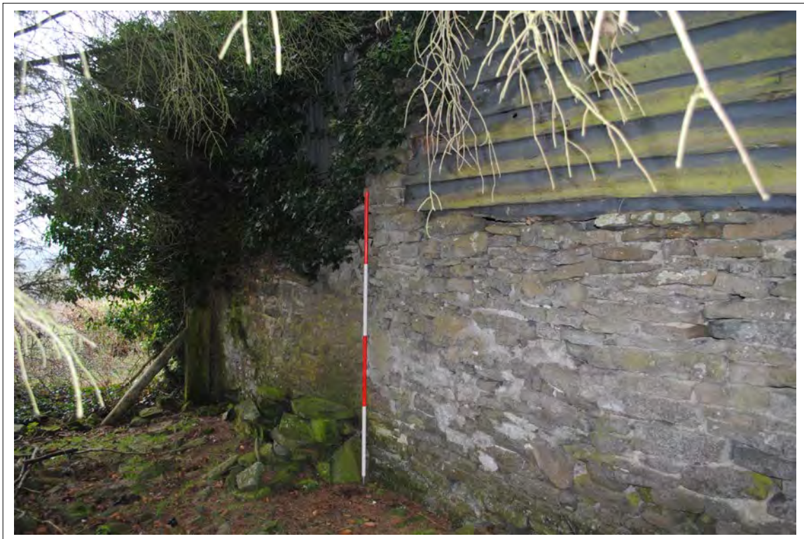
Plate 154. Oblique view of Bays E and F, the back wall of the former barn and cowhouse (eastern elevation). Looking south-southwest.
