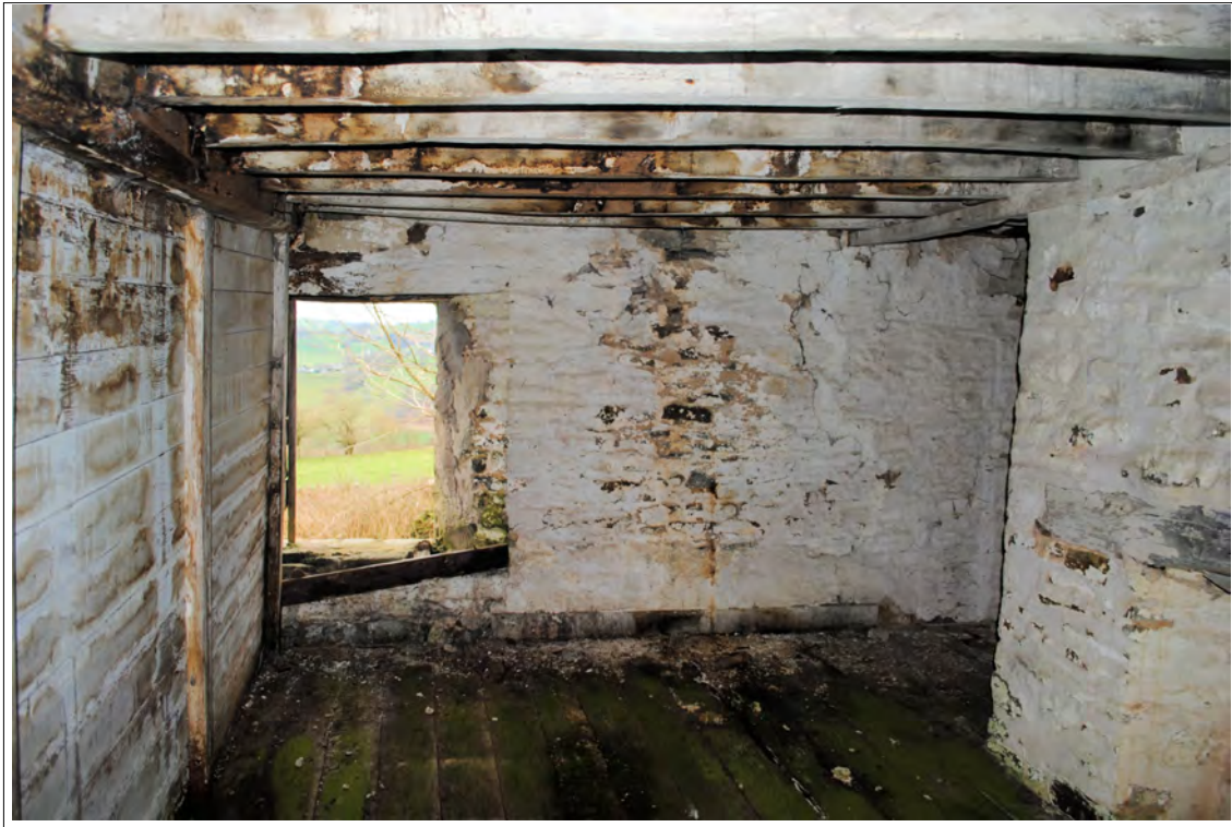
Plate 97. In Room 4b, the timber partition divides the central window on the southern wall (front of the farmhouse).
