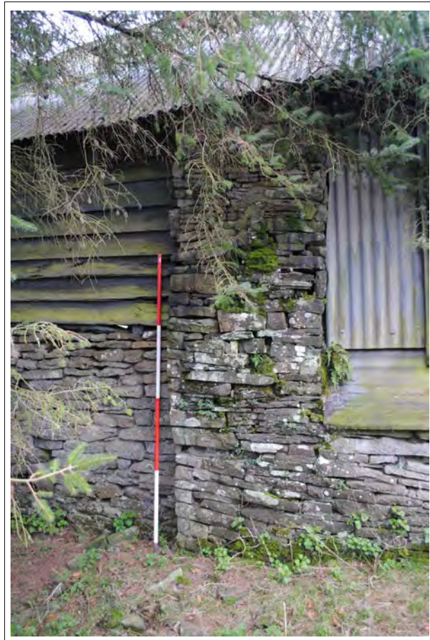
Plate 152. Detail of the separate phases of stonework between Bays D and E (eastern elevation). Looking west.
