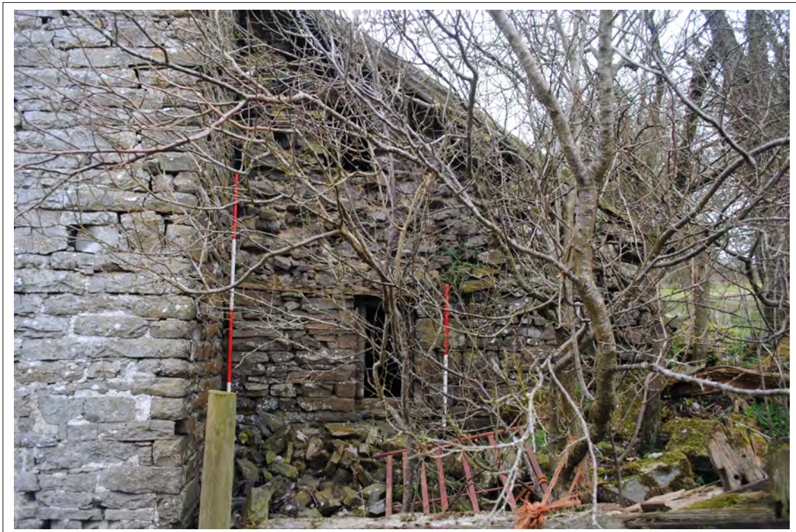
Plate 40. The lower ventilation slit and collapsed upper opening on the eastern side of the lean-to. Looking west.
