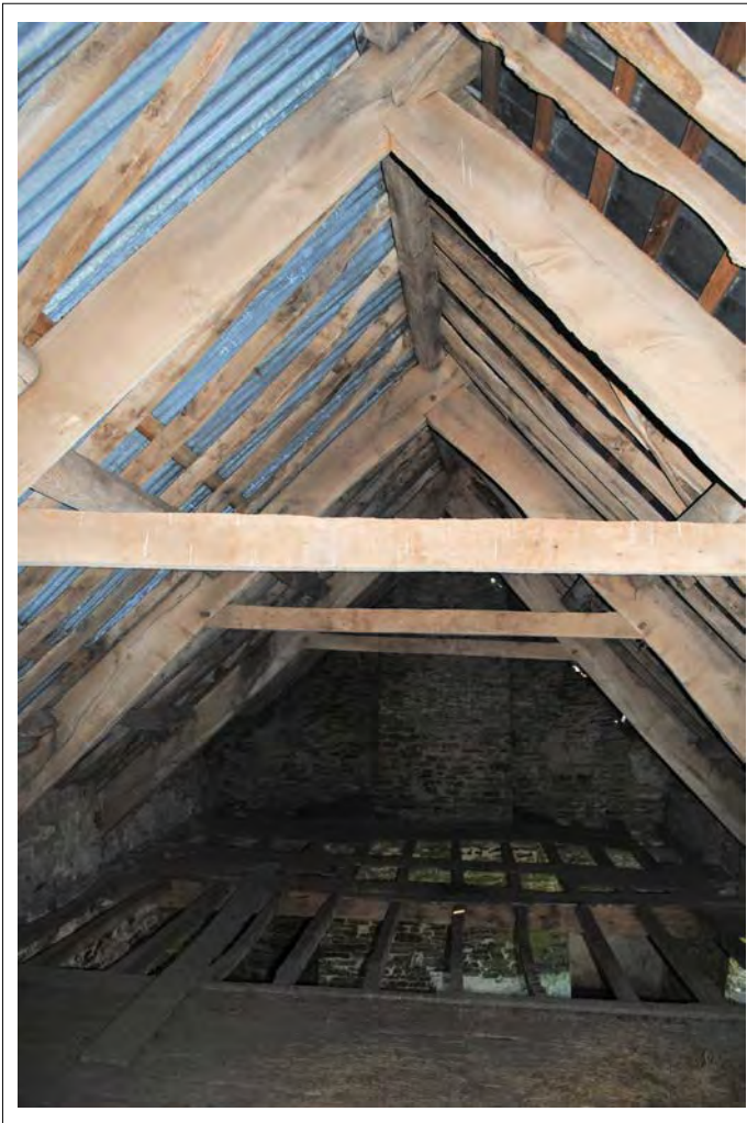
Plate 111. General view of trusses within the eastern part of the farmhouse. Looking east.
