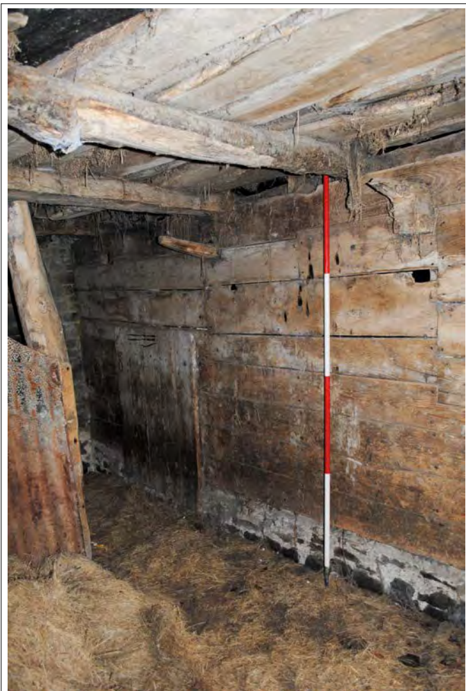
Plate 157. The timber-framed and boarded partition between Bays A and B, with harness hooks. Looking southeast.
