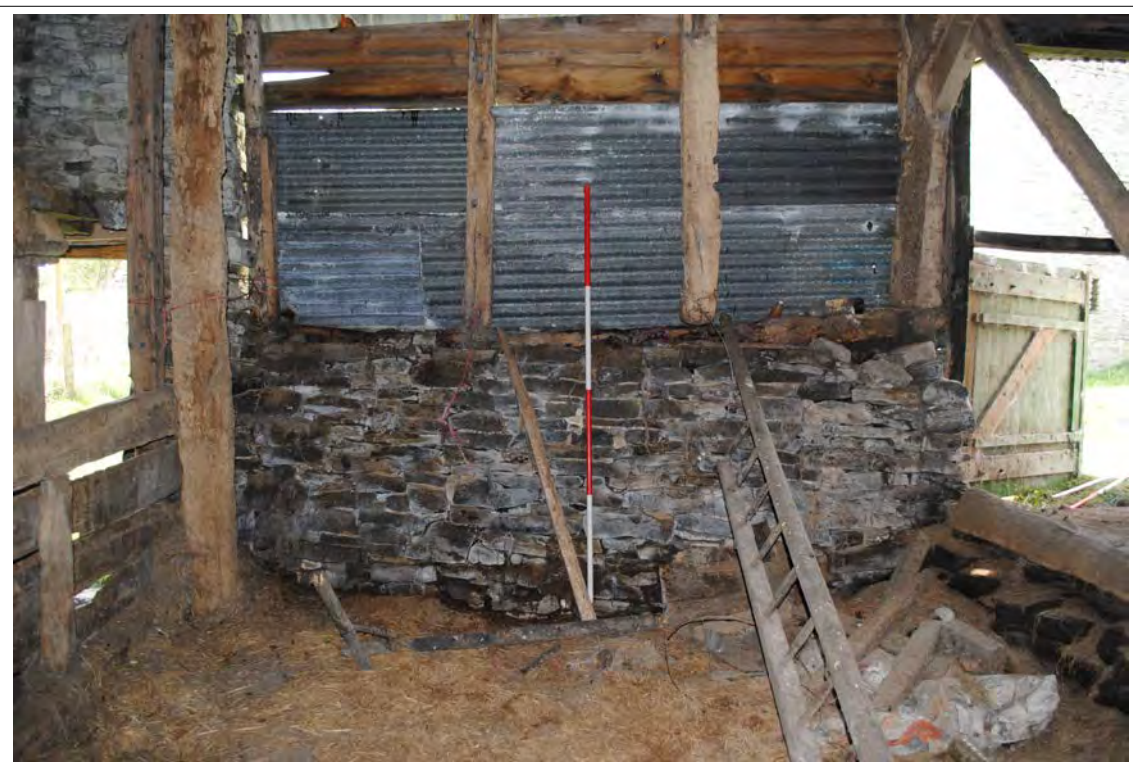
Plate 172. Lower section of the western elevation of Bay E, showing timber-framing over a masonry wall.
