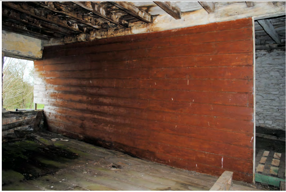
Plate 93. Modern timber partition viewed from Room 4a, dividing the original upstairs room. Looking southwest.
