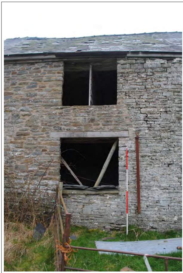
Plate 28. Front windows of the western part of the farmhouse, showing rebuilt stonework (southern elevation). Looking north.
