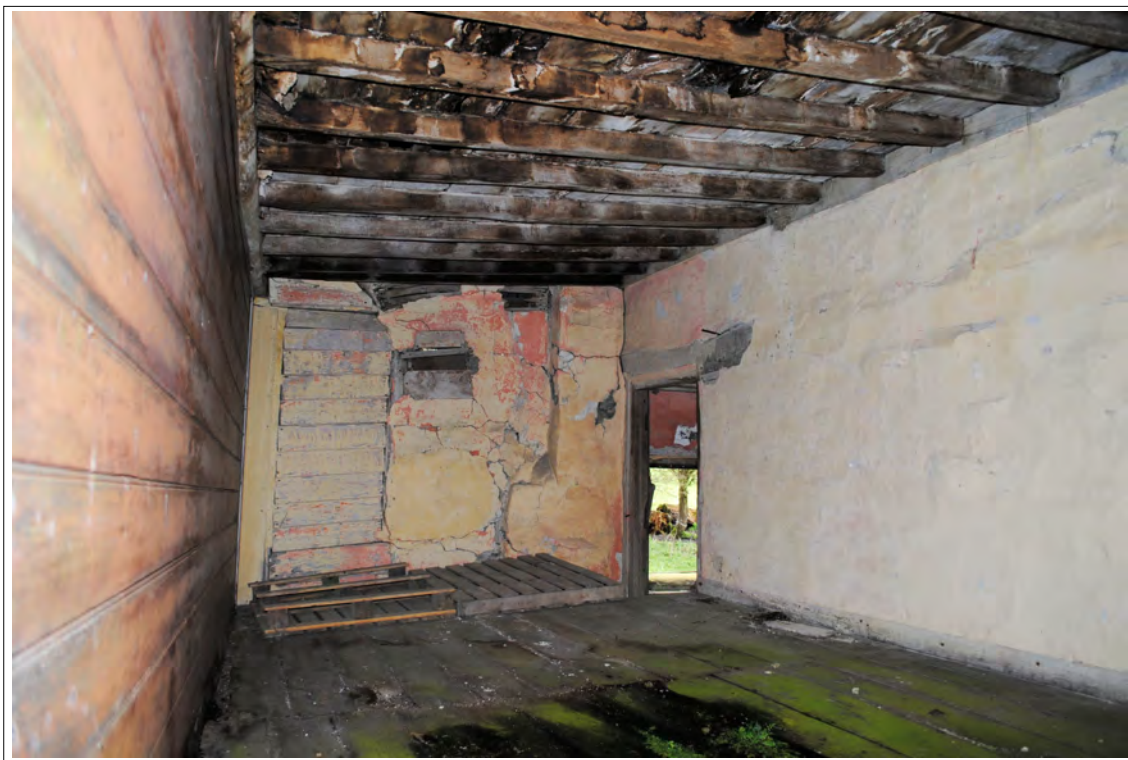
Plate 92. View towards the northern wall of Room 4a, with doorway to landing, showing painted plaster over boarded external timber-frame wall.
