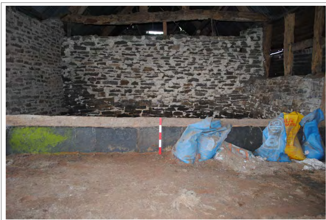
Plate 168. A low stone slab partition wall with cill dividing Bays C and D. Looking north-northeast.
