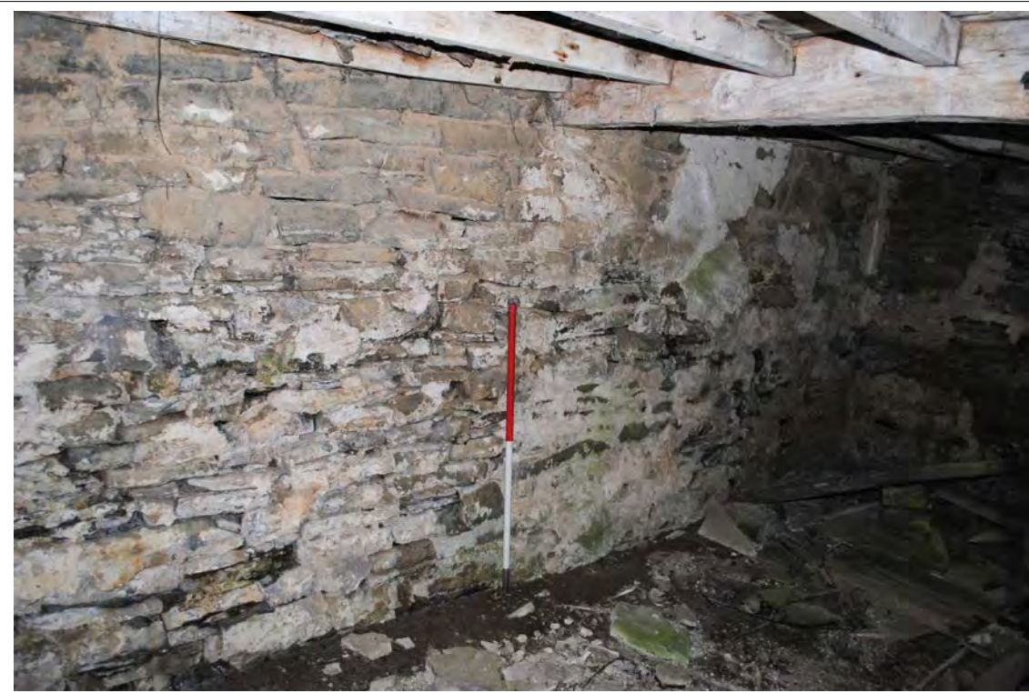
Plate 126. Oblique view of the northern wall, with limewash and patches of lime plaster. Looking east-northeast.
