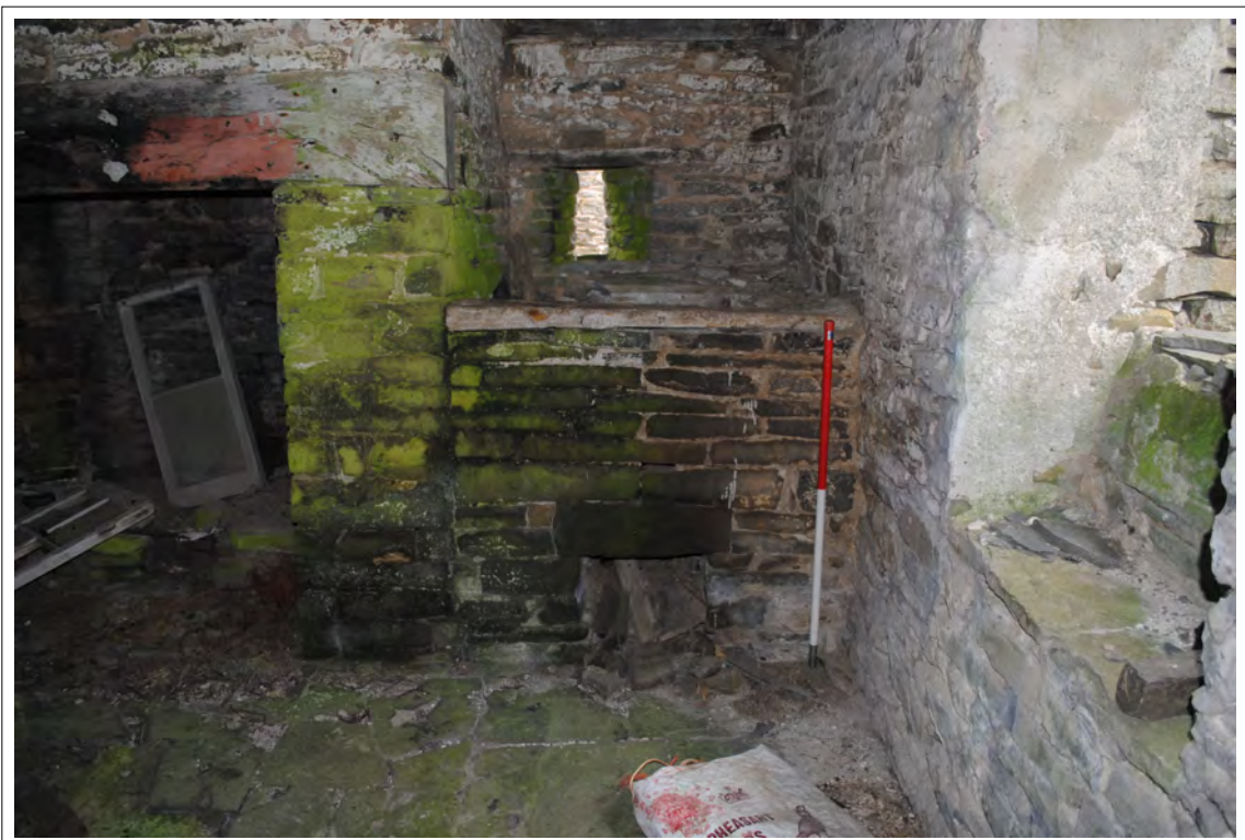
Plate 53. Probable structure for 'copper' adjacent to the fireplace on the eastern wall of Room 1.
