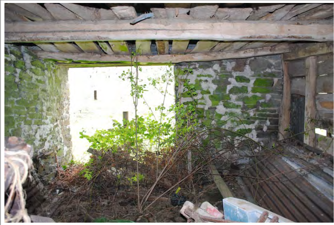
Plate 161. The cartshed entrance (western wall), showing timbers for the hayloft above. Looking west-northwest.
