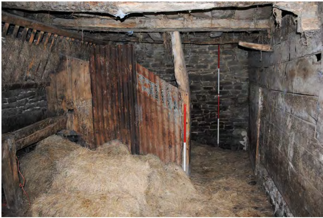
Plate 155. General view of the stable, showing the cobbled floor and partition for a single stall (Bay A). Looking east-southeast.
