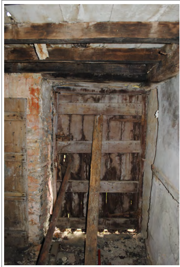
Plate 80. Front entrance to the western side of the farmhouse on the southern wall of the hall.
