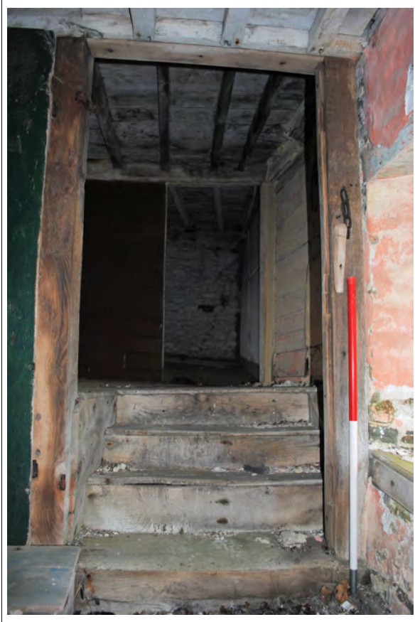
Plate 91. Steps from the landing to Room 4a of the farmhouse. Looking west.
