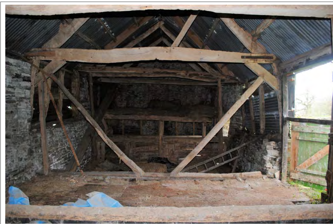
Plate 171. General view of Bays C to G, showing bracing in the foreground for Truss D. Looking south-southwest.
