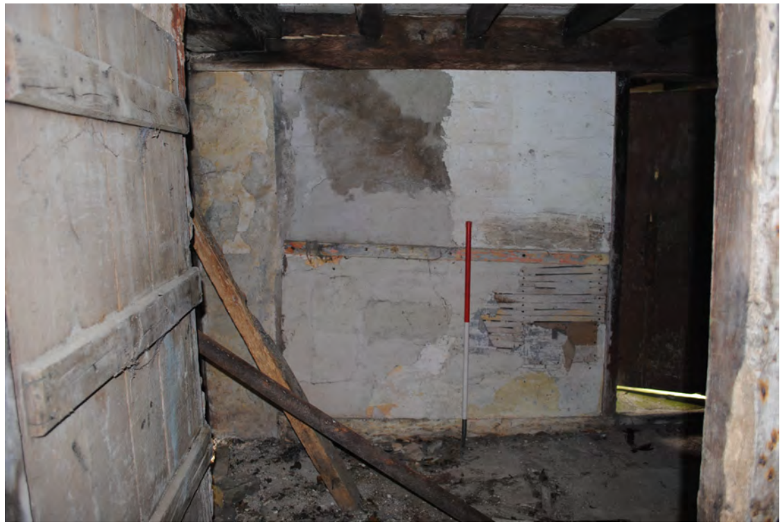
Plate 81. The western side of the hallway, showing lath-and-plaster over a timber-framed internal wall.
