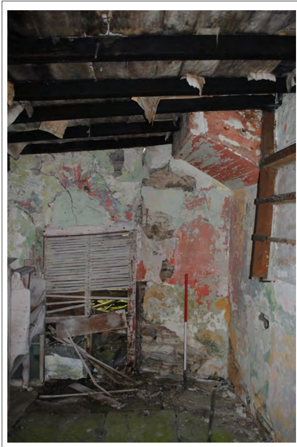
Plate 75. The northwest corner of Room 2, showing partly exposed timber frame abutting an external stone wall.
