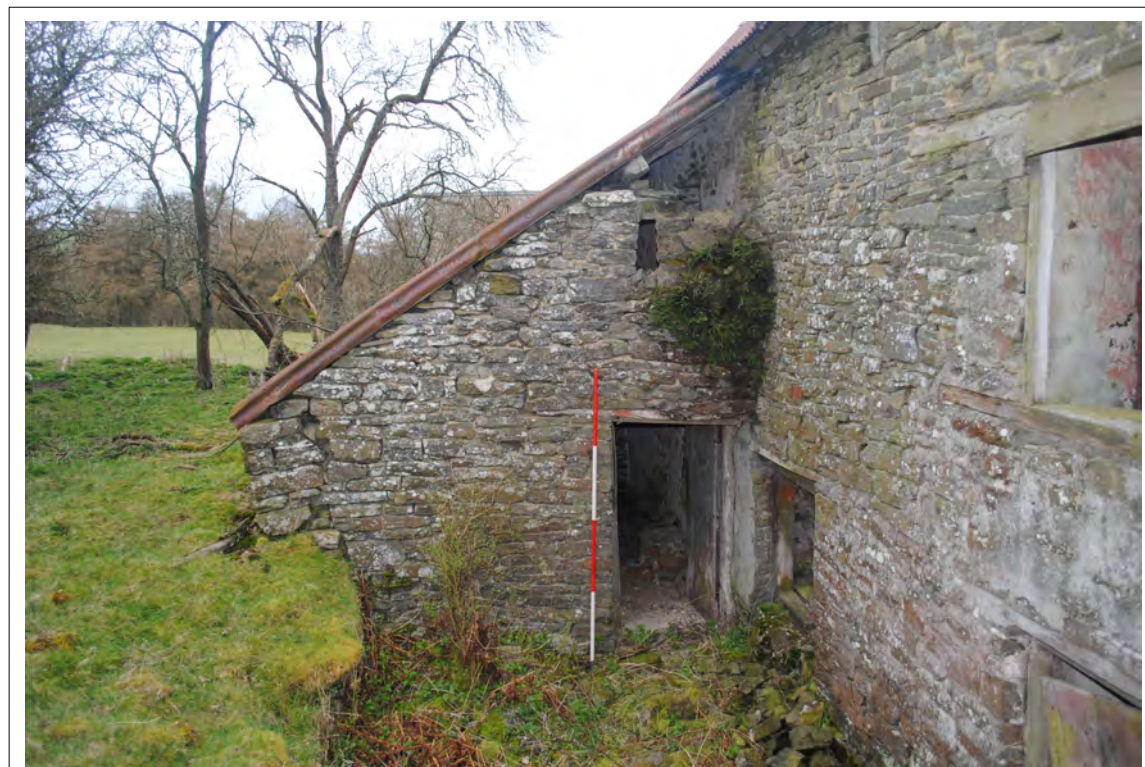
Plate 44. The western elevation of the lean-to, with doorway and upper ventilation slit. Looking east-southeast.
