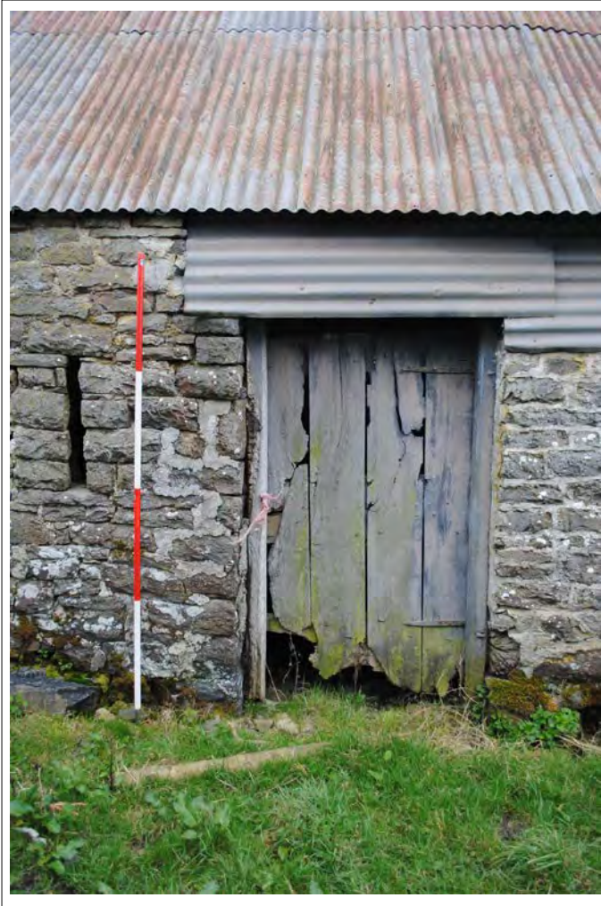
Plate 143. View of the entrance and ventilation slit on the western elevation for a stable (Bay A). Looking east-southeast.
