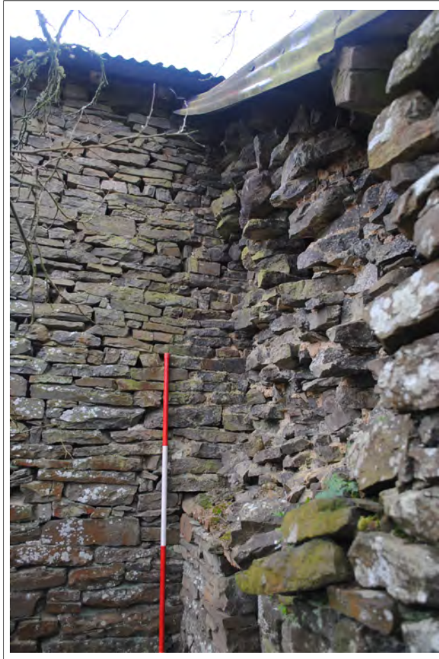
Plate 39. Oblique view of the partly collapsed eastern wall of a lean-to on the the northern elevation. Looking south-southwest.
