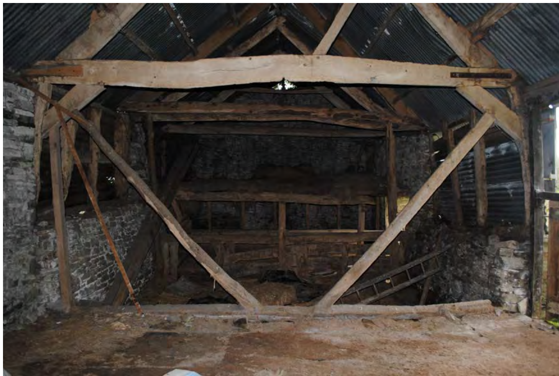
Plate 201. View across Bays D-G. Bracing timbers below Truss D are shown in the foreground. Looking south-southwest.
