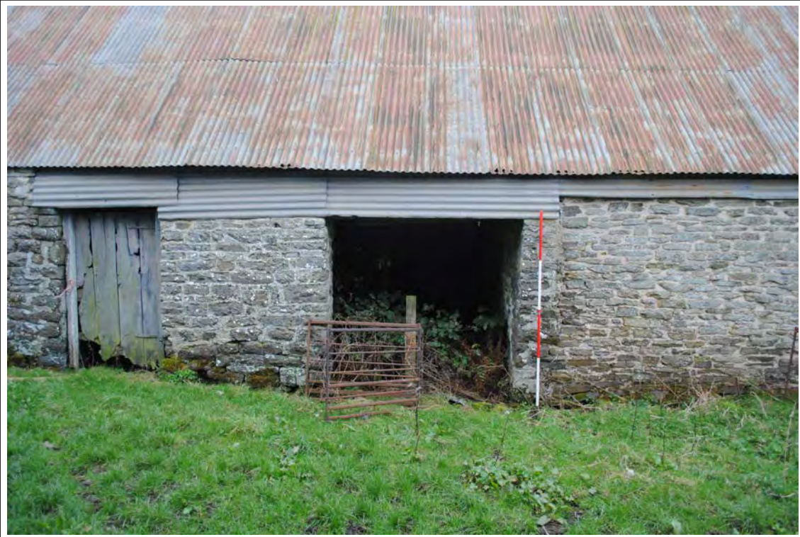
Plate 141. The entrances to the stables on the left (north) and cartlodge on the right (south) along the western elevataion. Looking east-southeast.
