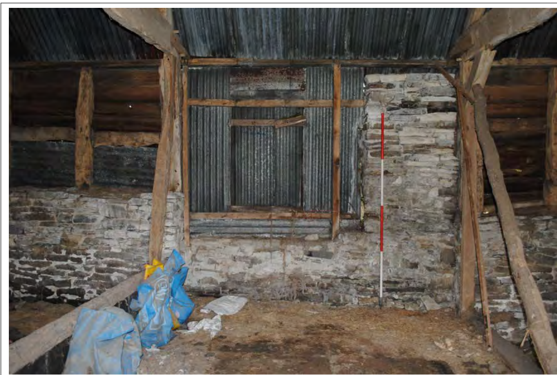
Plate 169. The eastern elevation of Bay D, showing masonry infill (set back from Bay C) and modern timber-framing.
