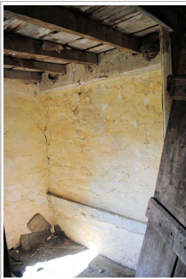
Plate 98. General view of the western side of Room 5, showing painted lath-and-plaster over an internal timber-frame wall. Looking southwest.
