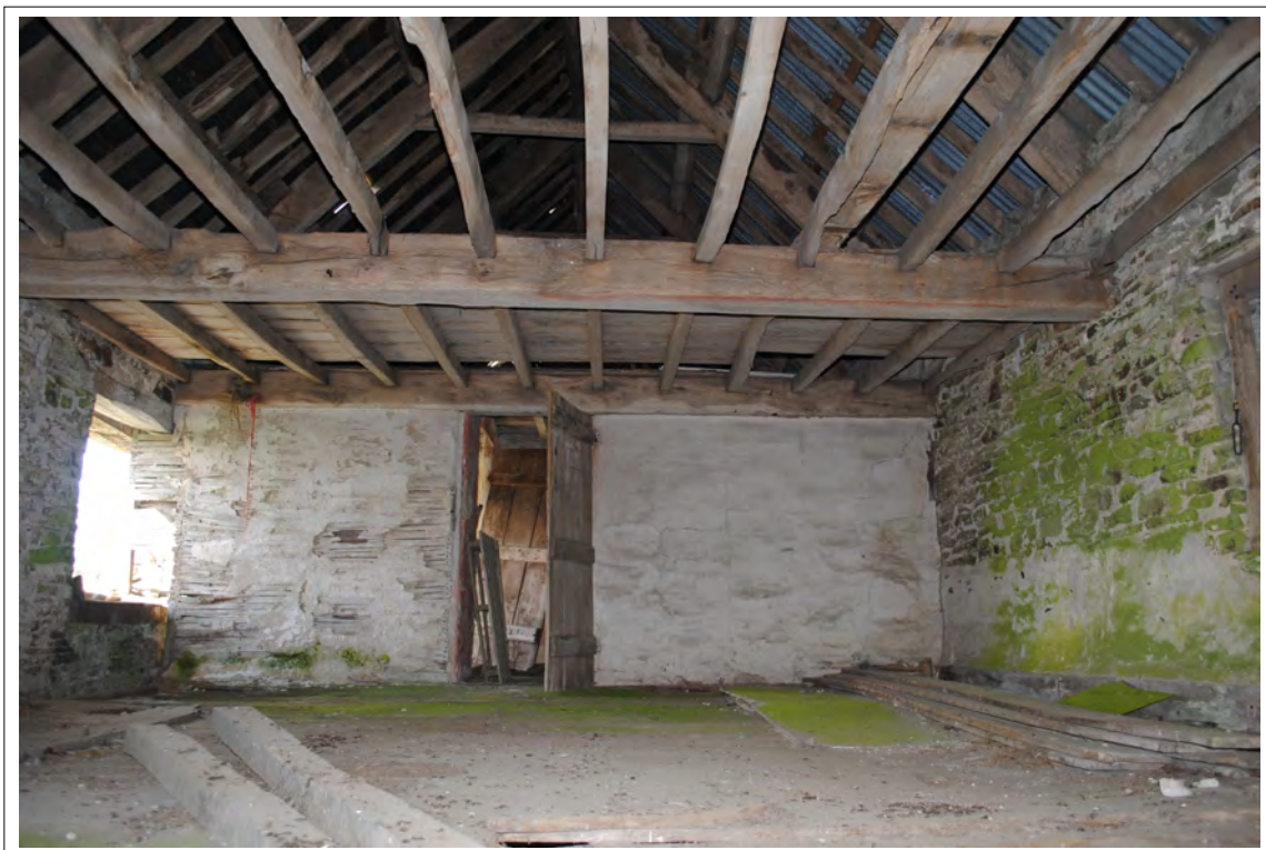
Plate 85. The west side of Room 3, showing whitewashed lath-and-plaster over a timber-frame internal wall.
