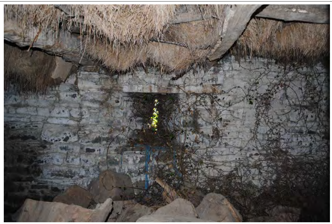
Plate 180. The central ventilation slit in the south gable wall (Bay G). Looking south-southwest.
