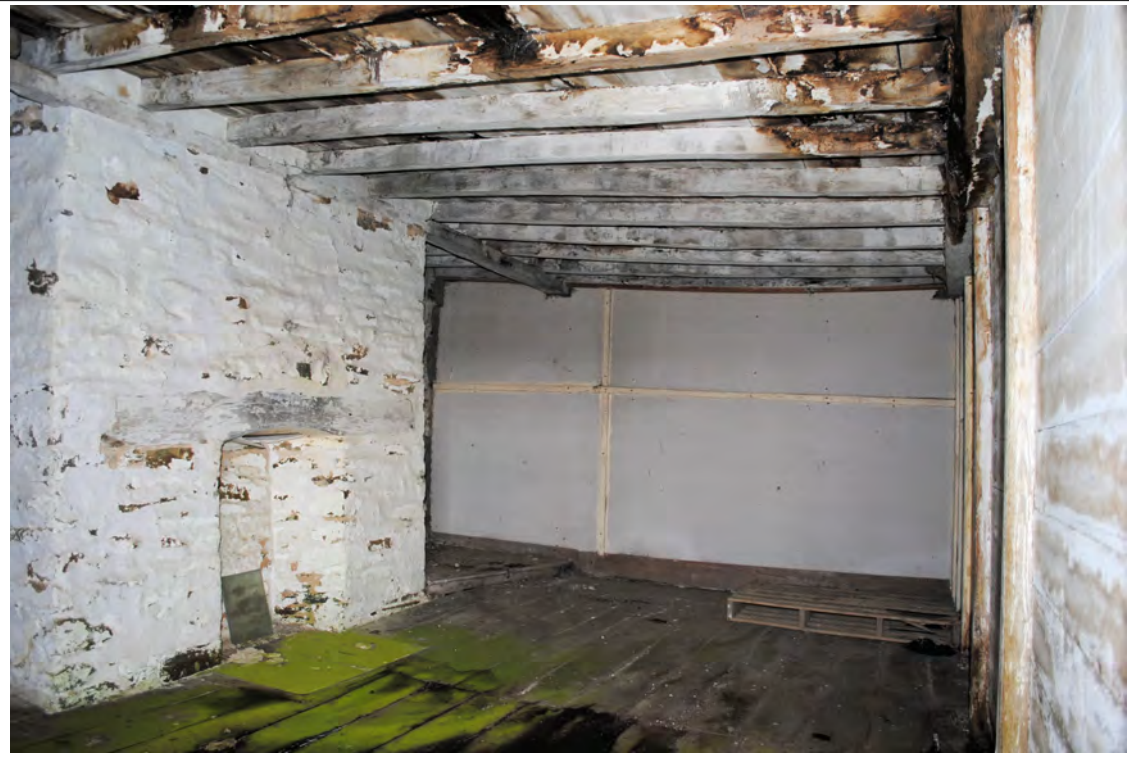
Plate 95. View towards the northern wall of Room 4b, with doorway from Room 4a, showing modern board over external timber-frame wall.
