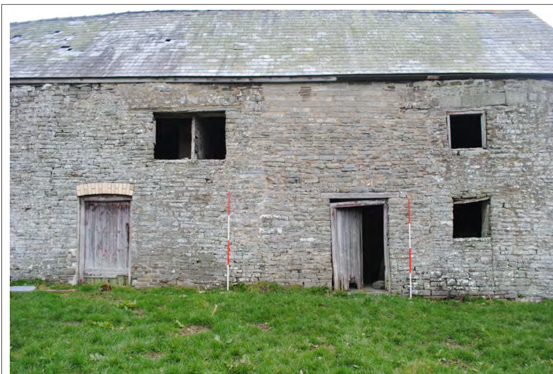
Plate 31. View of different phases of stonework on the southern elevation, between the two doorways, with rebuilt sections above the right (east) entrance and above both upper windows. Looking north.
