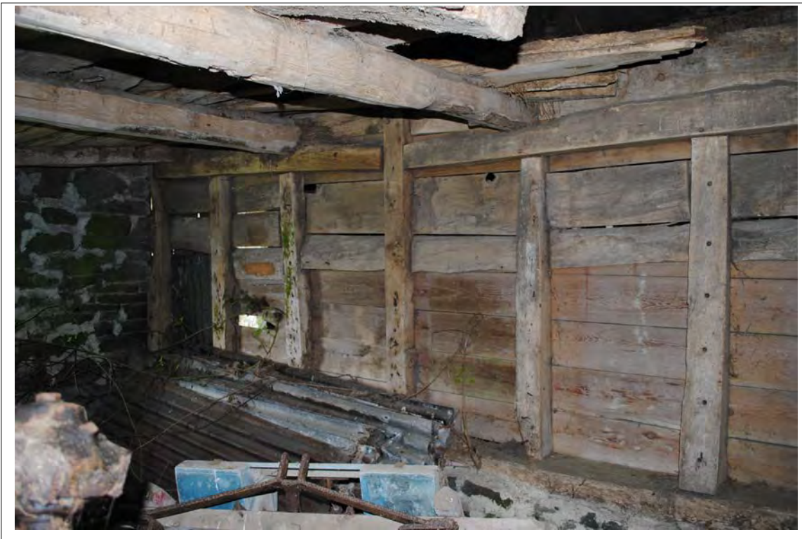
Plate 159. The timber-framed and boarded partition between Bays A and B, built over a low stone wall. Looking northwest.
