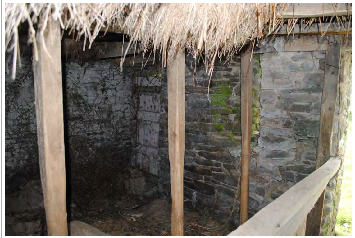
Plate 181. Oblique view of the doorway and ventilation slit along the western wall of Bays F and G. Looking southwest.
