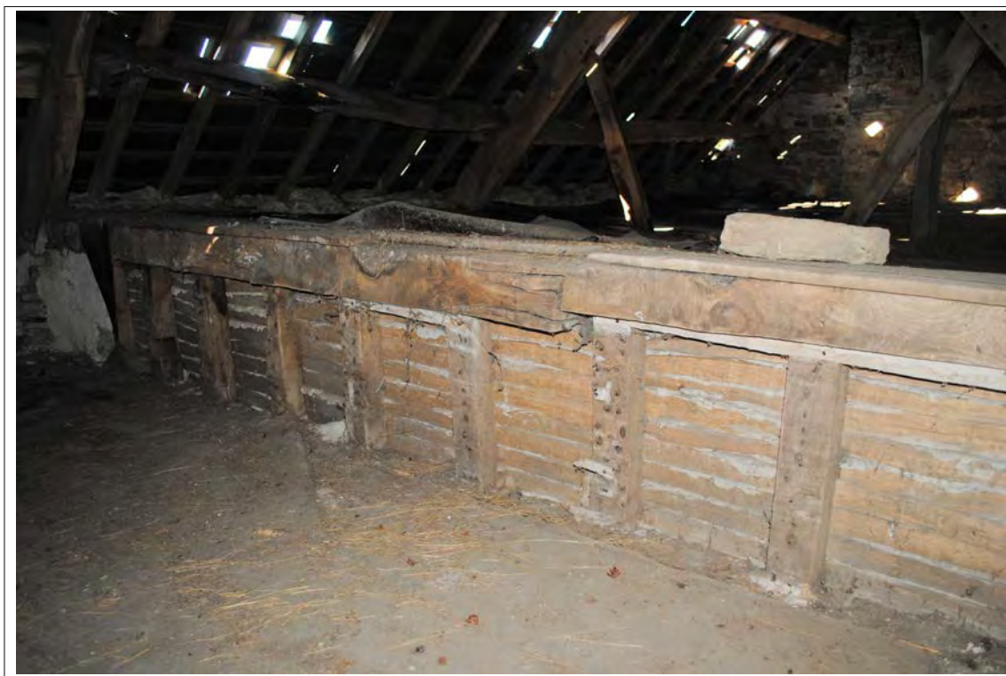
Plate 110. Oblique view of the stud wall extending into loft (top of the eastern wall of Room 4a). Looking southwest.
