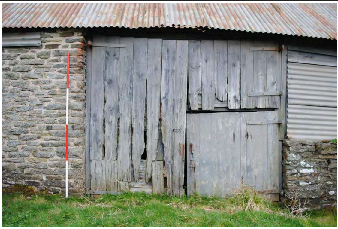
Plate 140. The entrance to the main barn, Bay D (western elevation). Looking east-southeast.
