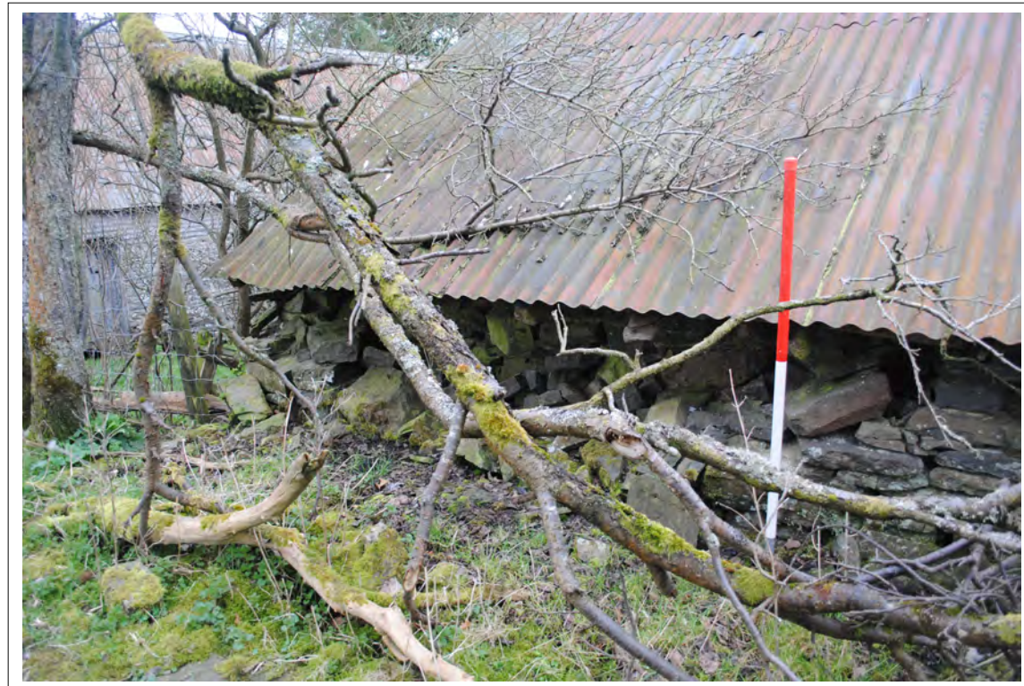
Plate 42. Detail of collapsed walling at the northeast corner of the lean-to (viewed along the northern elevation). Looking southeast.
