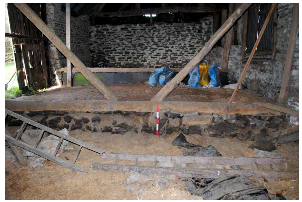
Plate 174. View of the masonry dividing wall where the floor level drops between Bays D and E. Looking north-northeast.
