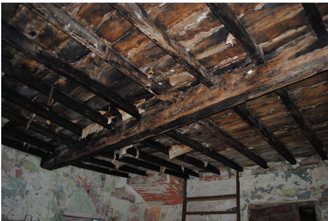
Plate 78. General view of the ceiling in Room 2, showing blackened timbers resulting from fire. Looking northeast.
