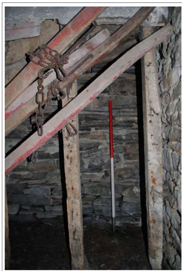
Plate 64. Detail of the stone wall supporting a staircase, viewed from the western side of Room 1.
