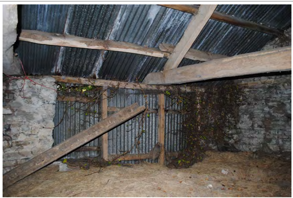
Plate 184. Oblique view of the eastern wall of the hayloft, showing modern timberwork (Bays F & G). Looking southeast.
