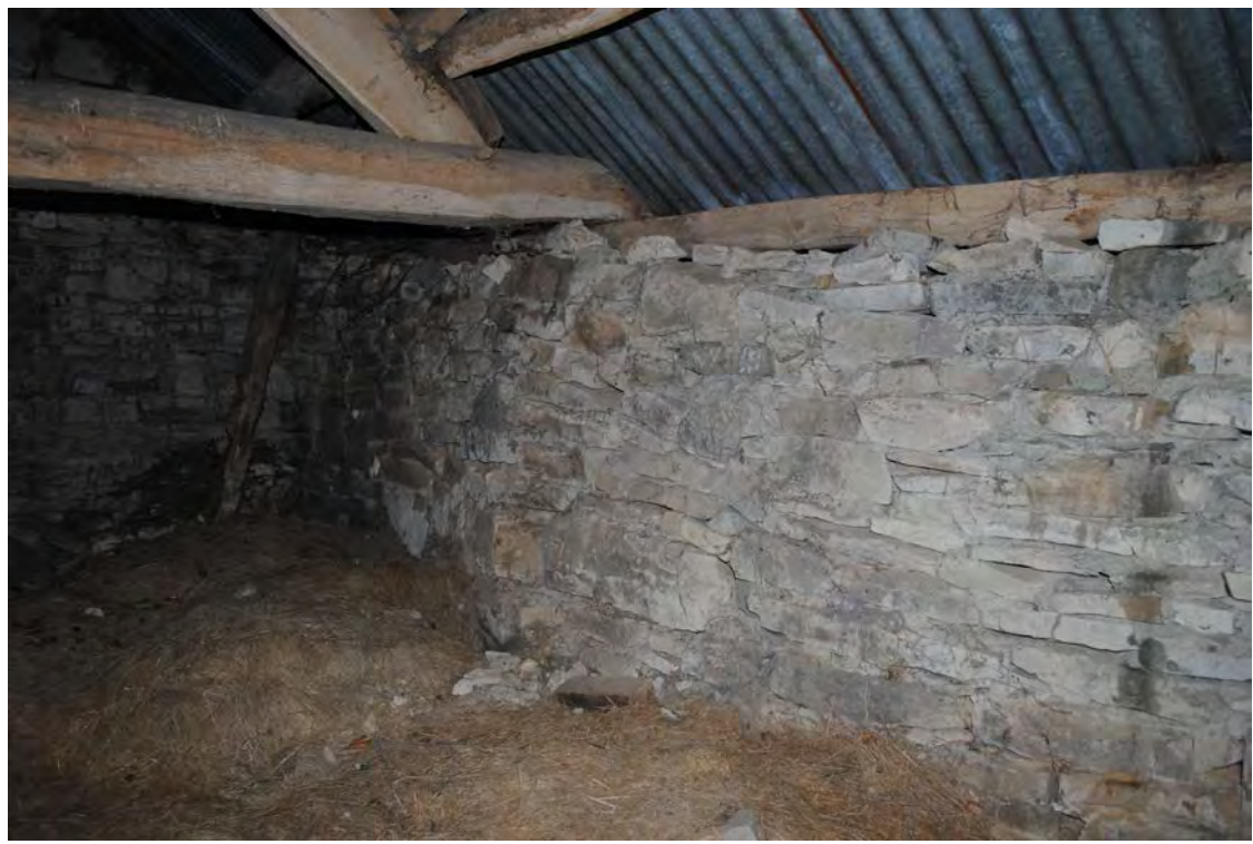
Plate 185. Oblique view of the western wall of the hayloft, showing bowing masonry (Bays F & G). Looking southwest.
