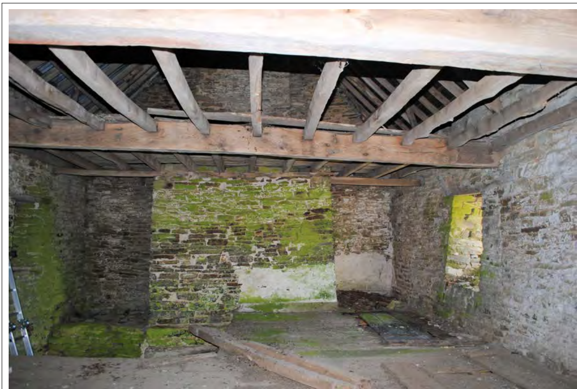
Plate 89. General view of the eastern wall in Room 3, with central chimney stack.
