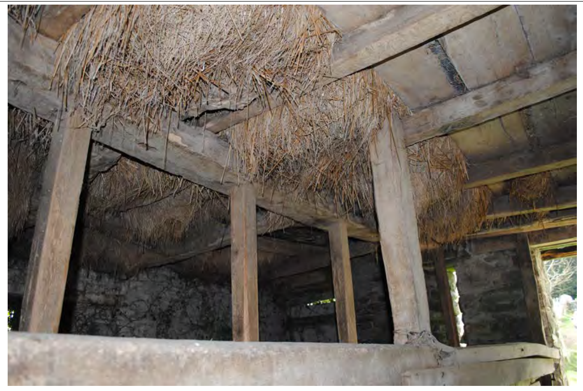
Plate 182. Detail of the timberwork for the hayloft above the probable cowhouse (Bays F & G).
