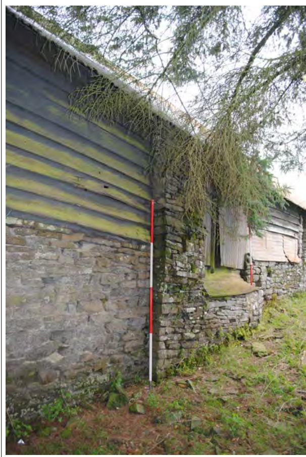
Plate 151. Oblique view of the back wall of Bay D of the barn (eastern elevation). Looking north.
