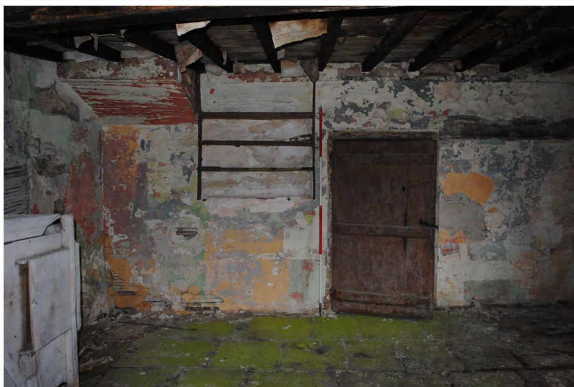
Plate 76. The eastern side of Room 2, showing lath-and-plaster over an internal timber-framed wall.
