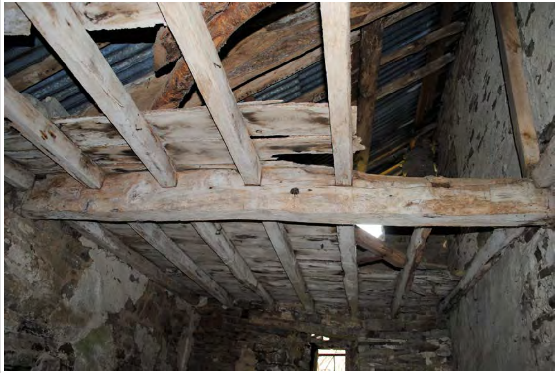
Plate 131. General view of the ceiling beam, joists and boards for the loft area. Looking East
