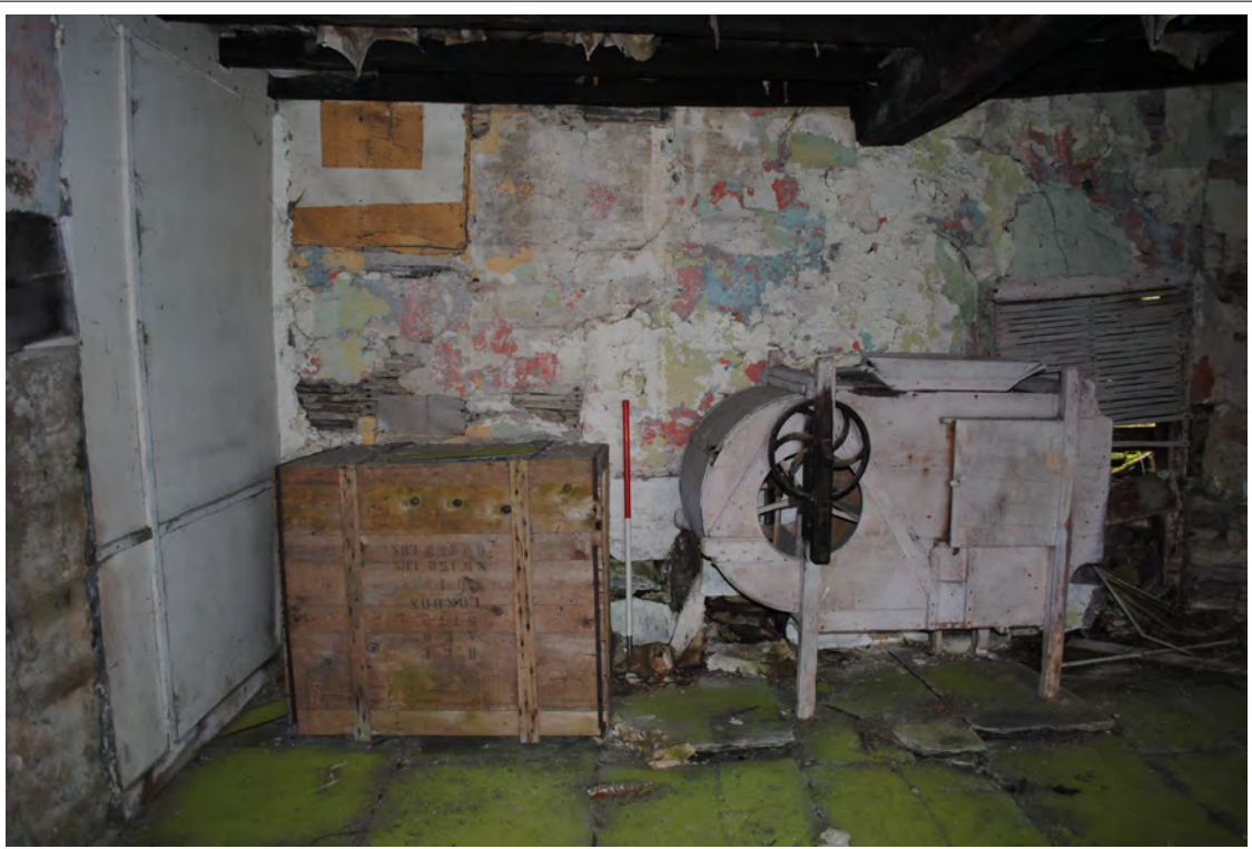
Plate 74. The northern side of Room 2, showing lath-and-plaster over a timber-framed external wall.
