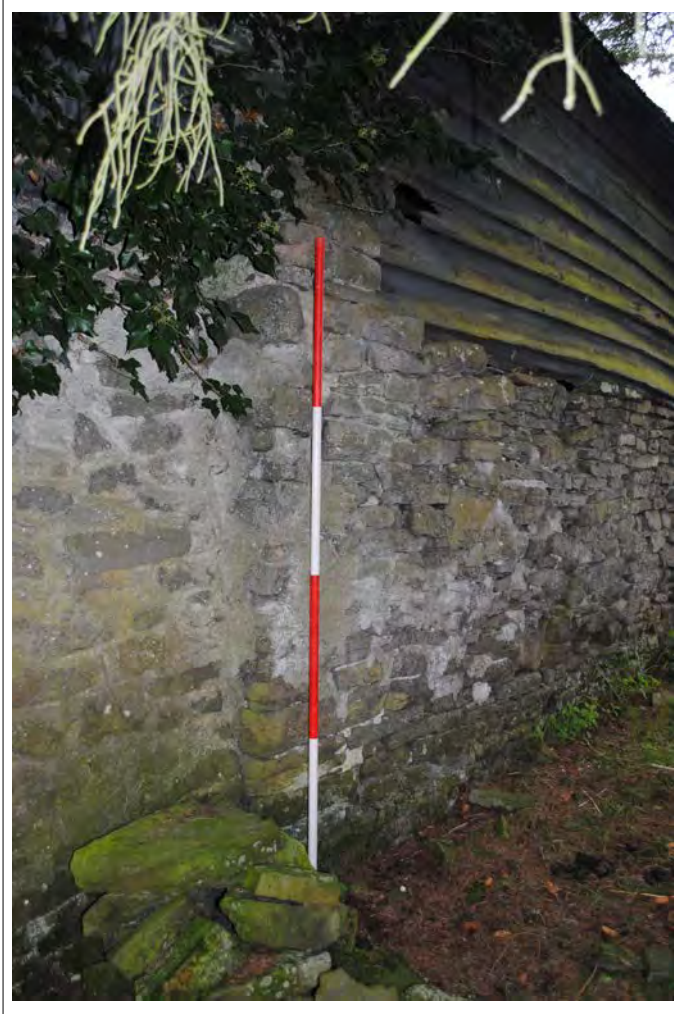
Plate 153. Oblique view of the separate phases of stonework between Bays E and F (eastern elevation). Looking north.
