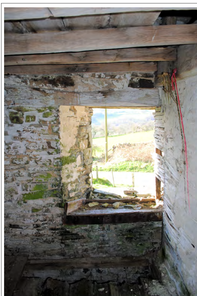
Plate 86. In Room 3 the timber partition divides the western window on the southern wall (front of the farmhouse).
