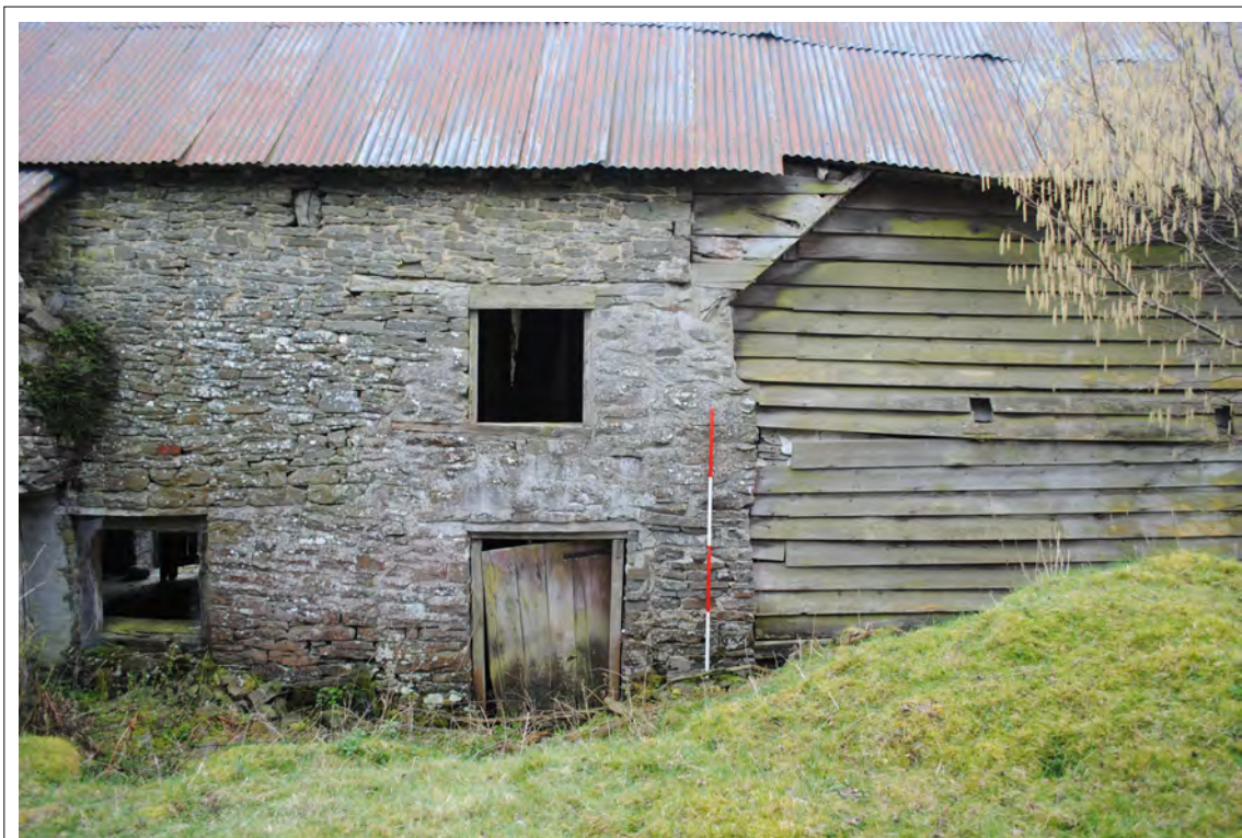
Plate 47. Probable former pillar originally for opening to west (right), now weatherboarded. Looking south.
