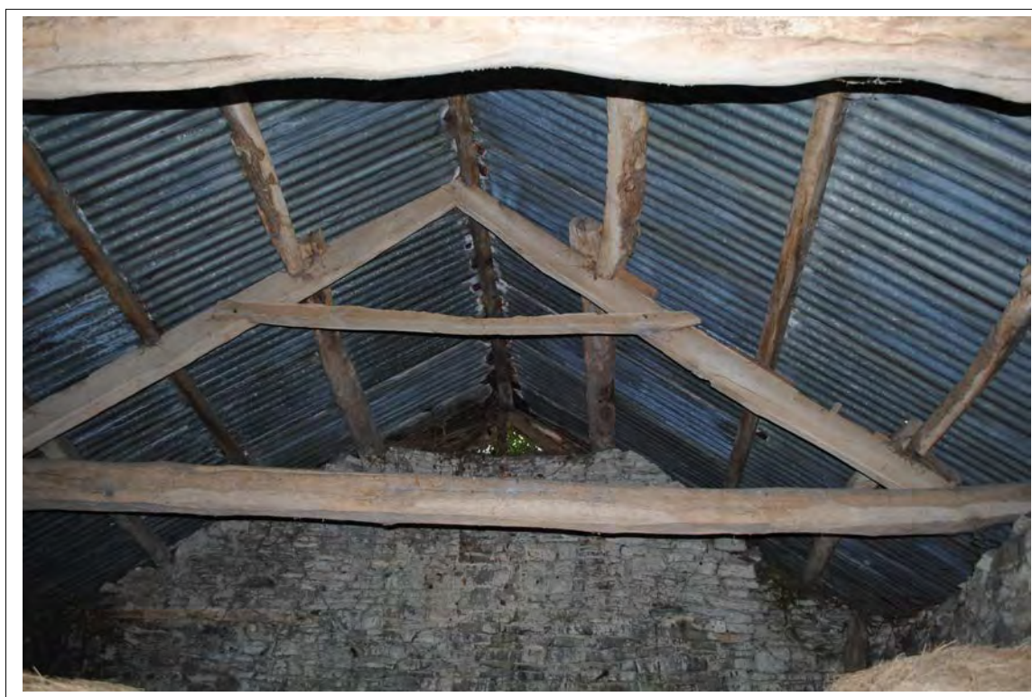
Plate 210. General view of Truss F. In the background an opening is shown at the top of the southern gable. Looking south-southwest.
