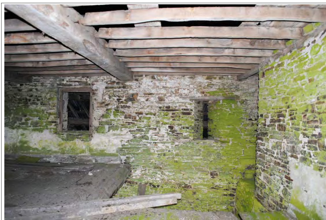
Plate 90. Northern wall of Room 3, showing a ventilation slit and window to the left (west) opening into the adjacent lean-to extension.
