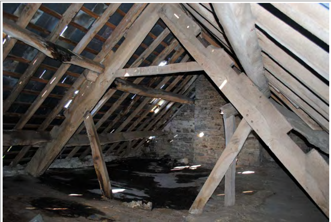
Plate 100. General view of Truss A at the western side of the farmhouse. Looking west-southwest.
