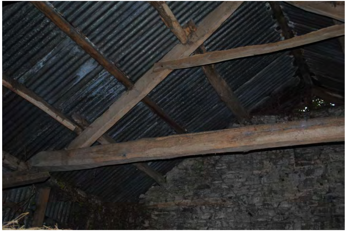
Plate 211. Eastern side of Truss F, with the tie-beam supported by modern timber-framing. Looking south.
