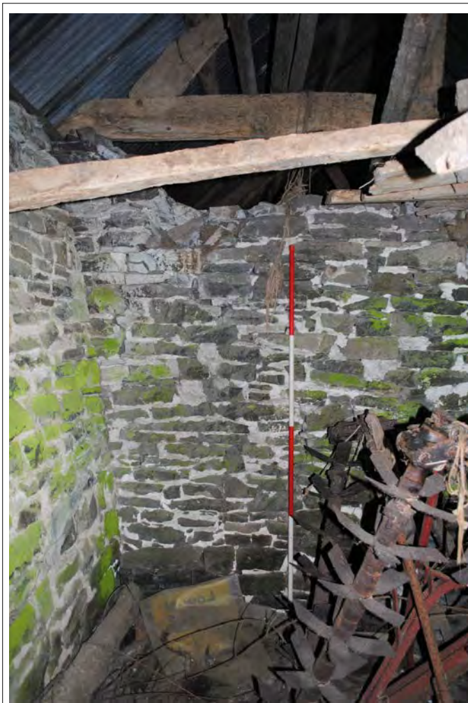
Plate 160. Detail of the western (back) wall and southern (side) wall of the cartshed. Looking south-southwest.
