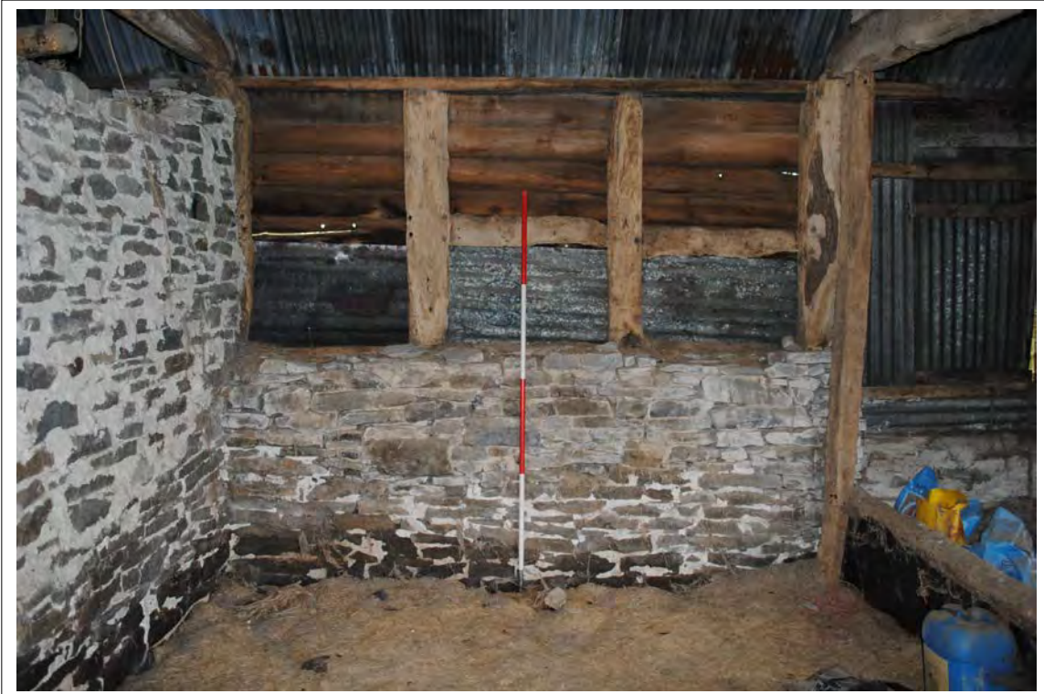
Plate 165. The eastern elevation of Bay C, showing timber-framing over a masonry wall.
