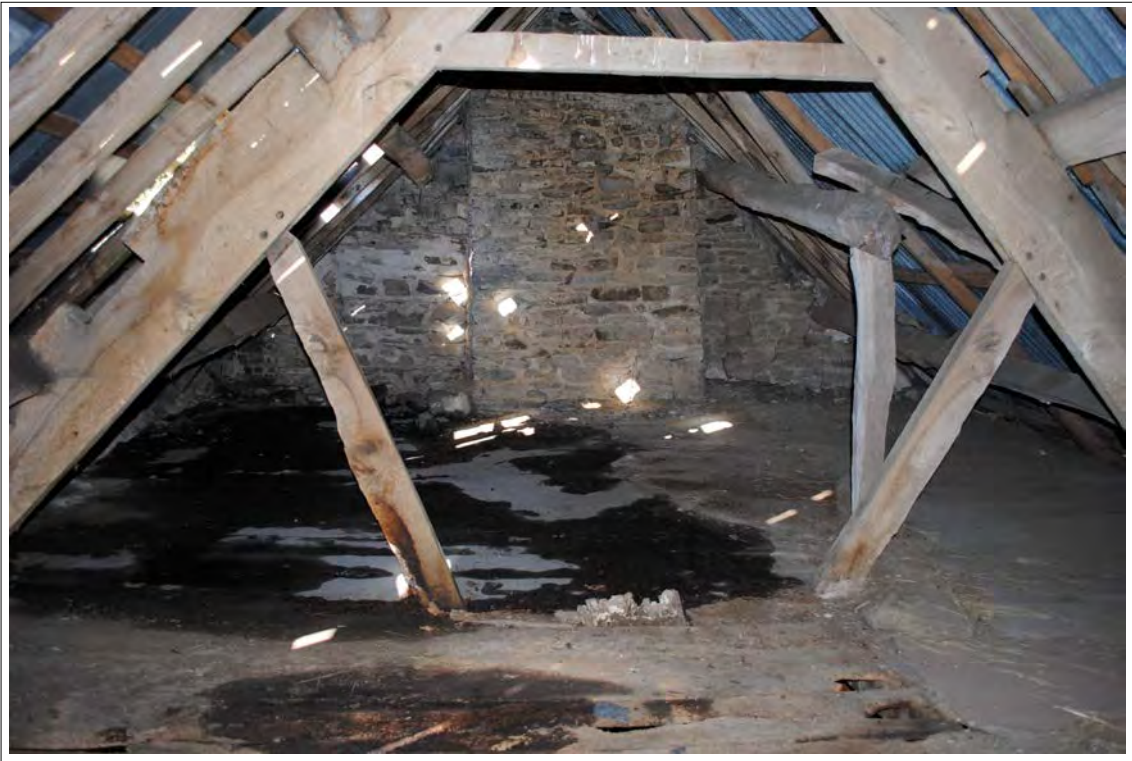
Plate 101. General view of Truss A and the internal face of the of the western gable. Looking west.
