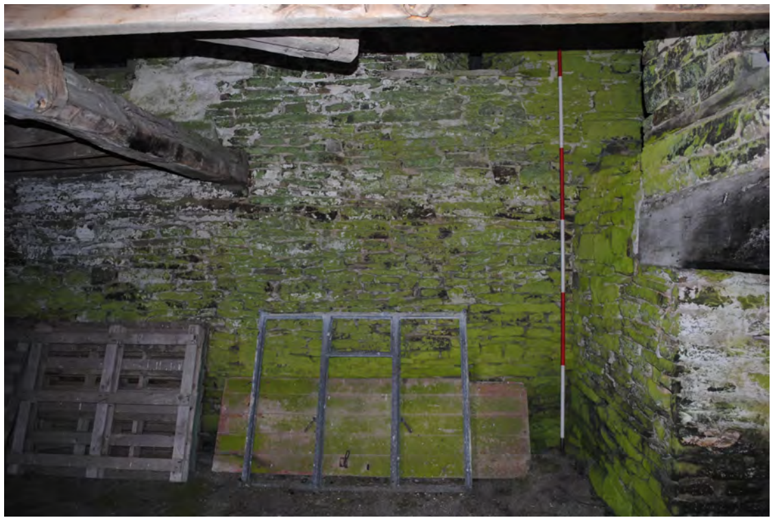
Plate 61. General view of the limewashed northern wall of Room 1, showing missing ceiling.
