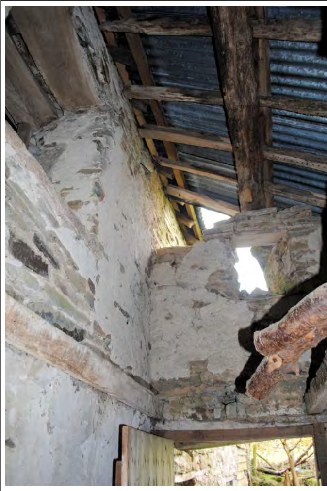
Plate 130. Oblique view of the upper southwest corner of the lean-to, showing a small window below collapsed stonework. Looking west-southwest.
