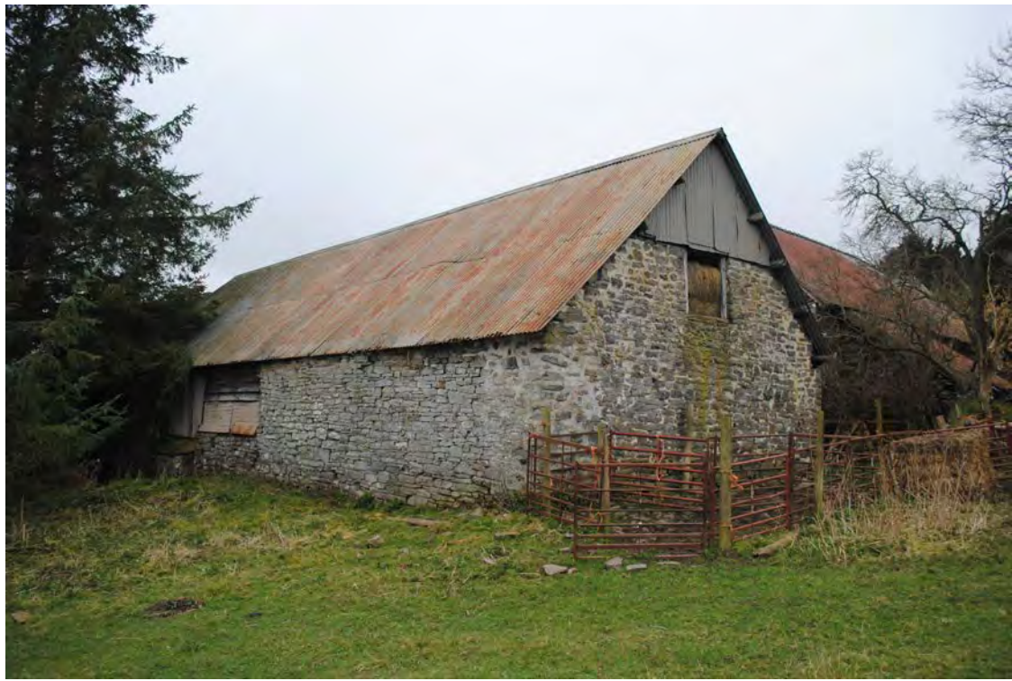
Plate 147. Oblique view of the northern and eastern elevations, showing the rebuilt corner of the stables. Looking west-southwest.
