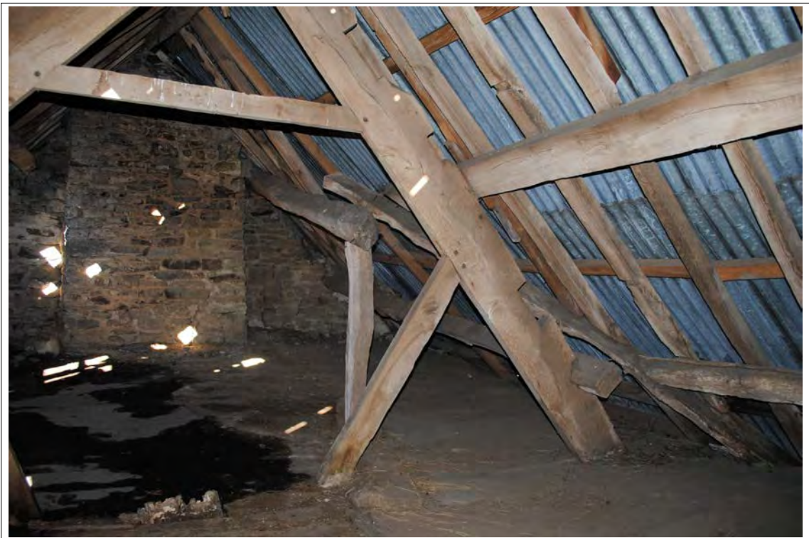
Plate 104. Modified roof timbers on the northern side of Bay A. Looking west.
