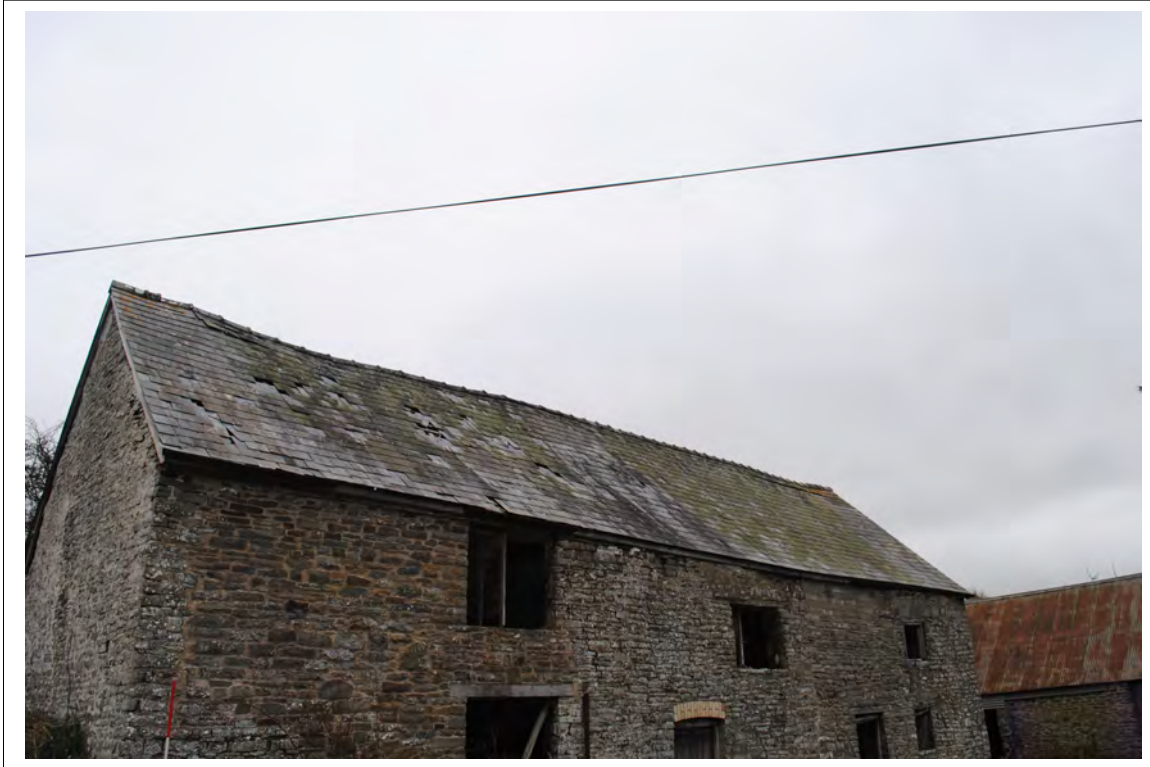
Plate 27. General view of the slate roof on the southern side of the farmhouse. Looking north-northeast.
