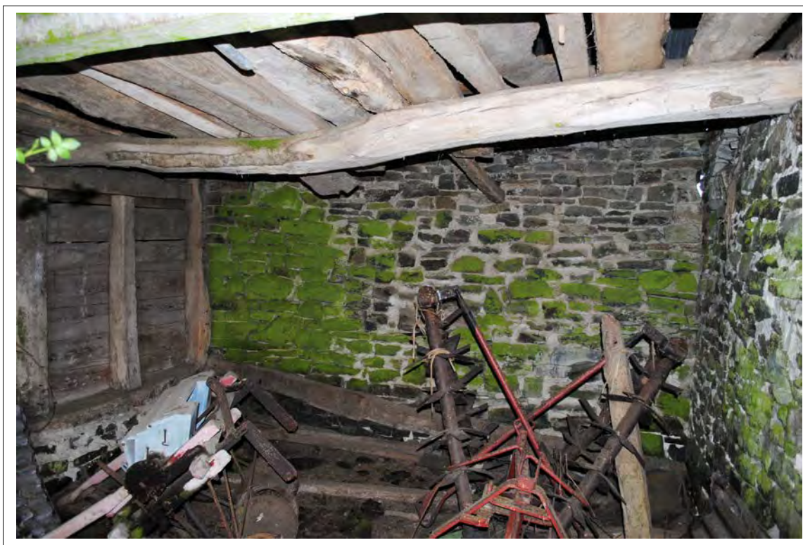
Plate 158. General view of the cartshed, showing timbers for a hayloft above (Bay B). Looking east-southeast.
