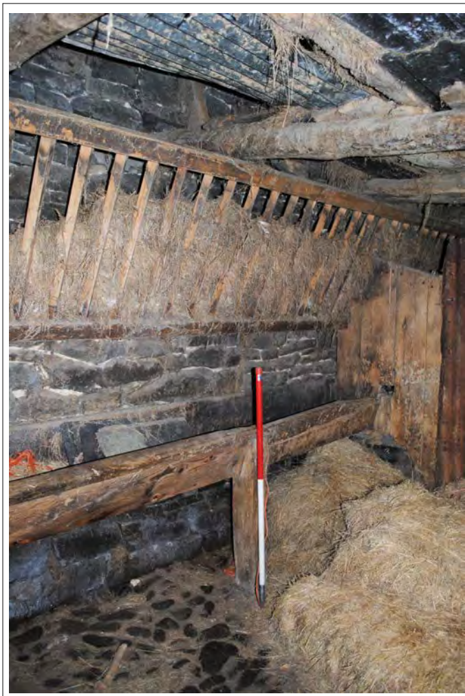
Plate 156. Oblique view of the feeding trough and rack along the northern wall of the stable (Bay A). Looking east.
