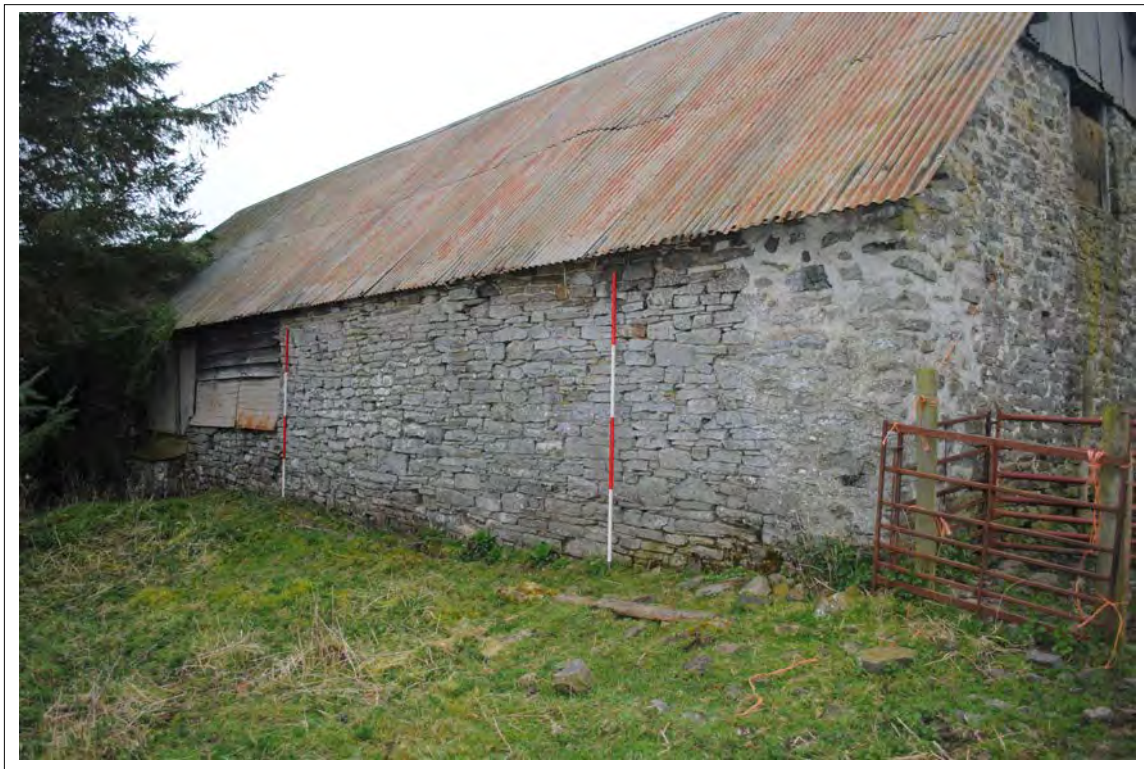
Plate 148. Oblique view of the eastern elevation, showing the back wall of the of the stable and cartshed (Bays A & B). Looking west-southwest.
