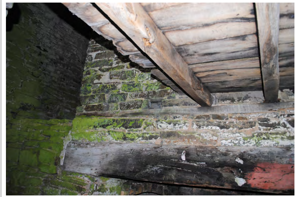
Plate 59. Detail of wall plate and sockets for ceiling joists above bressumer in Room 1.
