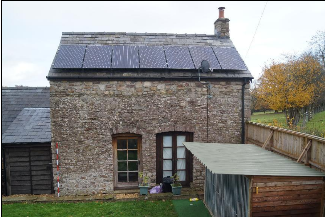
Plate 3: LPT2018_003, A view of the south-southwestern lateral wall of Little Pentre cottage, looking north-northeast. The original doorways are the only features. Note that the wallplate has been raised by over 0.40 metres, presumably during the 20 th century conversion. The roof and chimney are modern therefore.
