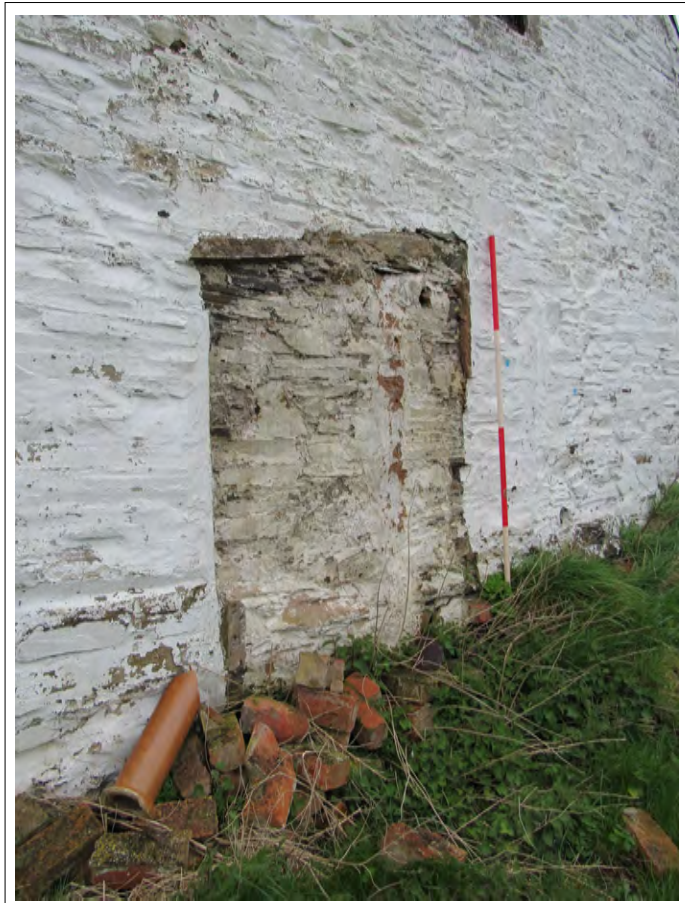
Plate 32. Barn south-west elevation toilet scar. View NE. 2m scale
