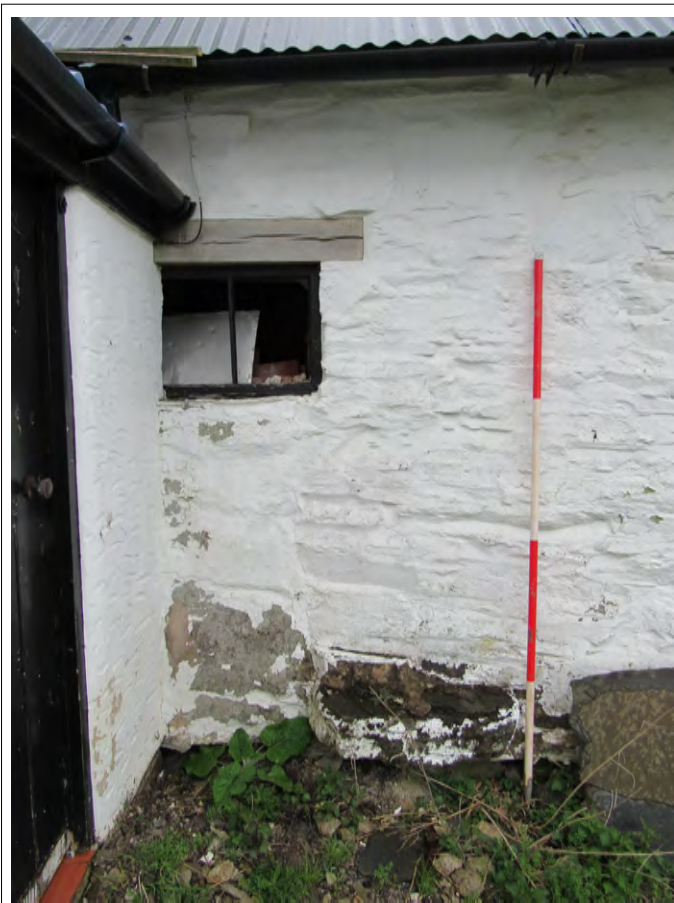
Plate 26. Barn north-west elevation window, original doorway blocked to become window. View SE. 2m scale
