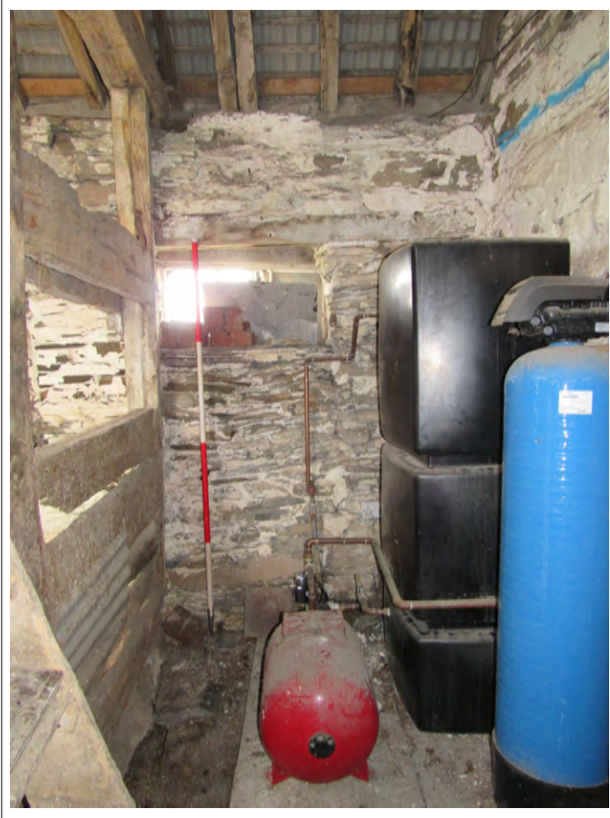
Plate 109. Barn interior blocked doorway in passage on NW wall. View NW. 2m scale
