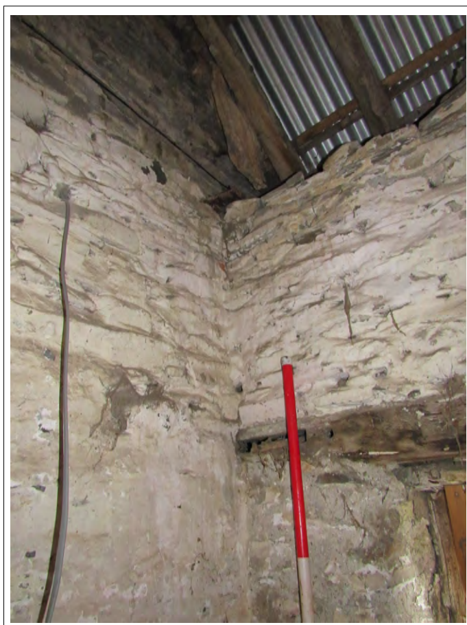
Plate 114. Barn interior, join of barn SE wall and SW wall of house. View E. 2m scale
