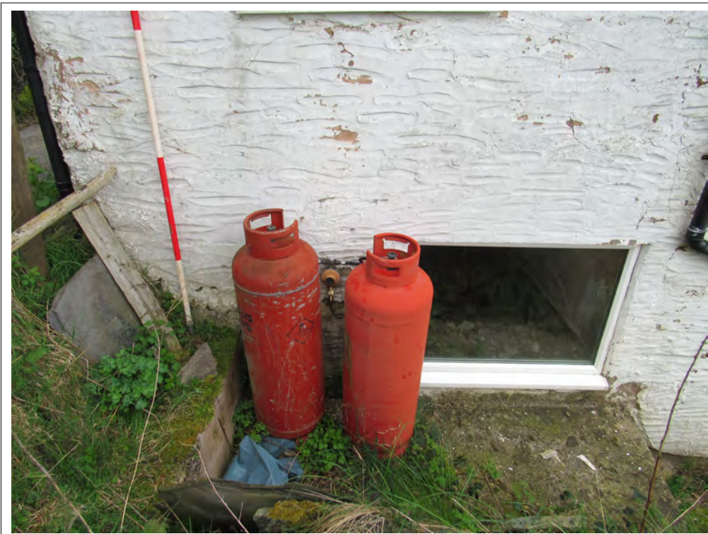
Plate 22. House north-west elevation of later extension ground floor window. View SE. 2m scale
