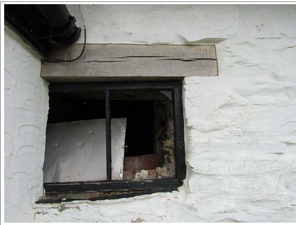
Plate 27. Barn north-west elevation window blocked by porch. View SE.
