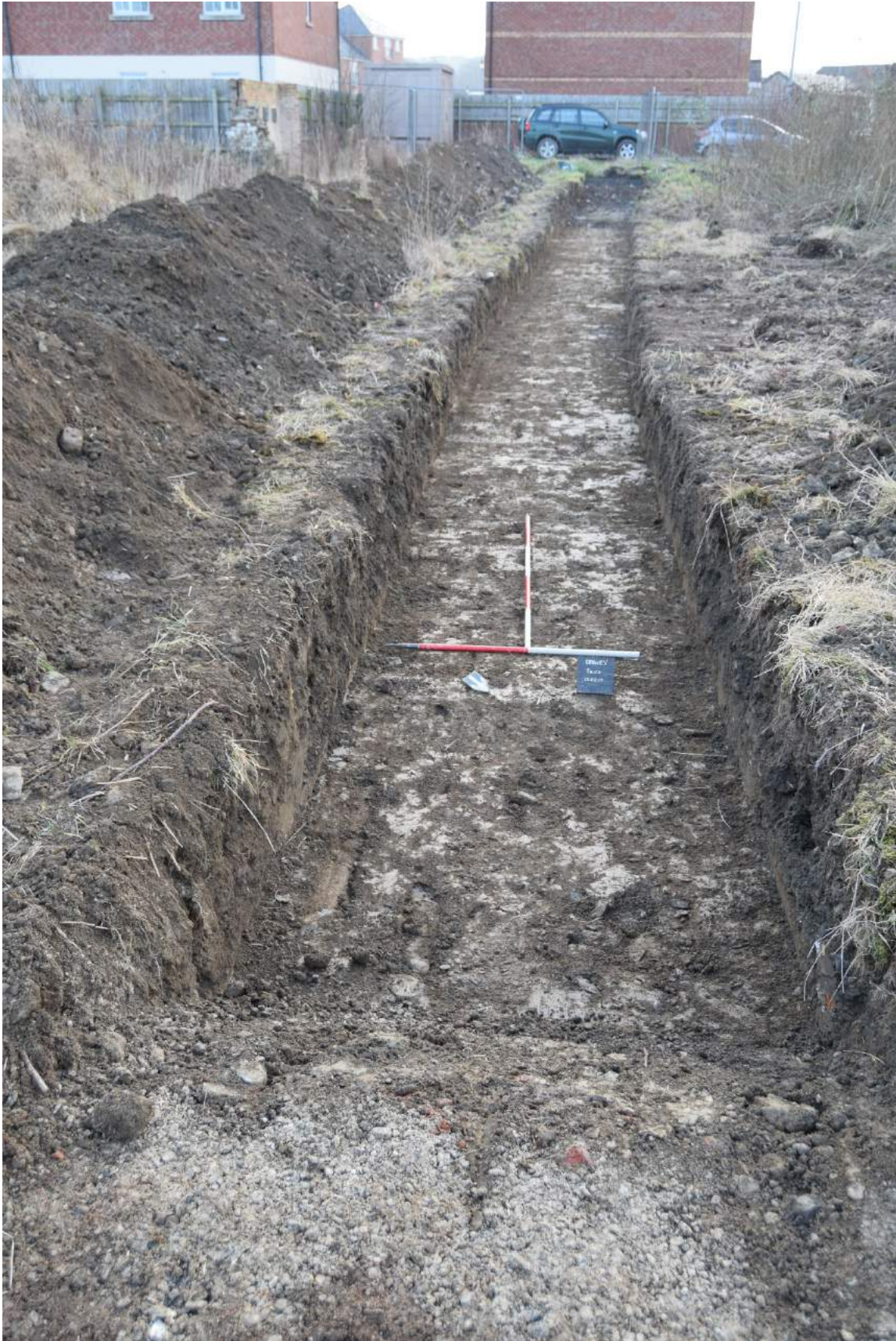
Plate 13: General view of Trench 3, with new flats in the background; shot facing southwest.
