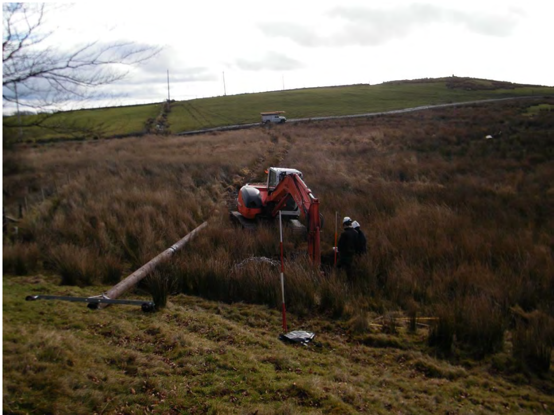
Photo 8: General view looking North from TP C (I) towards TP A. 2m scale.
