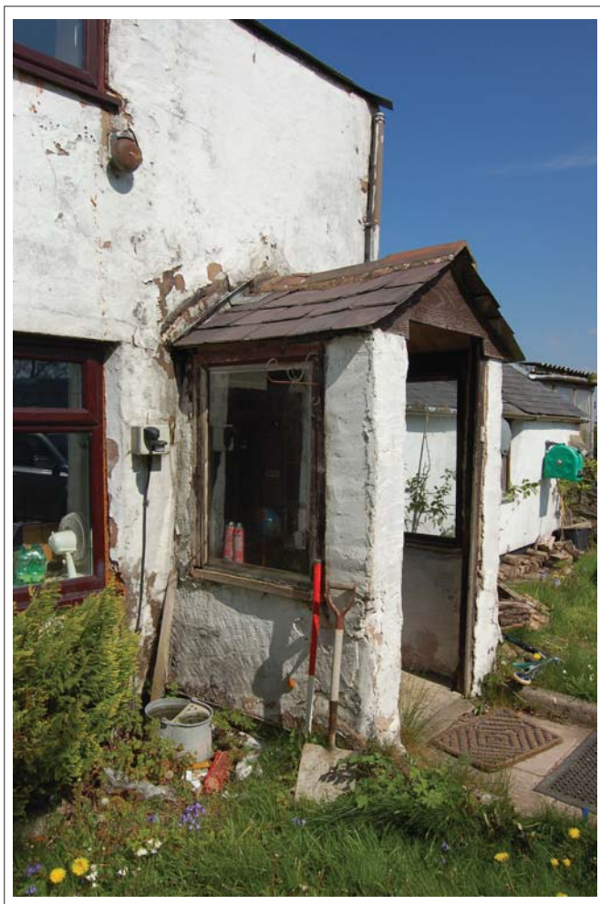
Plate 12. Porch on southern entrance to lounge. Note scar of earlier porch. View northeast. Scale 1m
