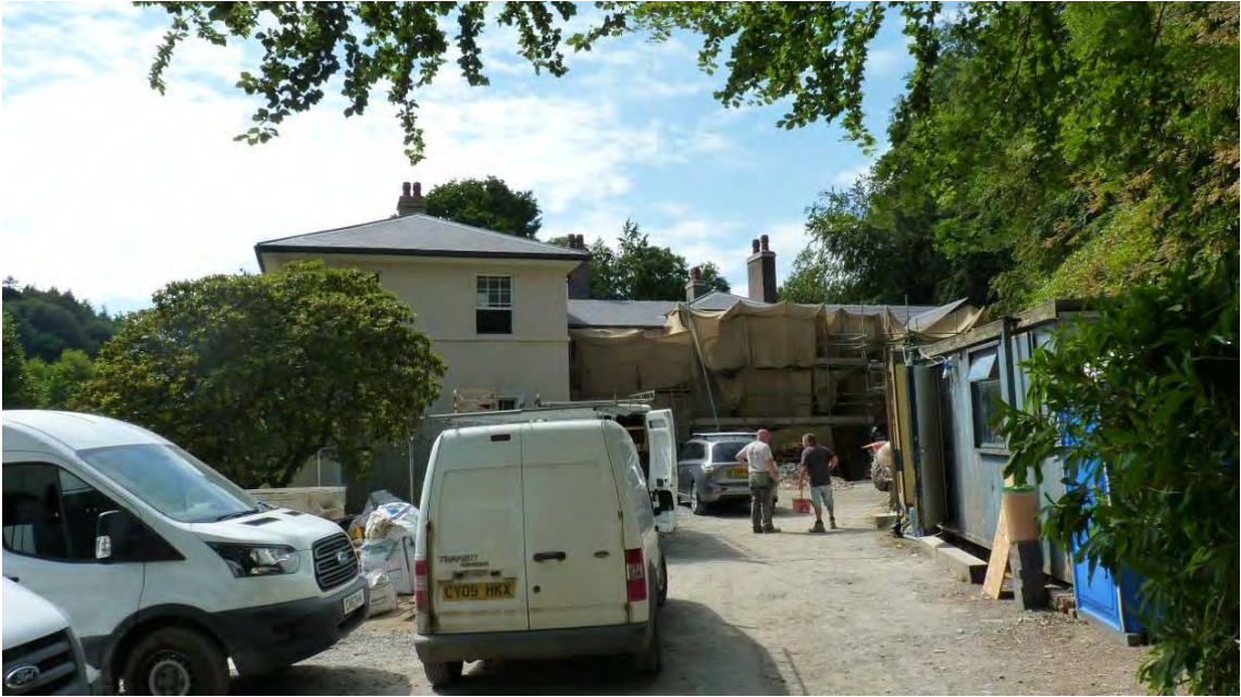
Photo 4: View west of the eastern elevation to Mount Severn, standing on the main approach drive to the house. The house entrance is covered by scaffolding.
