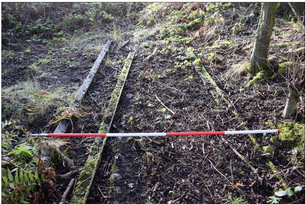
Fig. 15 Displaced tramway rails along a siding approaching the traverser tramway. Photo CPAT 4446-0027
