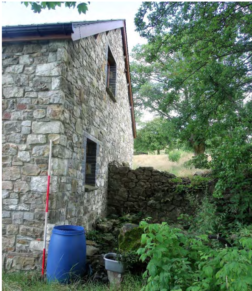
Plate 16: Lean-on structure and East side elevation, view from S; shot facing N. 2m scale.
