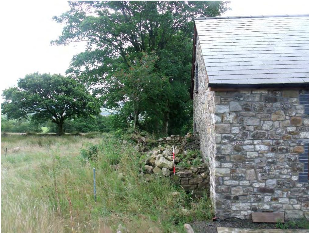
Plate 15: Lean-on structure and East side elevation, view from N; shot facing S. 2m scale.
