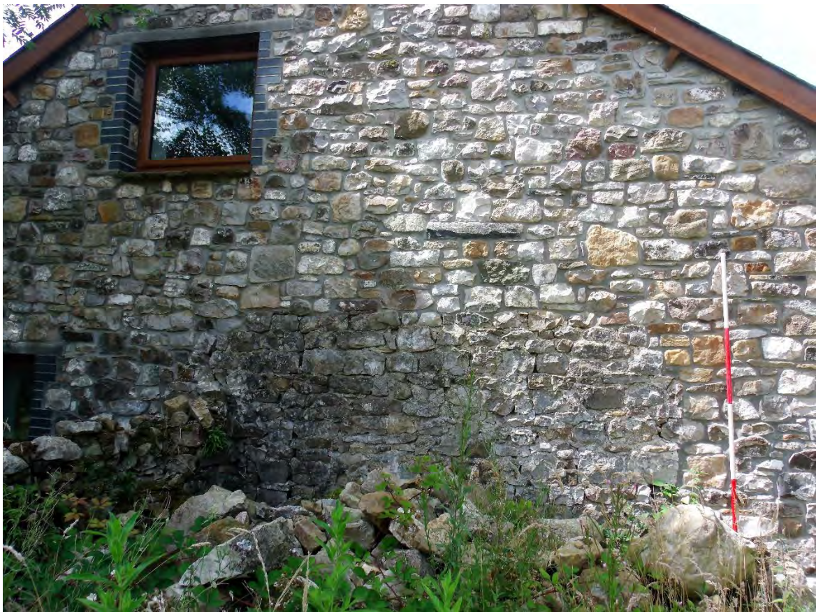
Plate 14: East side elevation, window and original wall detail; shot facing W. 2m scale.
