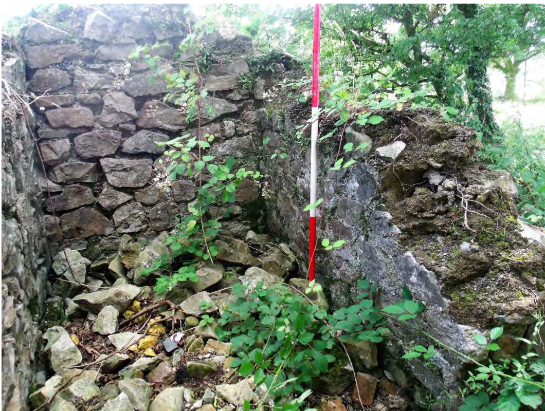
Plate 20: Lean-on structure, detailed view from East side; shot facing E. 2m scale.
