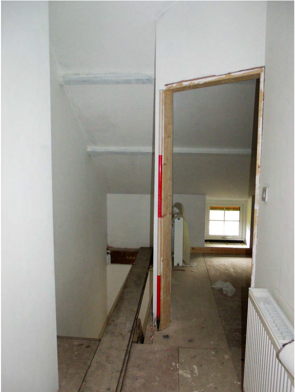
Plate 29: Interior, landing at first floor and entrance of Room 2; view towards N. 2m scale.
