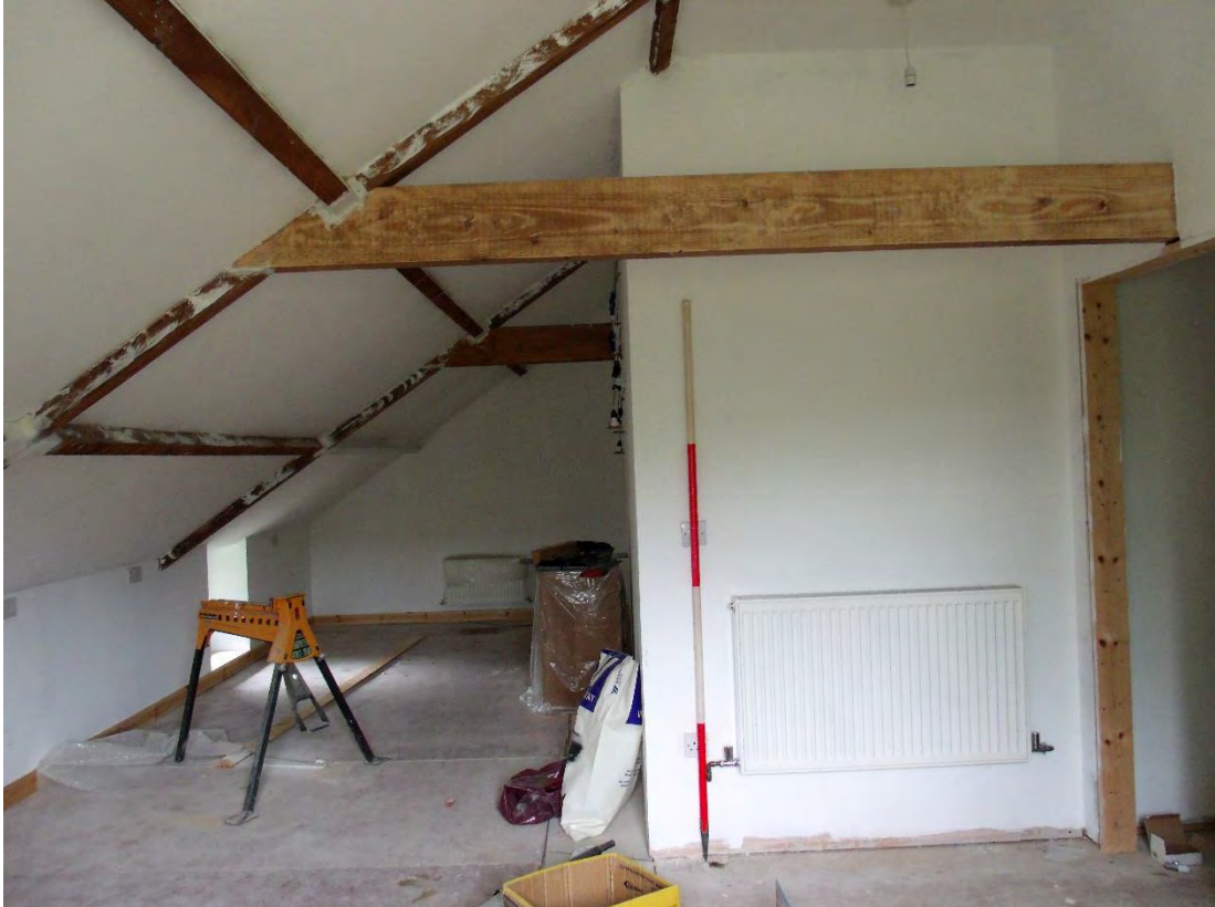
Plate 33: Interior, first floor, Room 1, view of trusses; view towards W. 2m scale.
