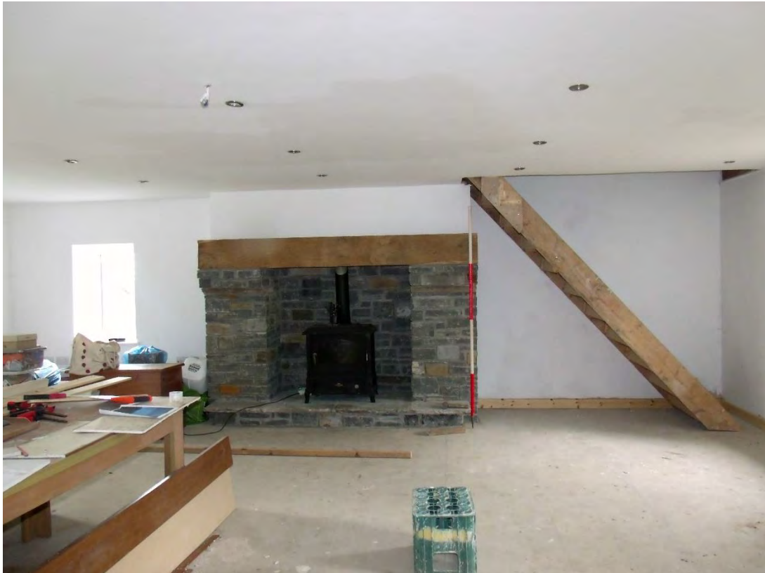
Plate 25: Interior, ground floor; view towards W with fire place and temporary staircase. 2m scale.
