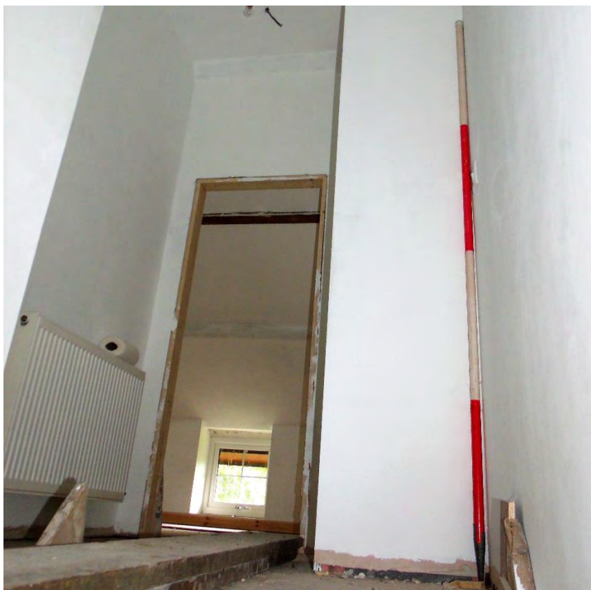
Plate 28: Interior, landing at first floor and entrance of Room 1; view towards S. 2m scale.
