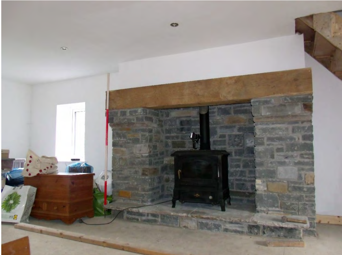
Plate 24: Interior, ground floor; view towards SW with rebuilt fire place in original location. 2m scale.
