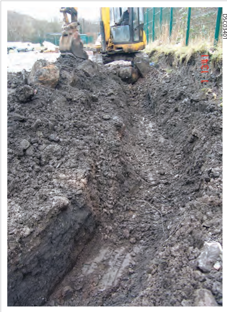
Plate 05: Overview of TR3, southern end, Cut line on left side of trench
