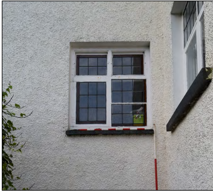
Plate 7: NE Facing Elevation of the Stair Hall, looking south west, 2m & 1m scale.
