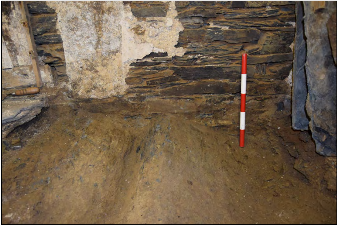
Plate 25: Basement, Test Pit 1 detail of NE facing wall, looking south-west, 0.5m scale.
