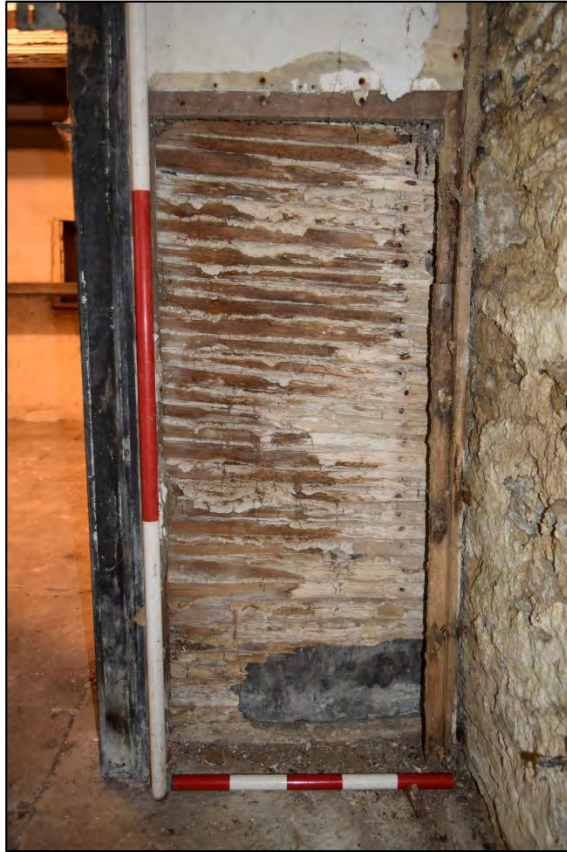
Plate 13: Basement corridor, lath and lime plaster partition wall looking south west, 2m & 0.5m scale.
