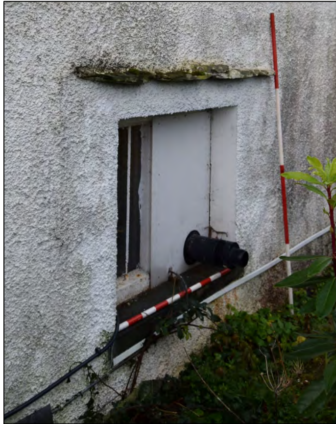
Plate 5: NE Facing Elevation, basement window. looking north north- west, 2m & 1m scale.
