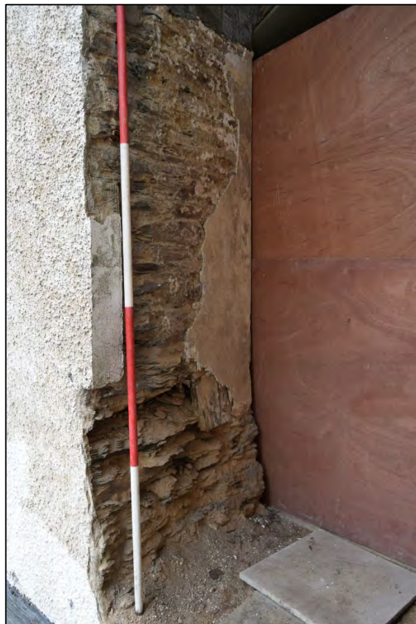
Plate 22: Stair Hall, first floor, new doorway opening, looking south south-west, 2m scale.
