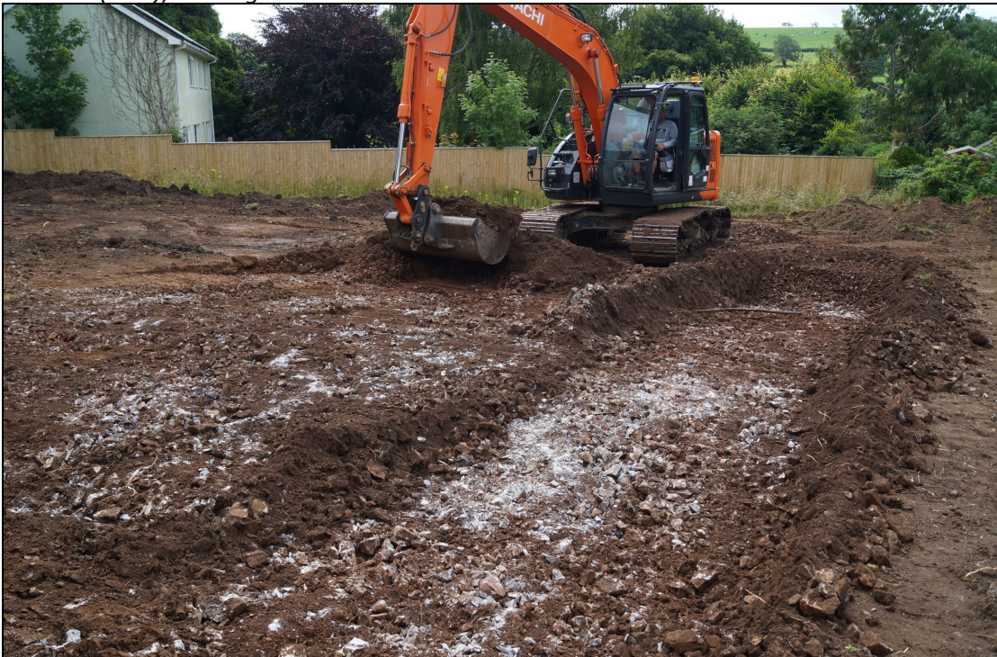
Plate 8: STF2020_108. A view of the bedrock (003) after stripping of (001) and (002) looking southeast.
