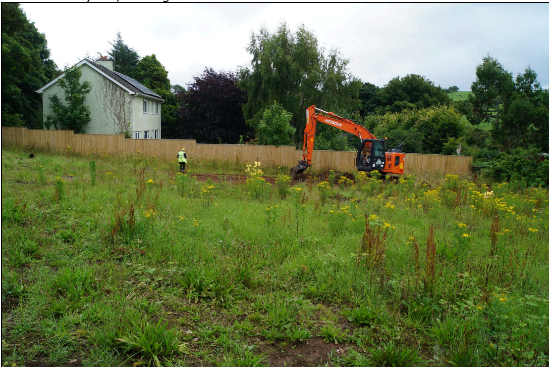
Plate 2: STF2020_102. General view of the development area looking at Tynewydd beyond, built in the mid 20 th century, looking south-southeast.
