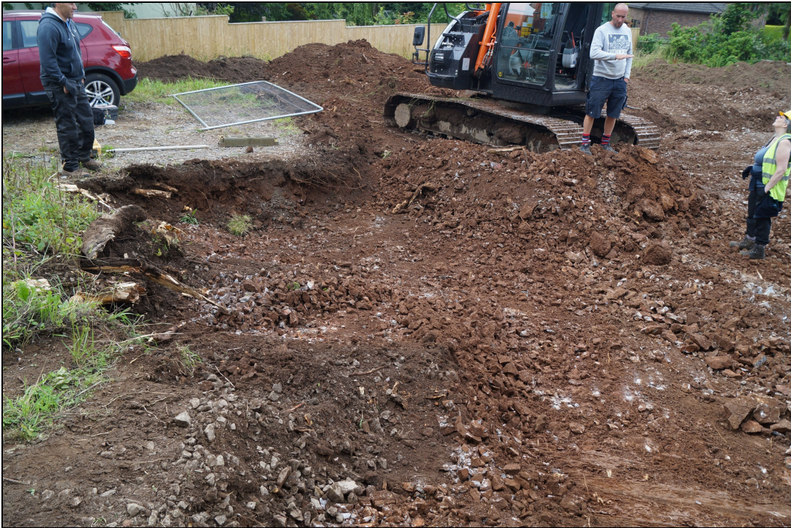
Plate 5: STF2020_105. A view of the site after removing of top soil (001), showing the subsoil (002) and bedrock (003), looking south-southwest.
