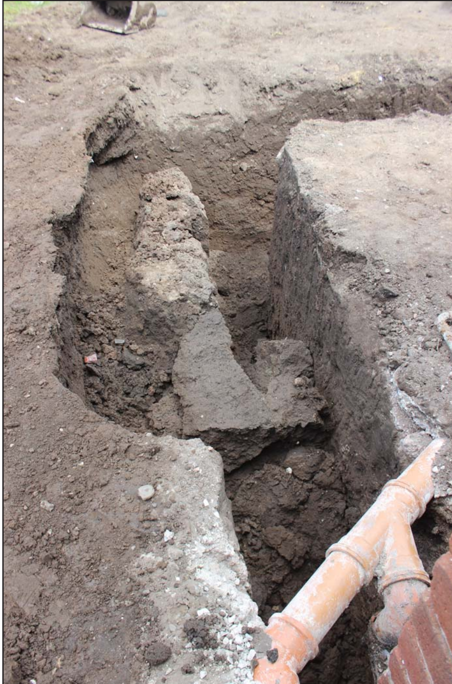
Plate 08: Collapse in northern footing - from the southwest - no scale
