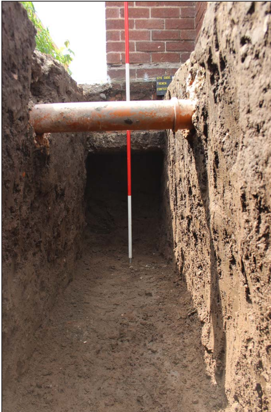
Plate 04: Shot of southern footing (from within trench) - from the northeast - scale 2.00m
