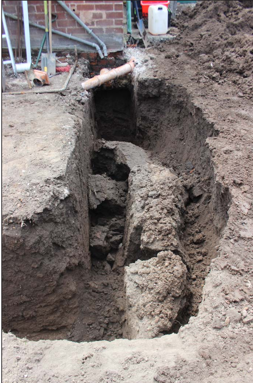
Plate 07: Collapse in northern footing - from the northeast - no scale
