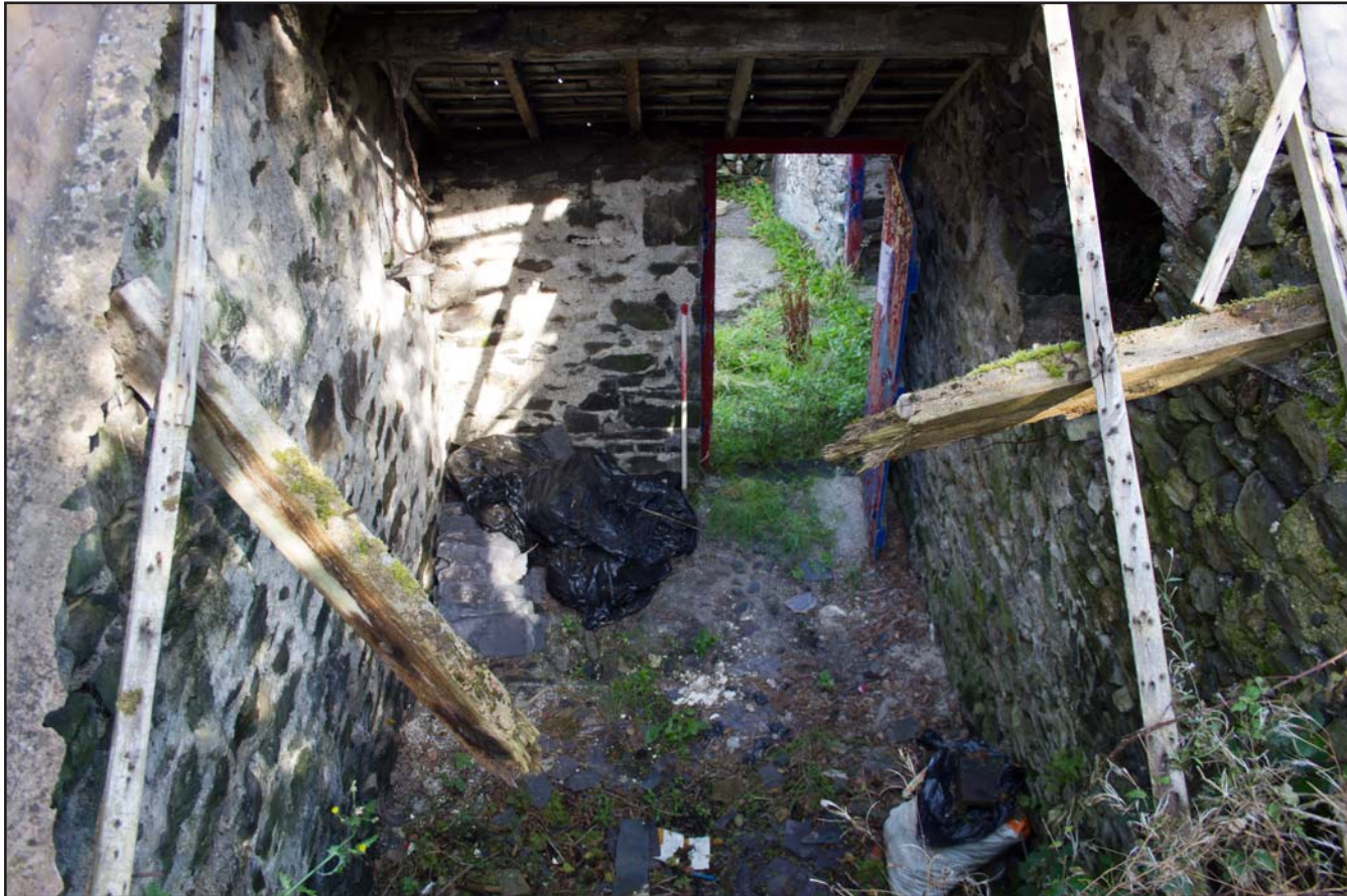
Plate 21: Internal shot - Southern elevation of Store 1, Tan Y Bodran, Bodran Road, Llanfairtalhaiarn, Conwy - from the north - no scale
