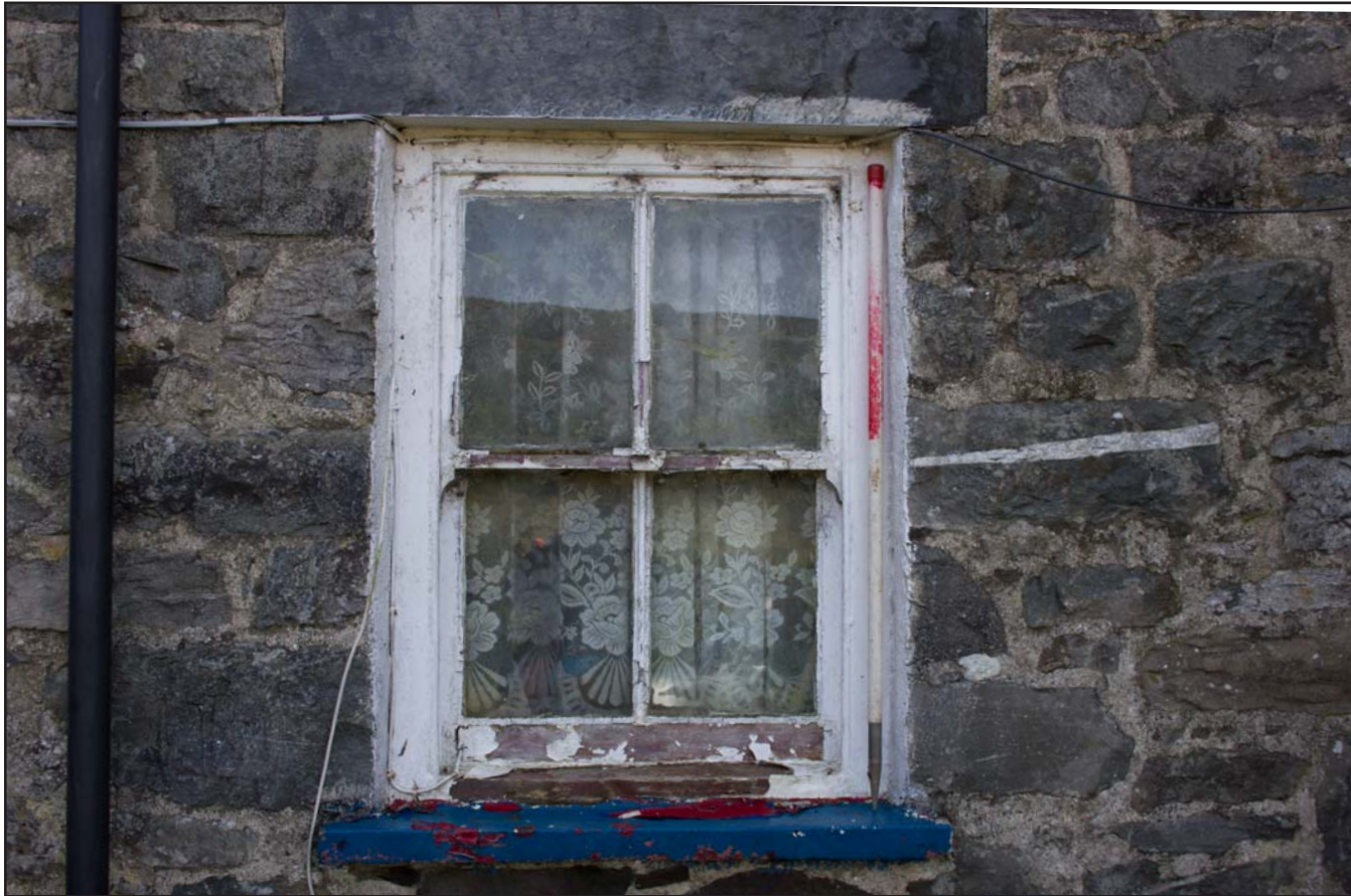
Plate 18: External shot - Ground floor window on northern elevation of the Farmhouse, Tan Y Bodran, Bodran Road, Llanfairtalhaiarn, Conwy - from the north - scale 1m
