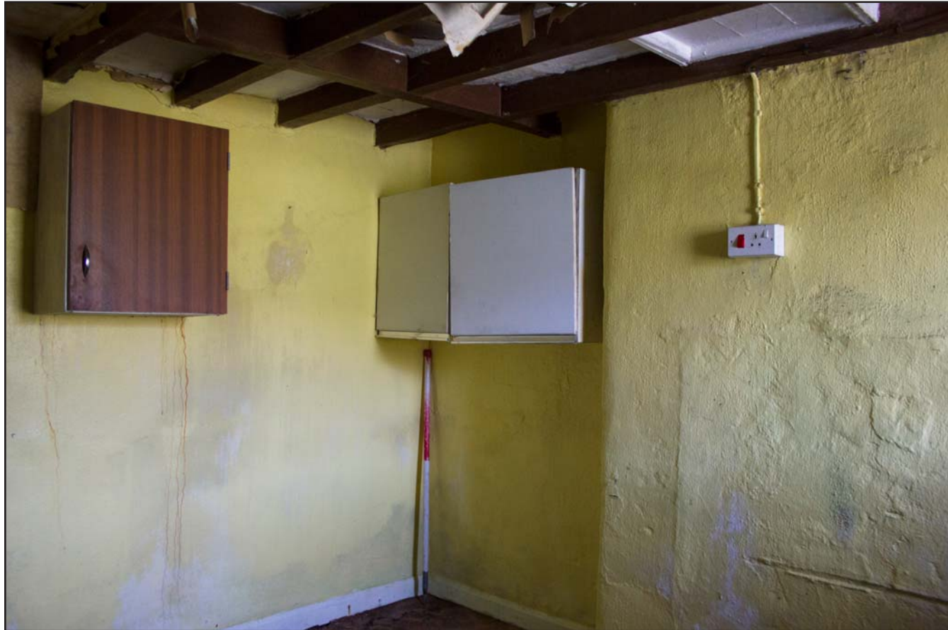
Plate 29: Internal shot - Kitchen within the Farmhouse building at Tan Y Bodran, Bodran Road, Llanfairtalhaiarn, Conwy - from the northeast - scale 1m
