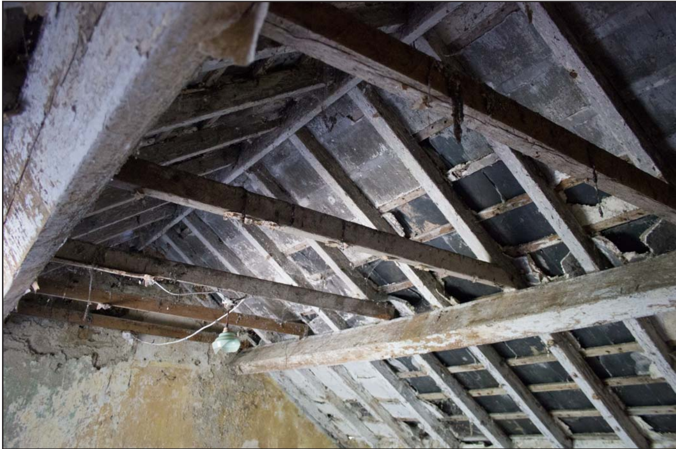
Plate 34: Internal shot - Bedroom 1 ceiling, within the Farmhouse building at Tan Y Bodran, Bodran Road, Llanfairtalhaiarn, Conwy - from the northwest - no scale
