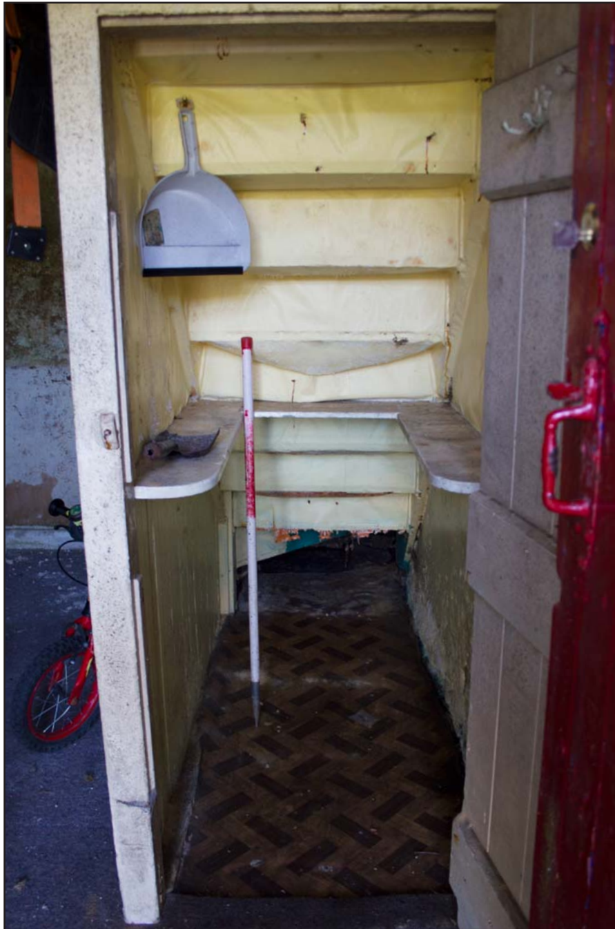
Plate 31: Internal shot - "Twill dan Stair" beneath stairwell within the Farmhouse building at Tan Y Bodran, Bodran Road, Llanfairtalhaiarn, Conwy - from the north - scale 1m
