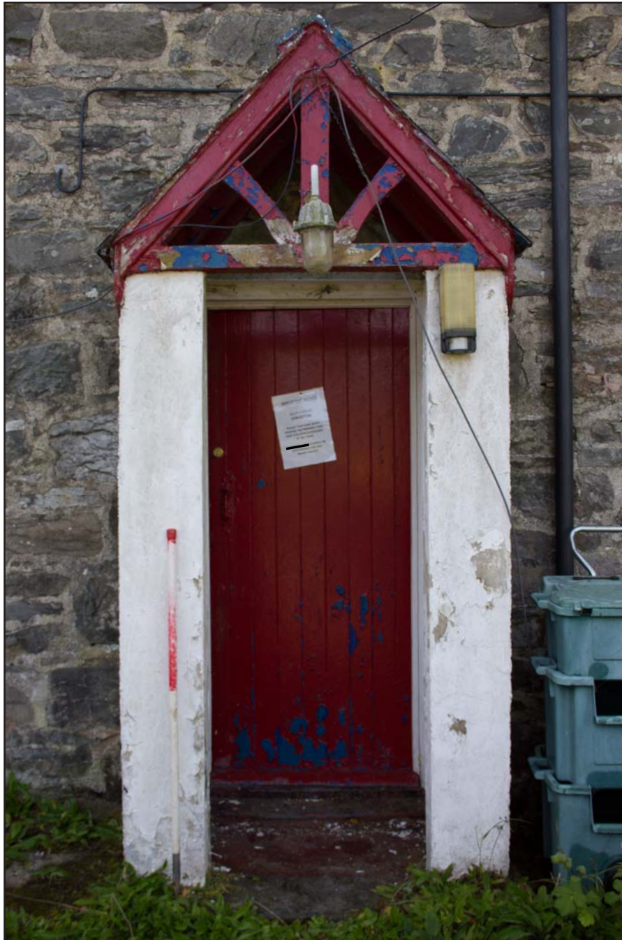
Plate 17: External shot - Porch on northern elevation of the Farmhouse, Tan Y Bodran, Bodran Road, Llanfairtalhaiarn, Conwy - from the north - scale 1m
