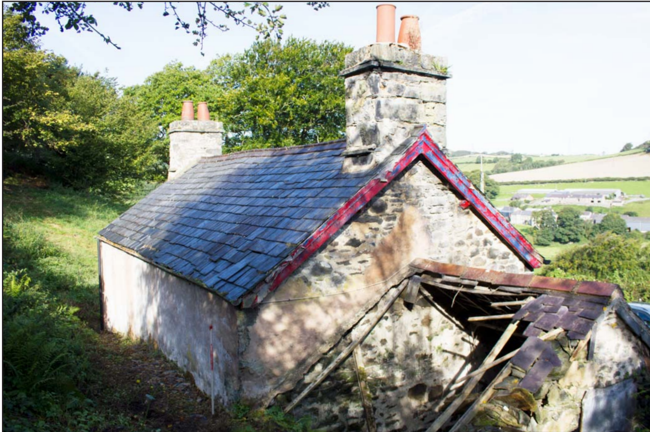
Plate 07: External shot - southern and eastern elevations of the Farmhouse, Tan Y Bodran, Bodran Road, Llanfairtalhaiarn, Conwy - from the southeast - scale 1m
