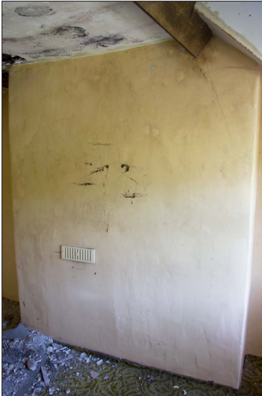
Plate 36: Internal shot - Bedroom 2, within the Farmhouse building at Tan Y Bodran, Bodran Road, Llanfairtalhaiarn, Conwy - from the northeast - no scale
