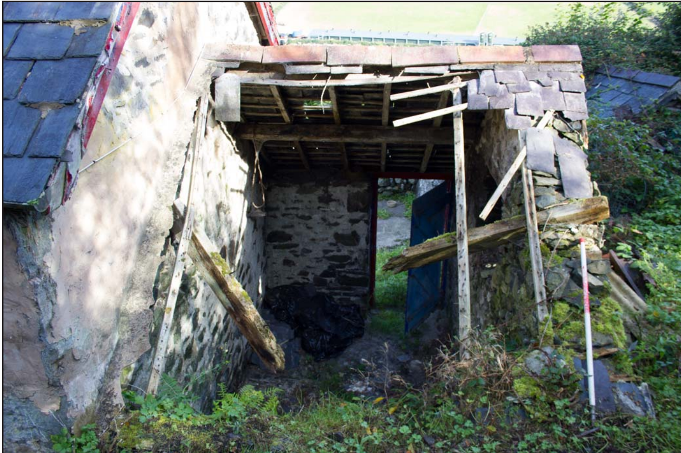
Plate 09: External shot - southern elevation of Store 1, Tan Y Bodran, Bodran Road, Llanfairtalhaiarn, Conwy - from the south - scale 1m
