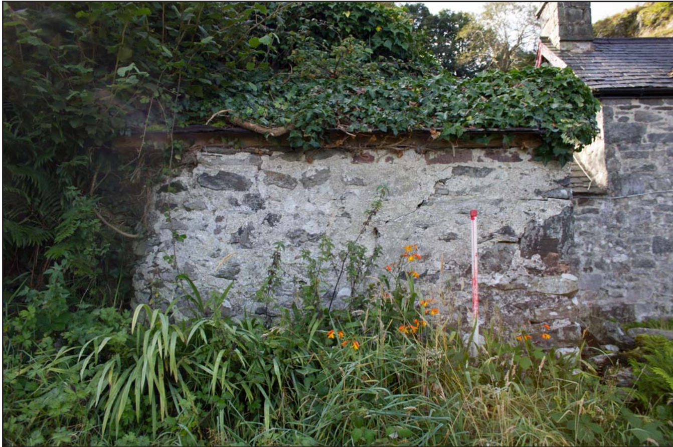
Plate 12: External shot - northern elevation of Store 2, Tan Y Bodran, Bodran Road, Llanfairtalhaiarn, Conwy - from the northeast - scale 1m
