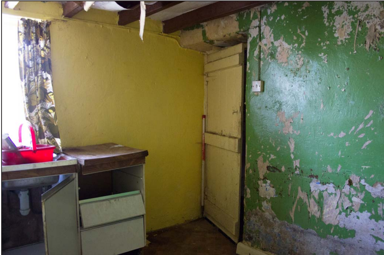
Plate 30: Internal shot - Kitchen within the Farmhouse building at Tan Y Bodran, Bodran Road, Llanfairtalhaiarn, Conwy - from the southeast - scale 1m
