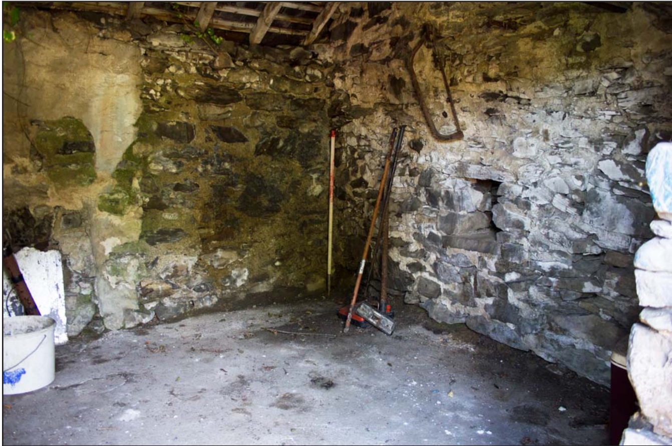
Plate 22: Internal shot - Oblique shot of Store 2, Tan Y Bodran, Bodran Road, Llanfairtalhaiarn, Conwy - from the southwest - scale 1m
