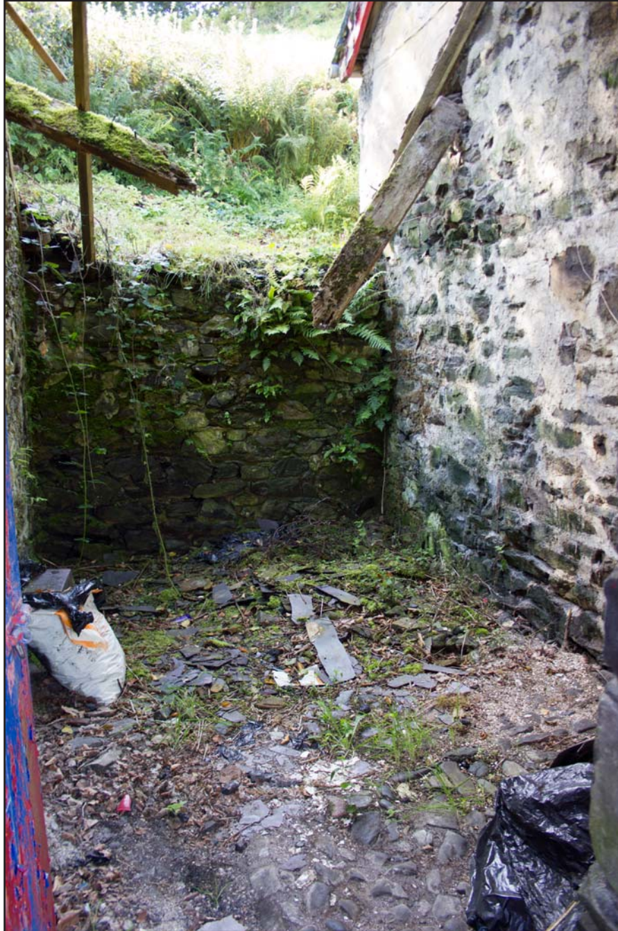
Plate 20: Internal shot - Floor and northern elevation of Store 1, Tan Y Bodran, Bodran Road, Llanfairtalhaiarn, Conwy - from the south - scale 1m
