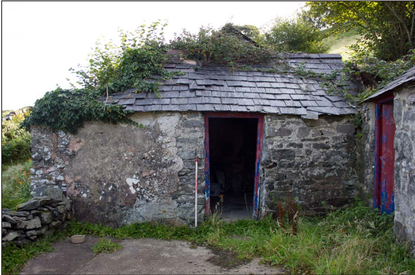
Plate 14: External shot - western elevation of Store 2, Tan Y Bodran, Bodran Road, Llanfairtalhaiarn, Conwy - from the west - scale 1m
