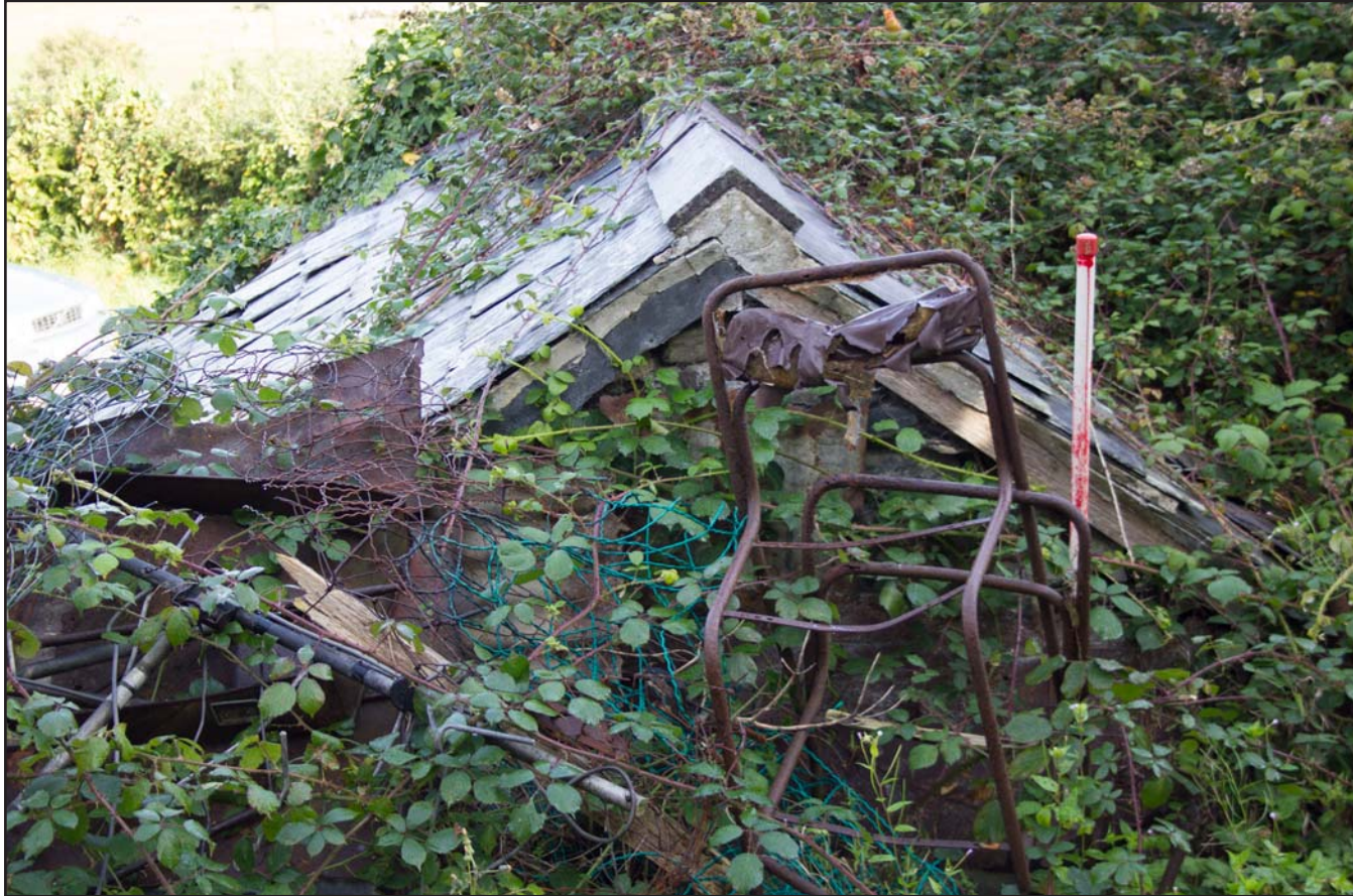
Plate 15: External shot - southern elevation of Store 2, Tan Y Bodran, Bodran Road, Llanfairtalhaiarn, Conwy - from the south - scale 1m
