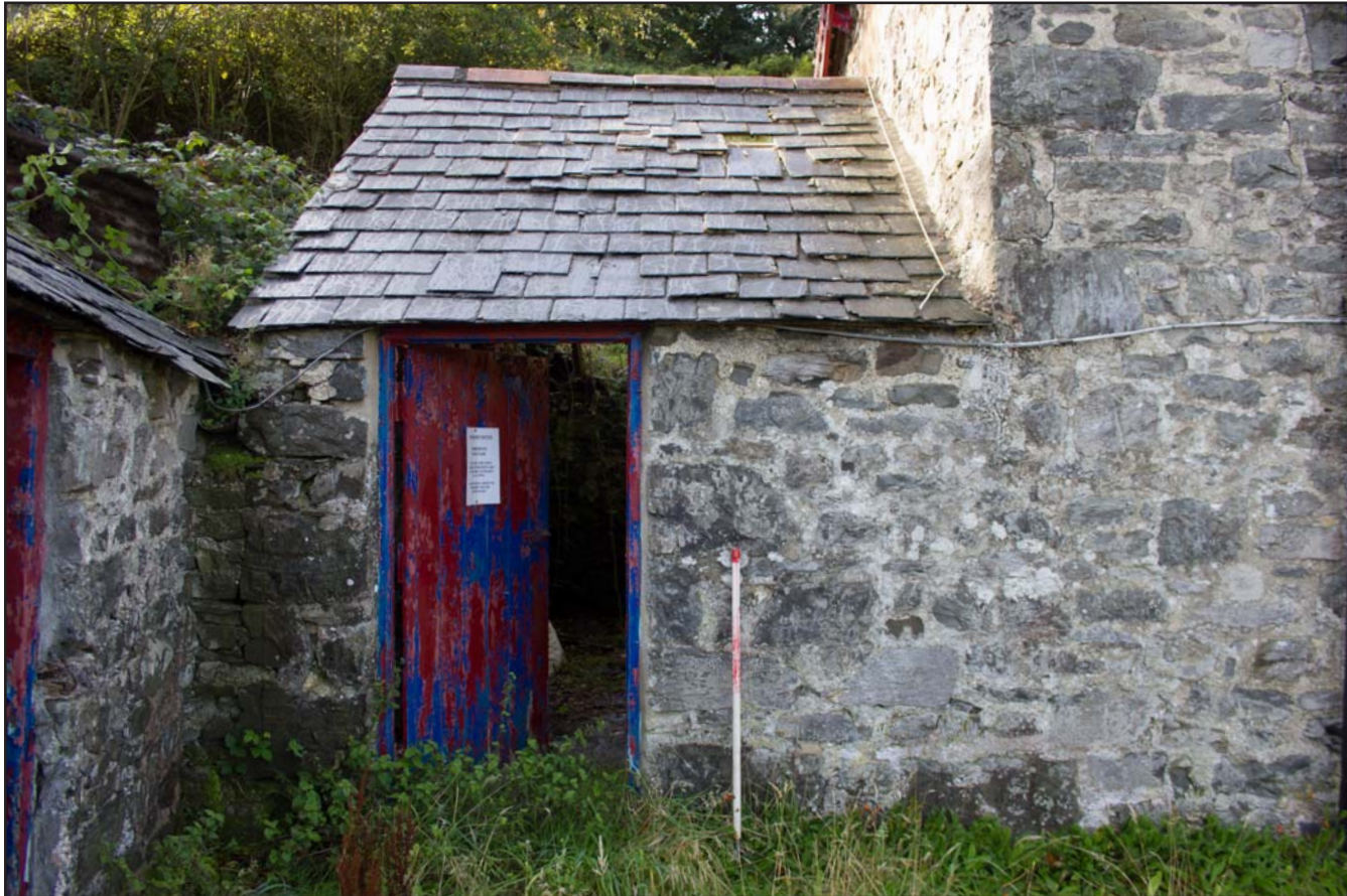
Plate 10: External shot - northern elevation of Store 1, Tan Y Bodran, Bodran Road, Llanfairtalhaiarn, Conwy - from the north - scale 1m
