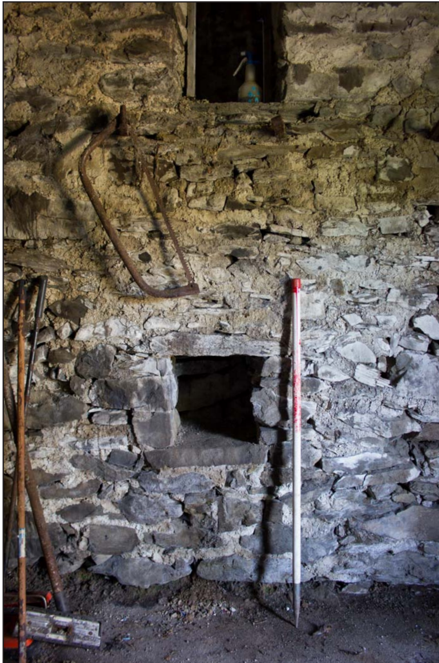
Plate 24: Internal shot - Southern elevation in Store 2, Tan Y Bodran, Bodran Road, Llanfairtalhaiarn, Conwy - from the southwest - scale 1m
