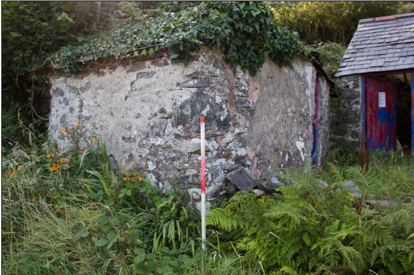
Plate 13: External shot - northern and western elevations of Store 2, Tan Y Bodran, Bodran Road, Llanfairtalhaiarn, Conwy - from the northwest - scale 1m
