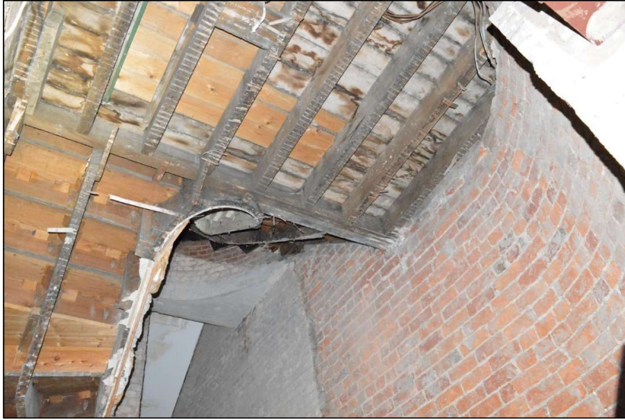
Fig 53: Timbers of the east stair looking up from the ground floor to the first floor landing (CPAT 4853-0052)
