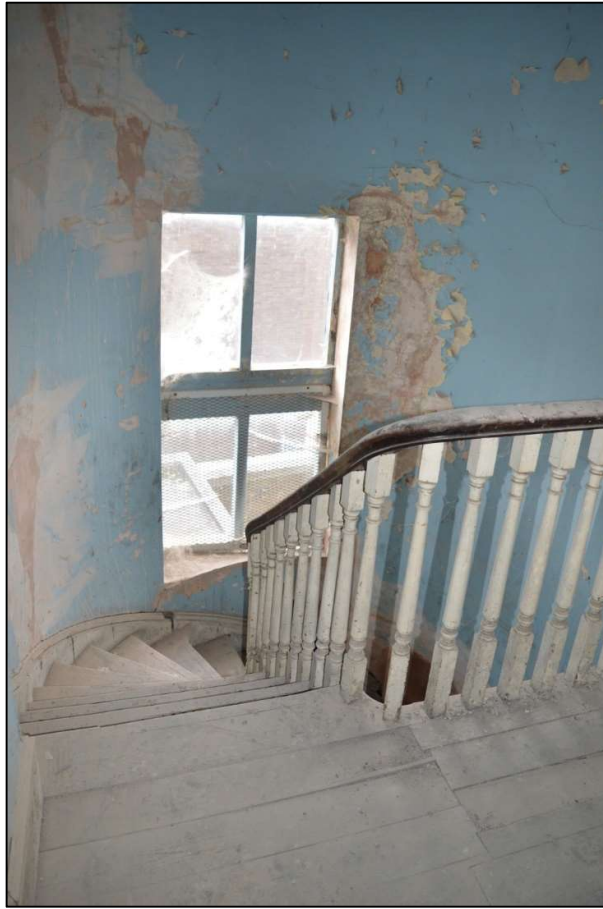
Fig 57: View looking down the east stair from the second floor landing (CPAT 4853-0056)
