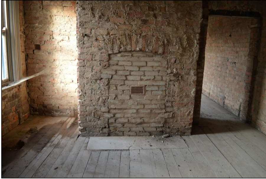
Fig 10: Blocked fireplace with hearth stone in Room 2 on second floor. Also shows wall cracks (CPAT 4853-0009)
