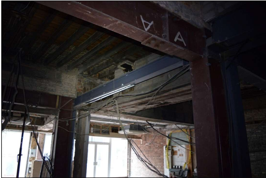
Fig 51: The inserted steelwork supporting the centre of the building from below. Also shows the surviving upper part of the south wall of the original building (to left) and the beams supporting the southern of the two chimney stacks (CPAT 4853-0050)
