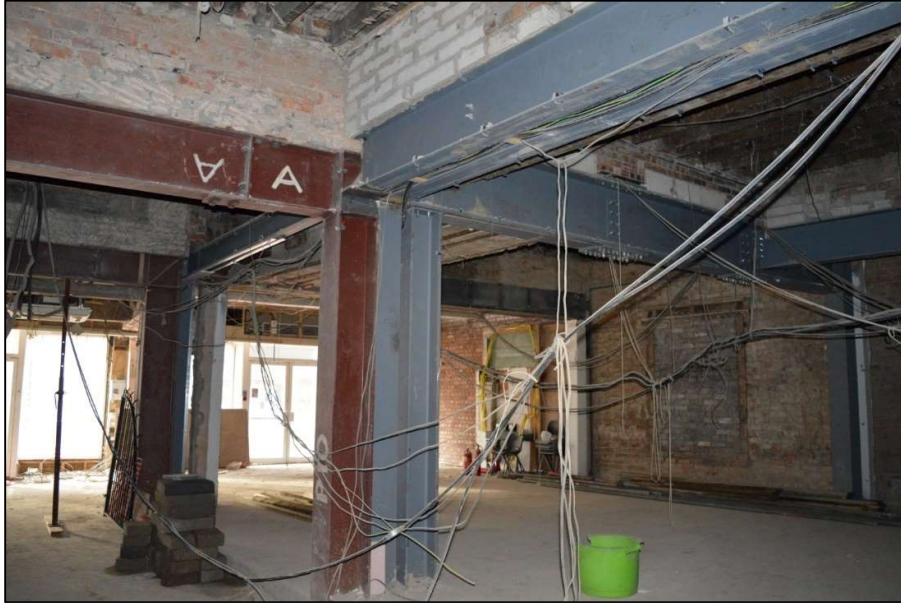
Fig 55: The inserted steelwork supporting the centre of the building from below. Also shows the surviving upper part of the east/west cross wall (to left) on the ground floor (CPAT 4853-0054)
