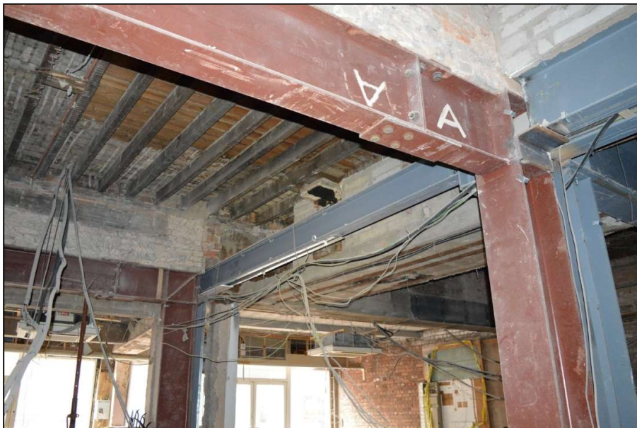
Fig 52: As 51. The inserted steelwork supporting the centre of the building from below. Also shows the surviving upper part of the ground floor south wall of the original building (to left) and the beams supporting the southern of the two chimney stacks (CPAT 4853-0051)
