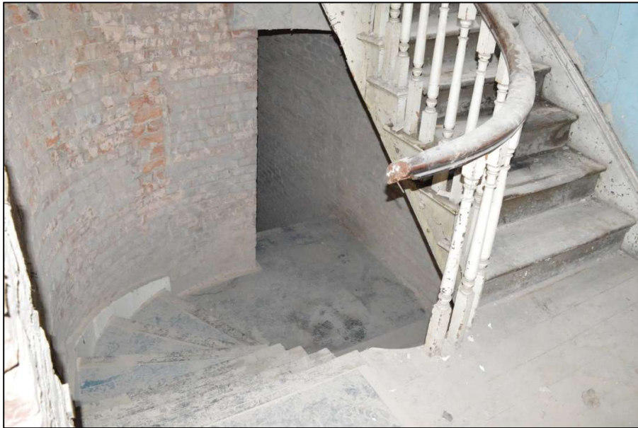
Fig 68: Looking down the east stair from the first floor landing. Shows where the east stair was truncated by the modern insertion of steps down (centre) to the rear of the building (CPAT 4853-0066)
