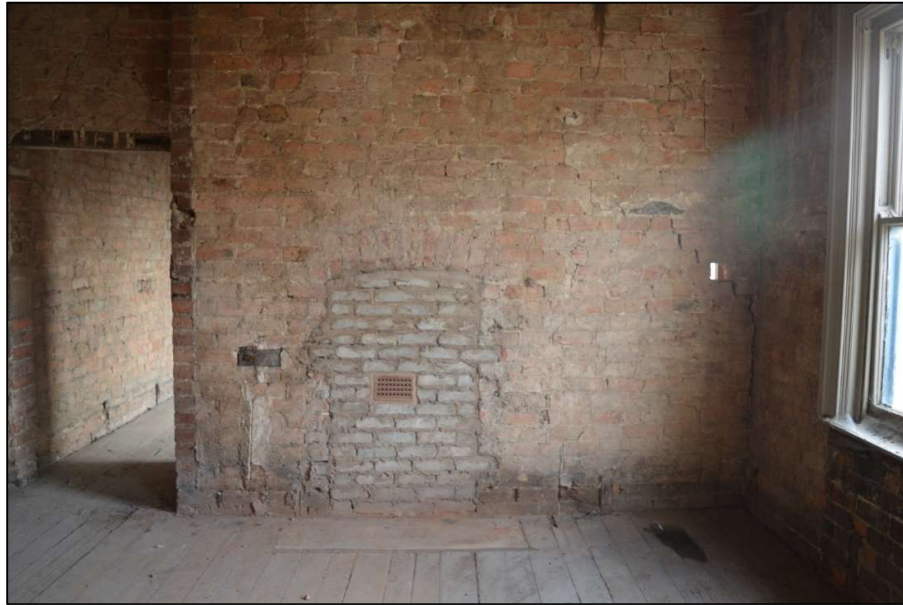
Fig 12: Blocked fireplace with hearth stone in Room 3 on second floor. Also shows wall cracks (CPAT 4853-0011)
