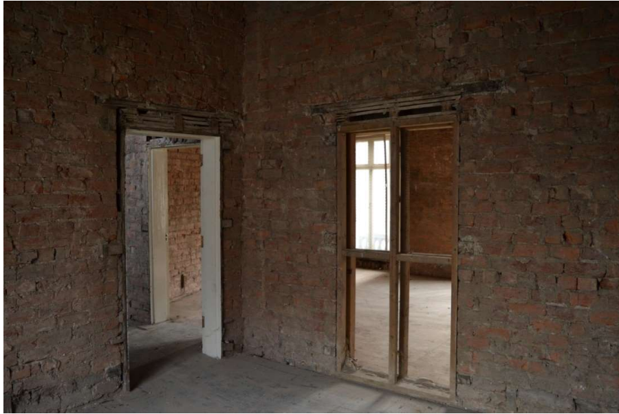
Fig 34: Blocked doorway in Room 5 on first floor (to right). Also shows doorway to east stair (CPAT 4853-0033)
