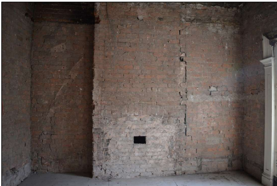
Fig 25: Blocked fireplace in Room 7 on first floor. Also shows wall cracks (CPAT 4853-0024)
