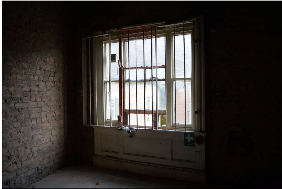
Fig 28: Window in Room 8 on first floor. (CPAT 4853-0027)
