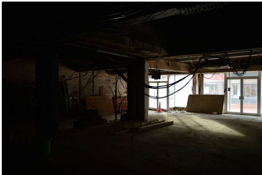
Fig 46: General view of ground floor (CPAT 4853-0045)
