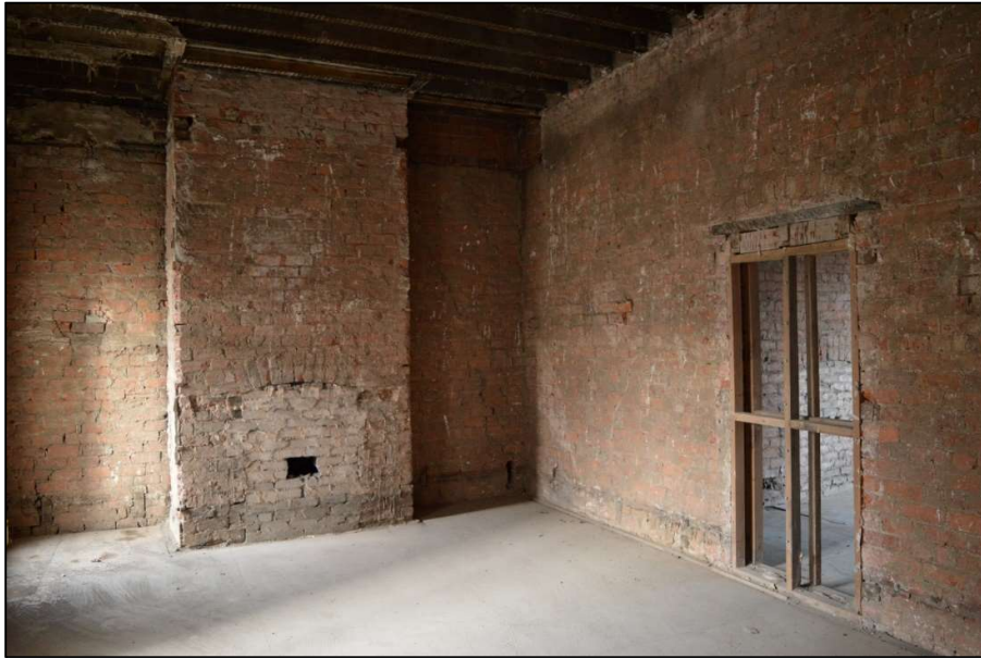
Fig 39: Blocked fireplace and door in Room 6 on first floor. Also shows wall cracks (CPAT 4853-0038)
