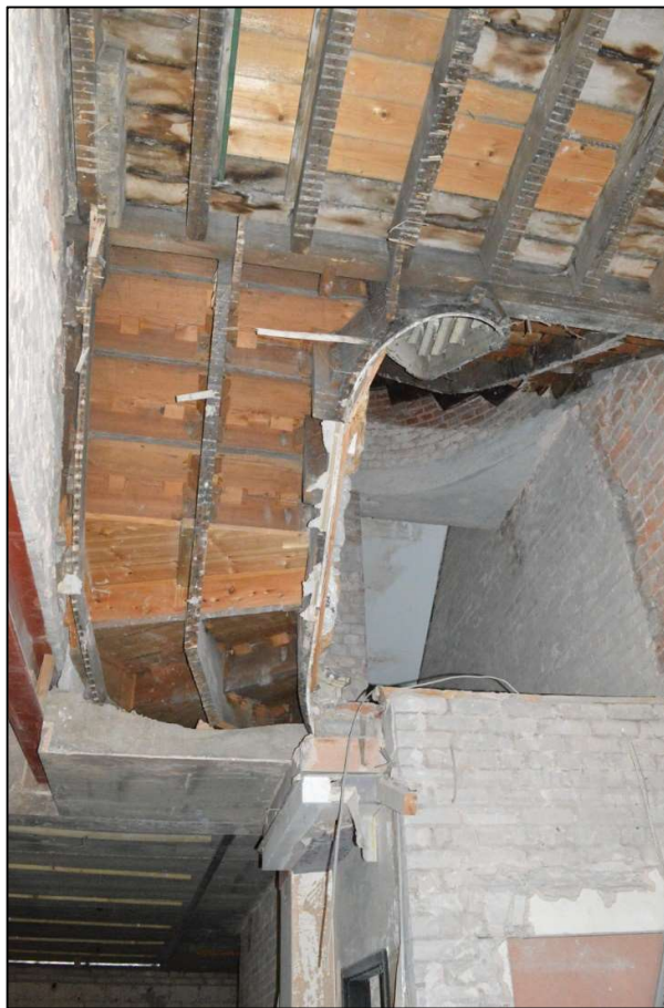
Fig 54: View looking up from the ground floor to the first floor landing of the east stair showing how it was truncated (CPAT 4853-0053)
