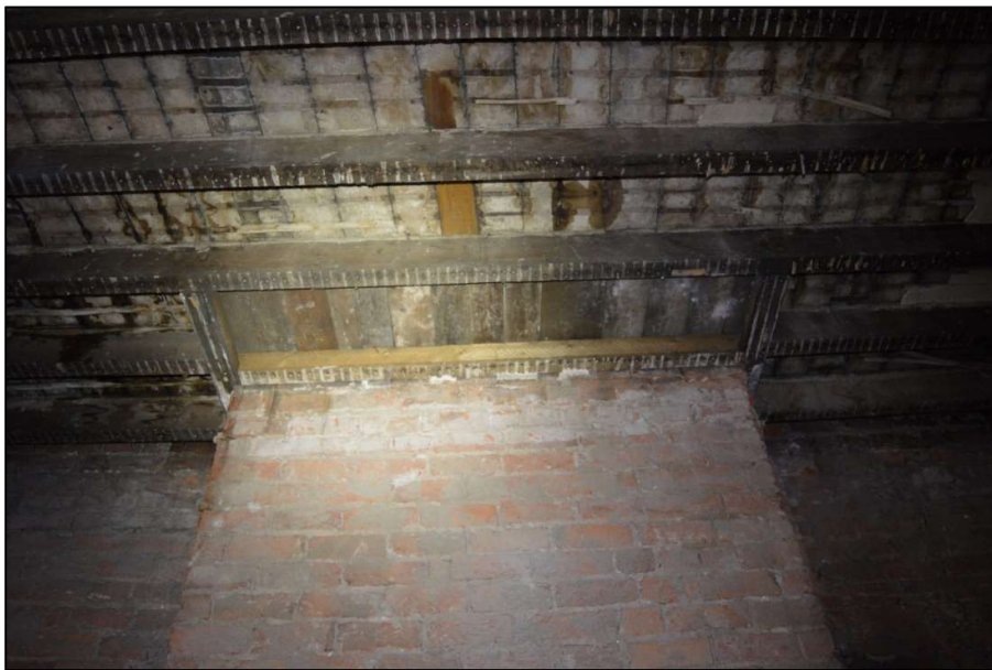
Fig 31: Top of chimney breast in Room 8 on first floor showing supporting timber for the hearth stone (CPAT 4853-0030)
