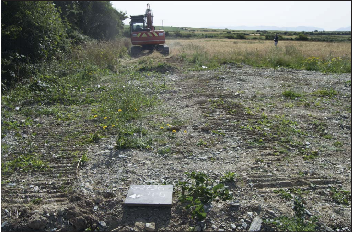
Plate 33: Pre-commencement view of Trench 5 from the west (with board); scale Not used; view from W (archive reference: G2736_05).
