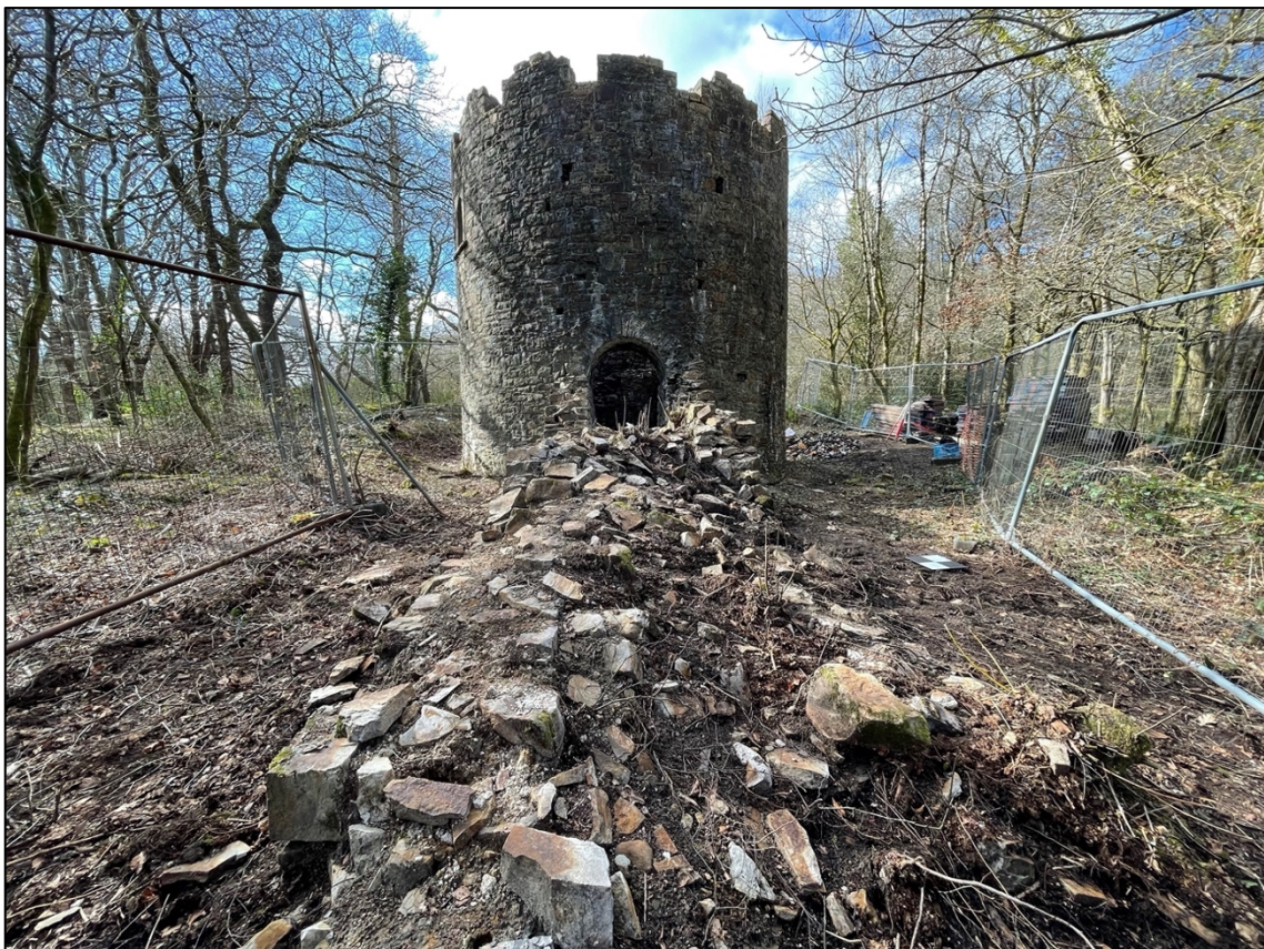
Plate 10 –E facing elevation of Ivy Tower showing external putlog holes and remains of Phase I Flue. GCP scale 0.3m.
