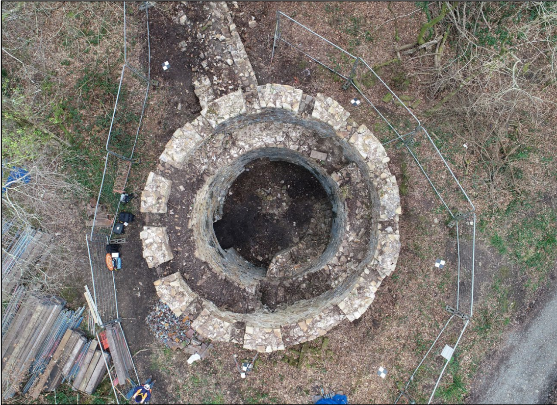
Plate 15 – Nadir view (E = top) of Ivy Tower Phase I chimney base, Phase II gothic battlements and internal staircase. Note missing merlon to WSW. GCPs scale 0.3m.
