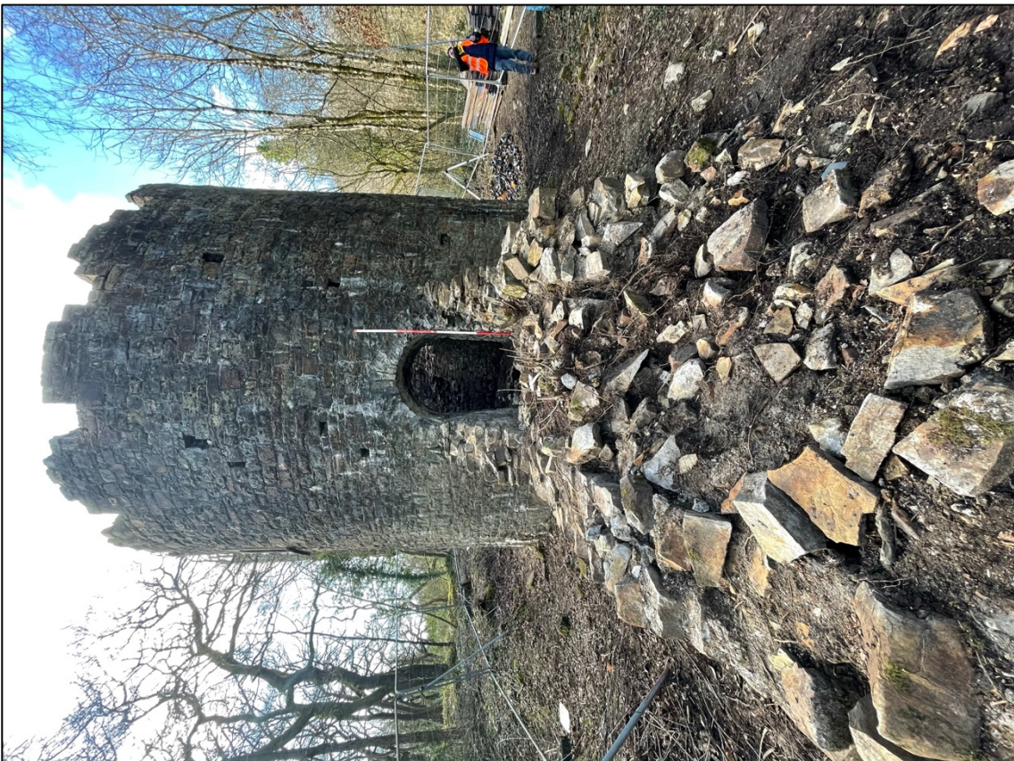
Plate 12 – E facing elevation of Ivy Tower showing external putlog holes and remains of Phase I Flue. Scale 2m.
