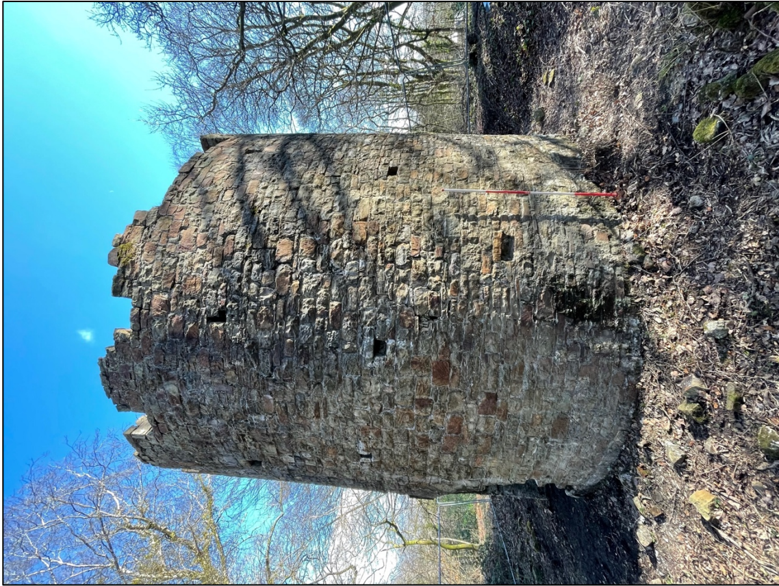
Plate 3 – W facing elevation of Ivy Tower showing external putlog holes. Scale 2m.
