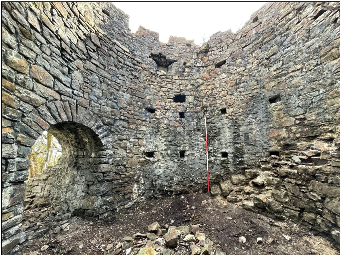
Plate 18 – N facing internal elevation of Ivy Tower showing internal putlog holes and two sets of joist sockets. Scale 2m.
