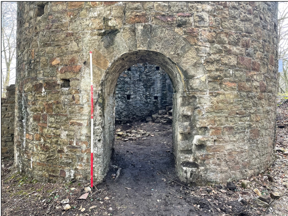
Plate 2 – Inserted Phase II folly door of Pennant sandstone with semi-circular stone arch. N facing elevation Scale 2m.
