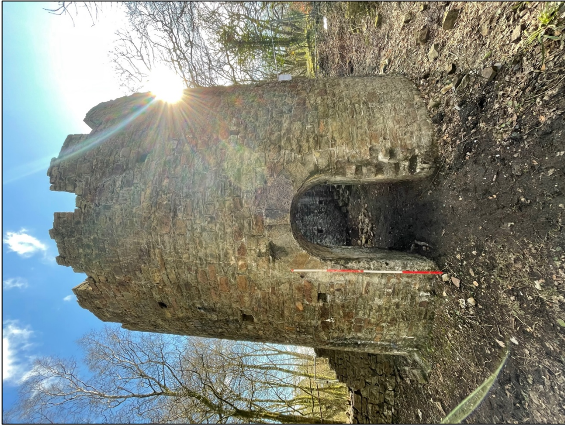
Plate 1 – N facing elevation of Ivy Tower showing inserted Phase II folly door. Scale 2m.
