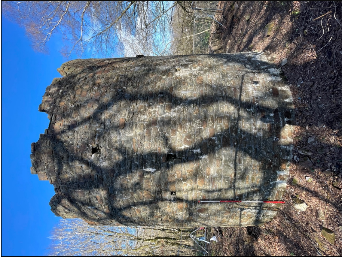
Plate 5 – SW facing elevation of Ivy Tower showing external putlog holes. Scale 2m.
