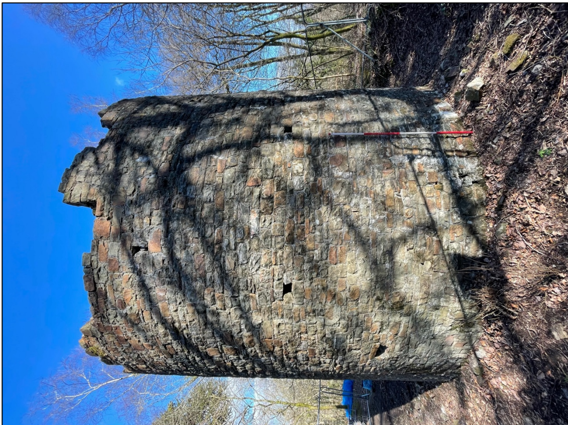
Plate 4 – WSW facing elevation of Ivy Tower showing external putlog holes and missing merlon on battlements. Scale 2m.
