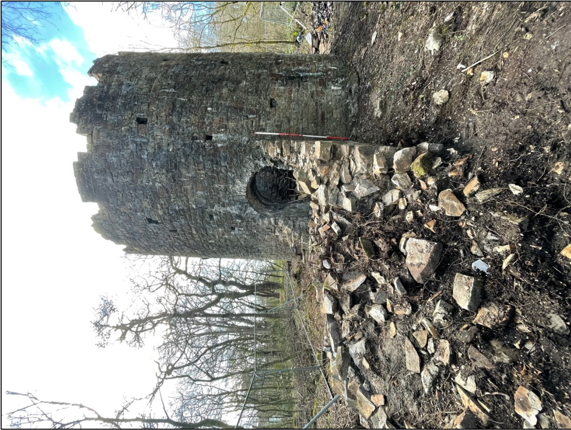
Plate 13 – NE facing elevation of Ivy Tower showing external putlog holes and remains of Phase I Flue. Scale 2m.
