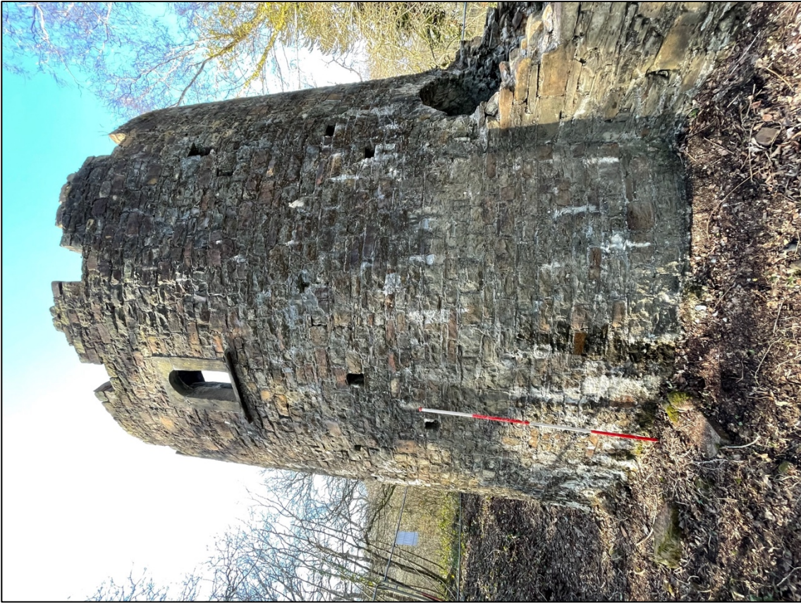
Plate 7 – SE facing elevation of Ivy Tower showing external putlog holes, Phase I Flue and Phase II gothic round-topped window. Scale 2m.
