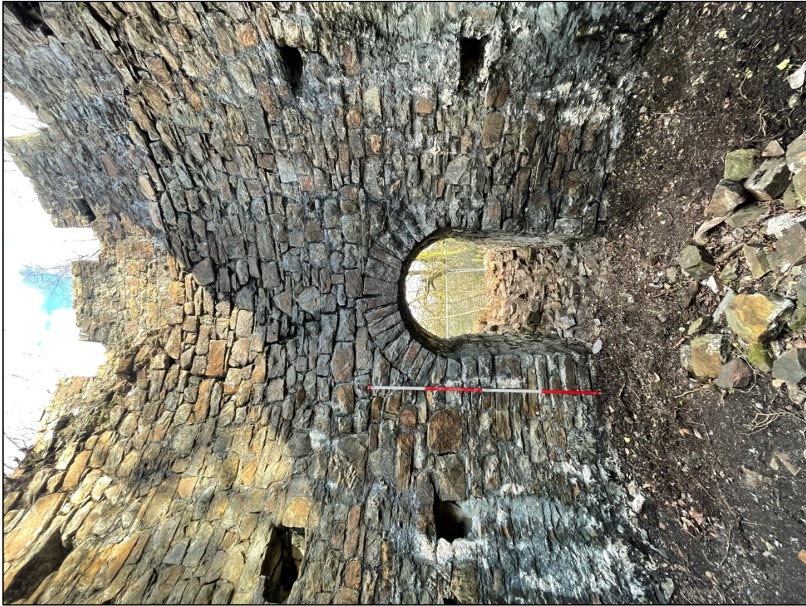
Plate 17 – W facing internal elevation of Ivy Tower showing the Phase I Flue entrance. Scale 2m.
