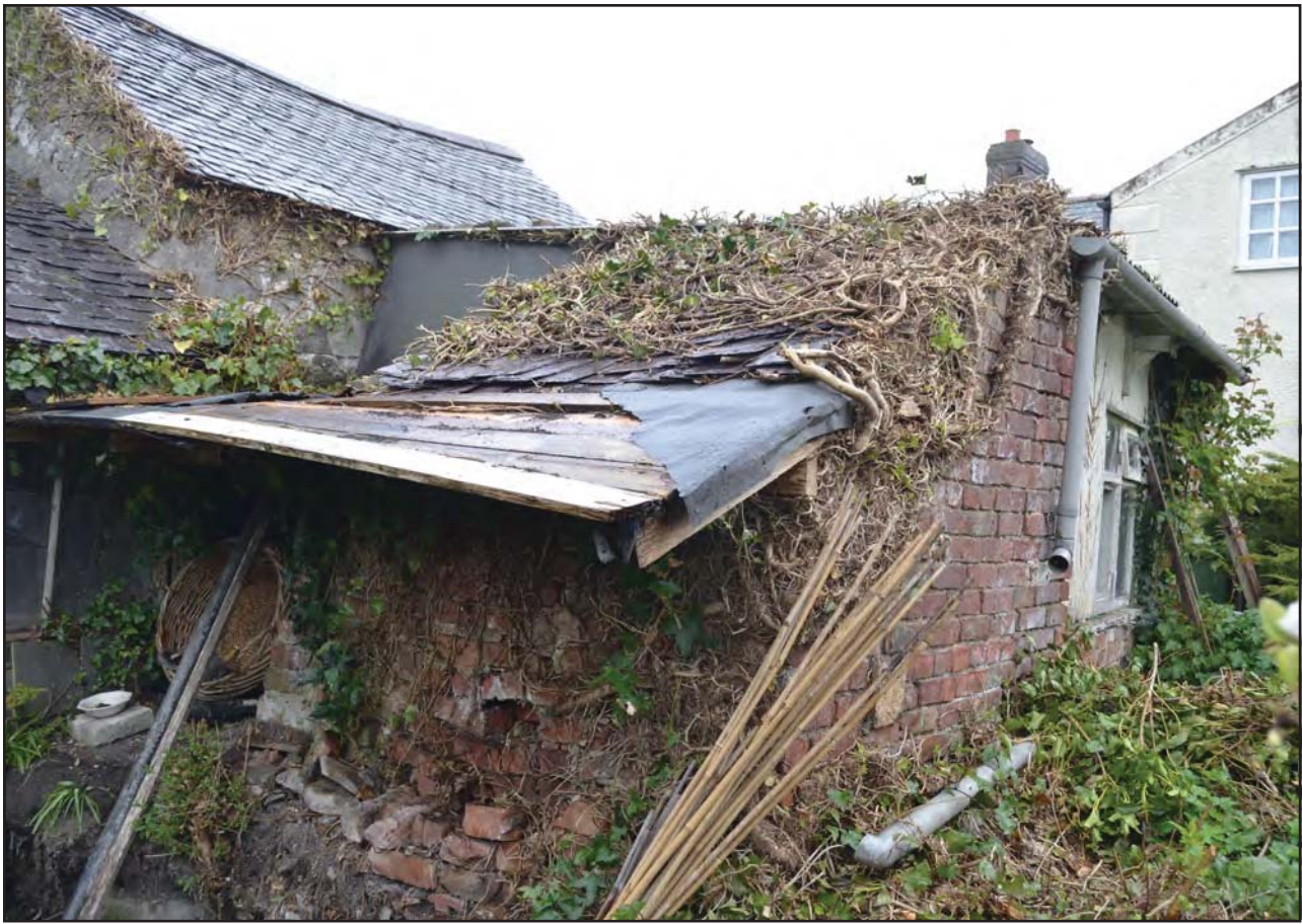
Plate 26: Exterior of outside toilet 1, showing roof, from the west (archive reference: G2776_156)
