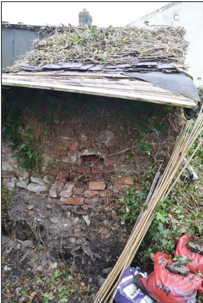
Plate 27: Outside toilet 1 built on thick deposit of earth, from north-west (archive reference: G2776_033)
