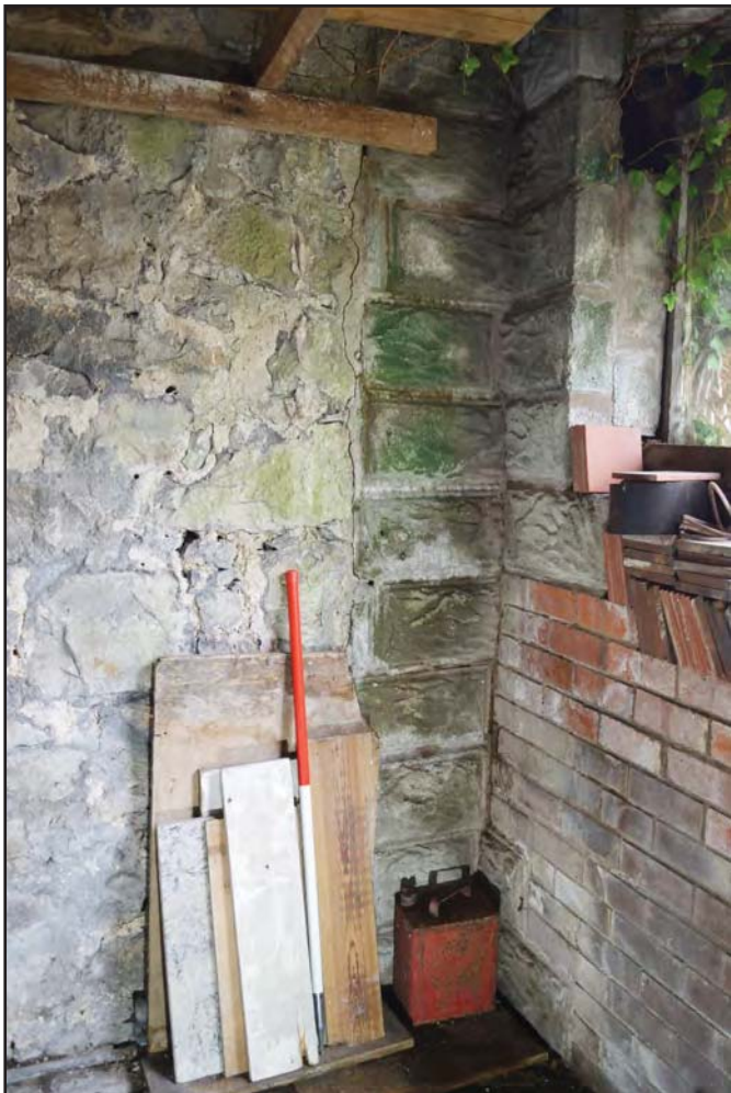
Plate 19: Breeze blocks and brick wall in southern corner of garage; scale 1x1m (archive reference: G2776_124)
