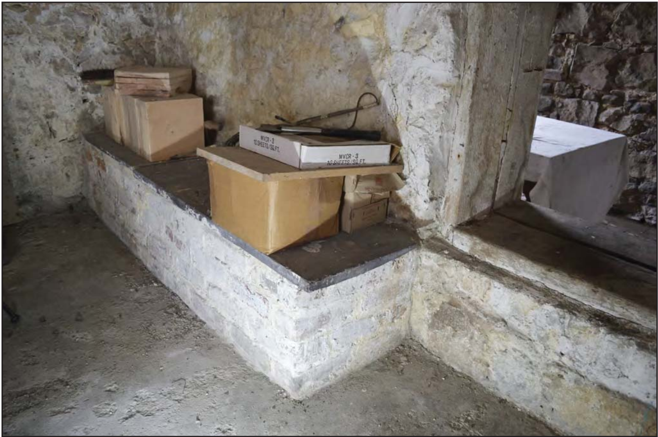
Plate 8: Brick shelf in outbuilding ground floor room, from the east (archive reference: G2776_115)
