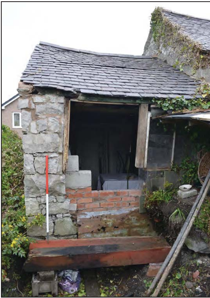
Plate 18: Rear wall of the garage, from the south-west; scale: 1x1m (archive reference: G2776_031)
