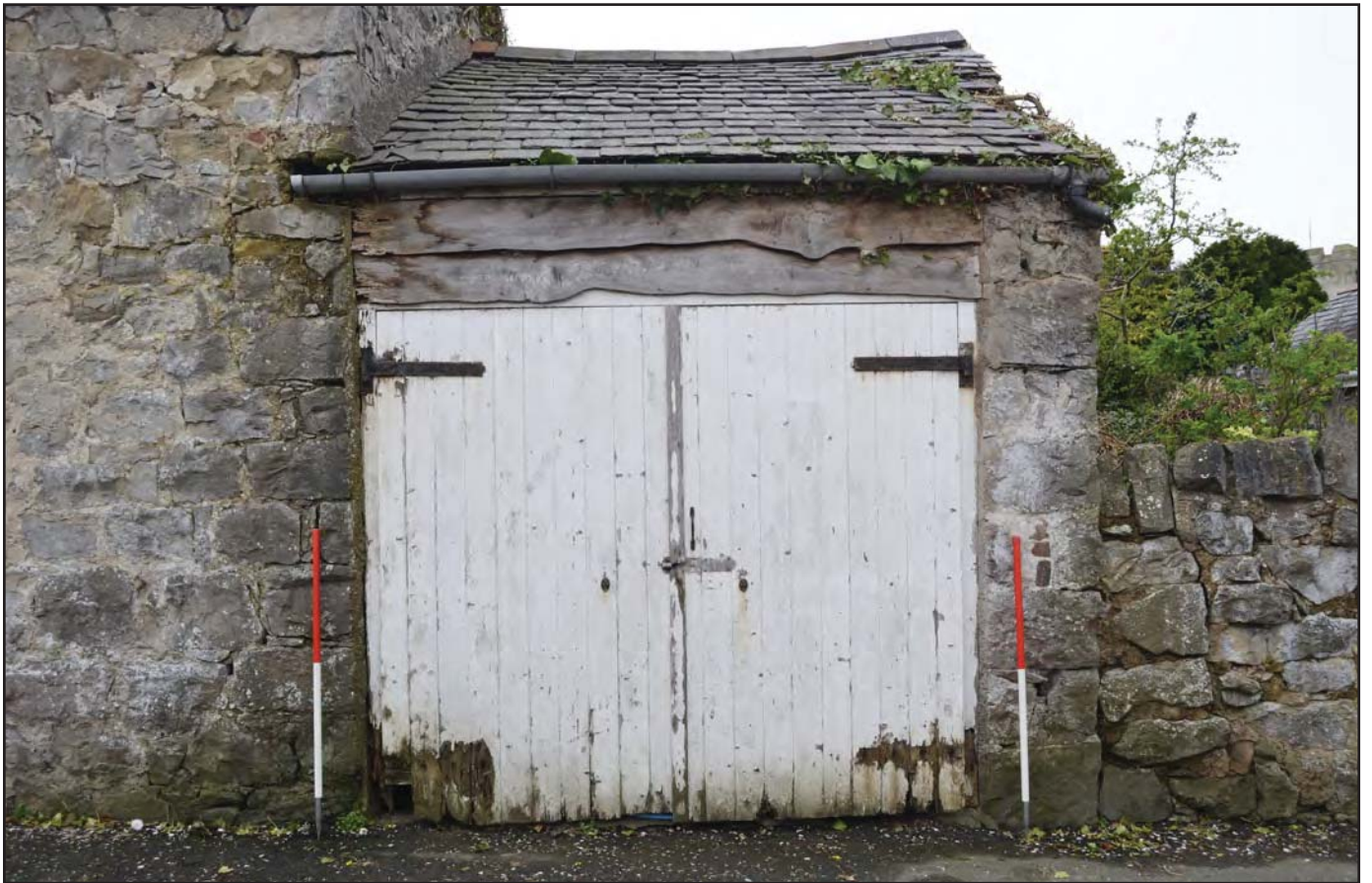
Plate 16: North-east elevation of the garage, from the north-east; scale: 2x1m (archive reference: G2776_011)
