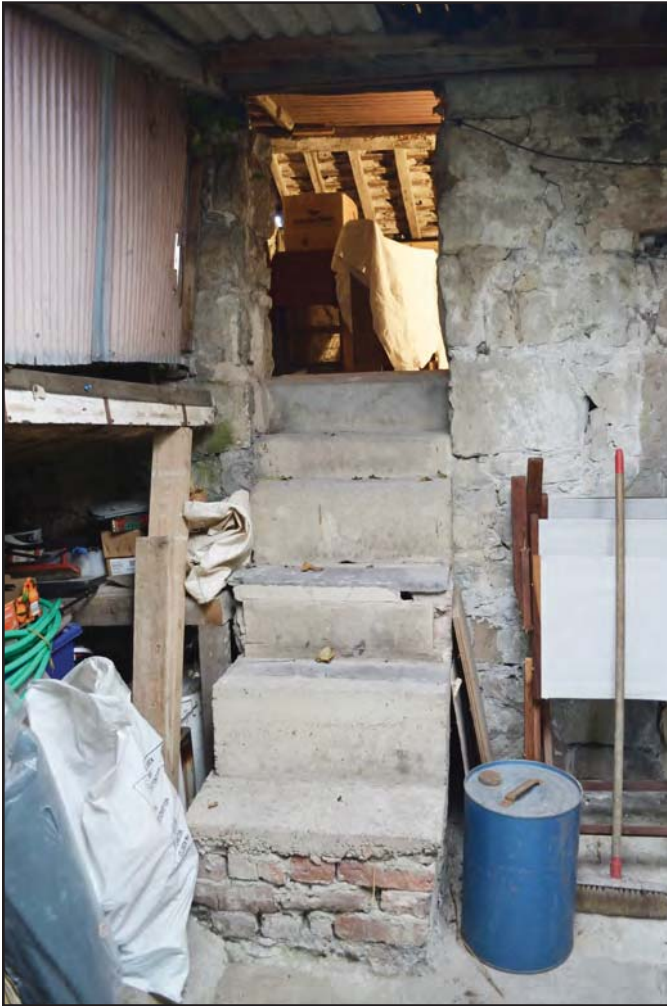
Plate 12: Steps up to entrance to upper room in outbuilding, from the south-west (archive reference: G2776_053)
