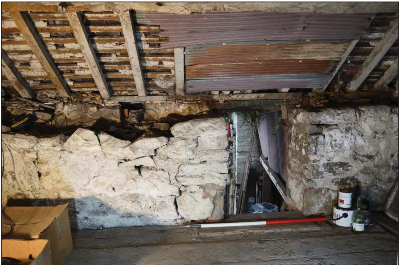
Plate 13: South-west wall and roof of upper room of outbuilding with entrance, from the north-east; scale: 1x1m (archive reference: G2776_073)
