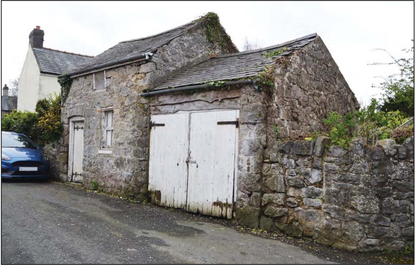
Plate 1: Outbuilding and garage from Church Street, from the north (archive reference: G2776_015)
