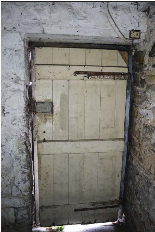
Plate 6: Interior of door in ground floor room in outbuilding, from the south-west (archive reference: G2776_140)
