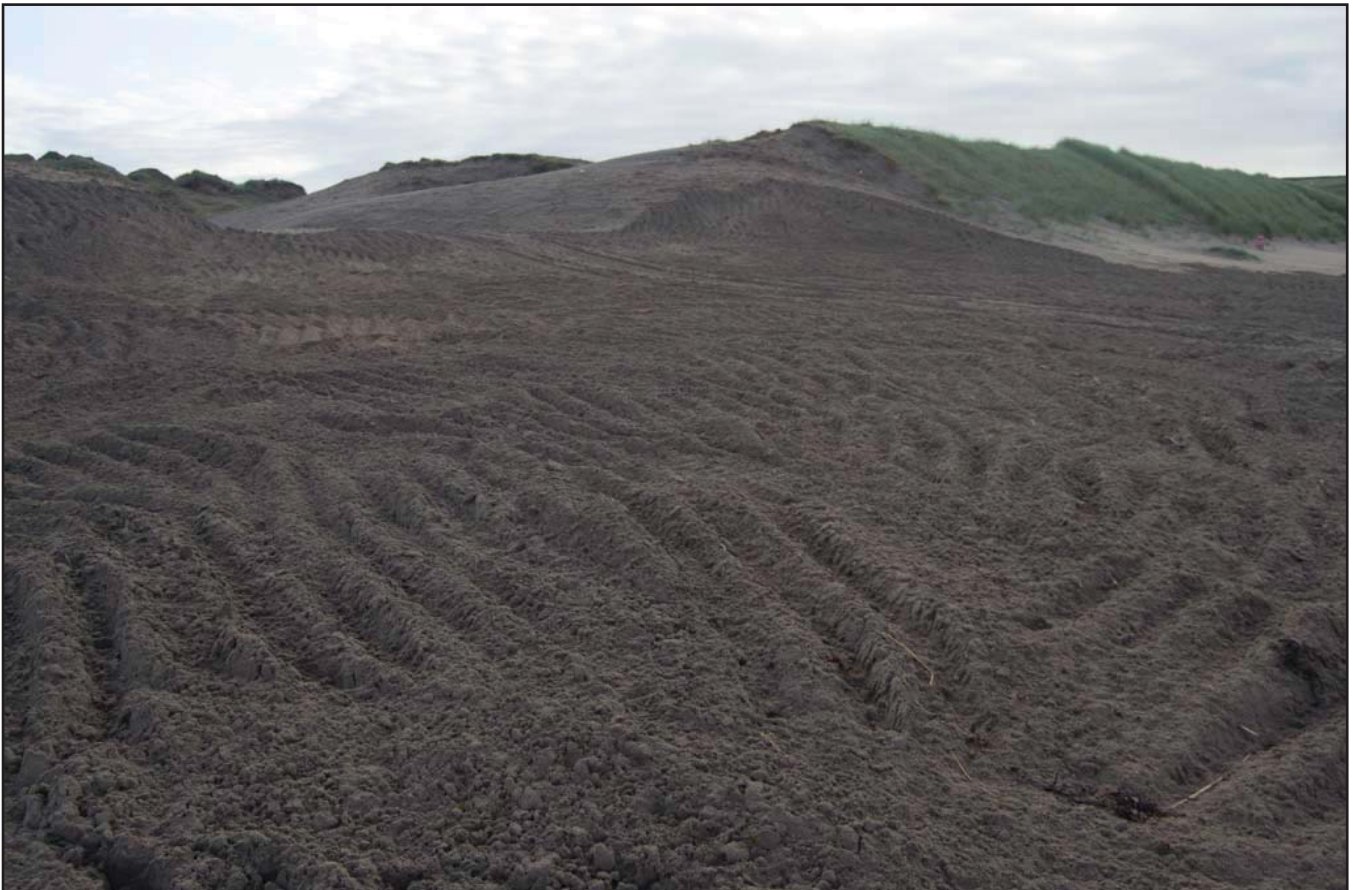
Plate 10: View of the notch after excavation completed from the beach; (archive reference: G2742_65).
