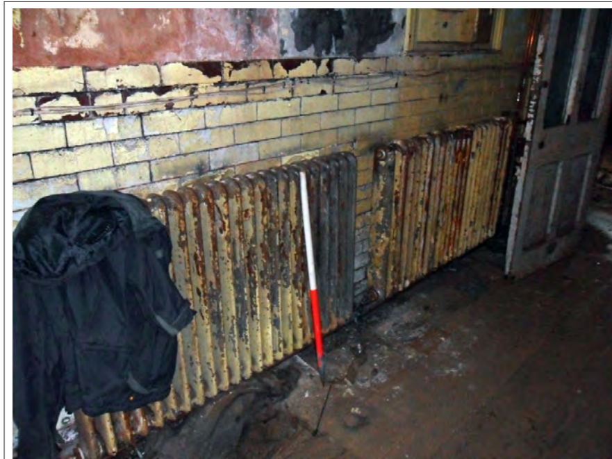
Plate 11: View of original radiators fitted to east wall of Room 4 Scale 1x1m
