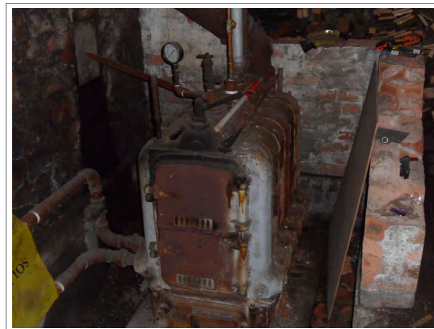
Plate 44: View of boiler/stove located within brick surround and recess within Room 9, Scale 1x1m
