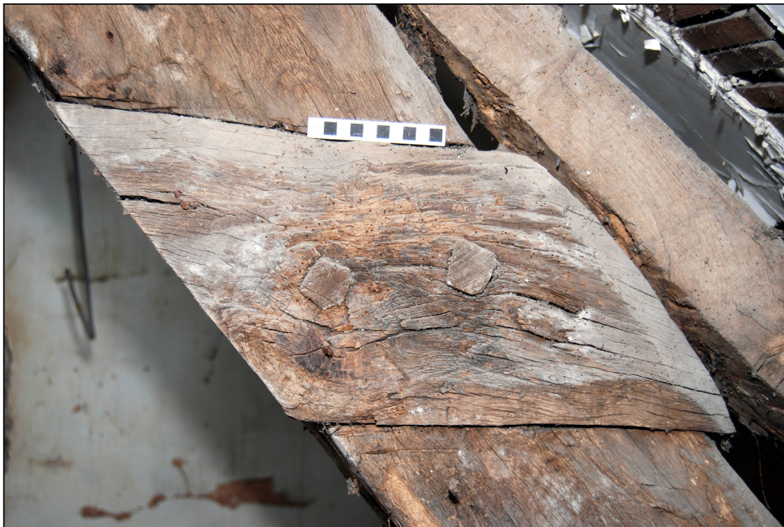
Plate 14: Remains of the collar on the northern principal rafter of Truss 1
