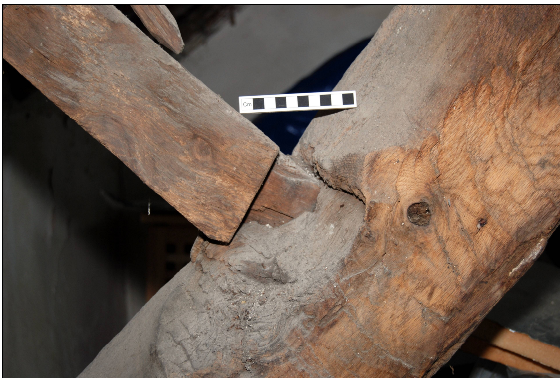
Plate 22: Detail of the joint between the southern principal rafter and the support for the secondary rafter of Truss 1
