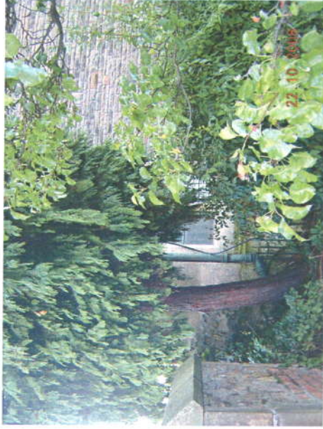
Tree T1 (proximity to building & foul drainage)
