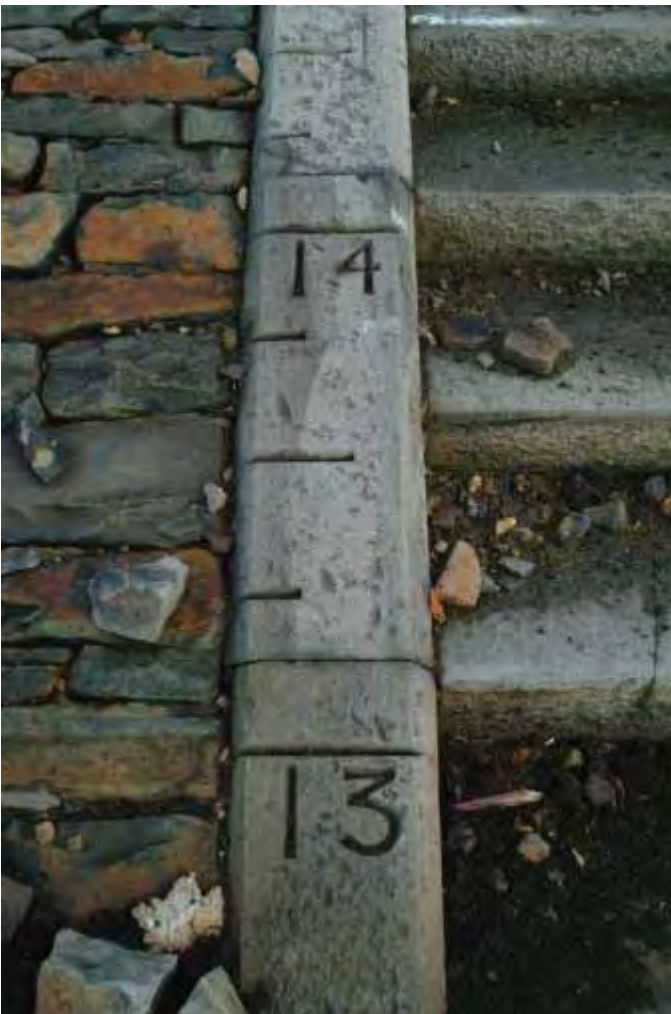
Appendix 5.20: Incised water level markers on original stairs, view to the east
