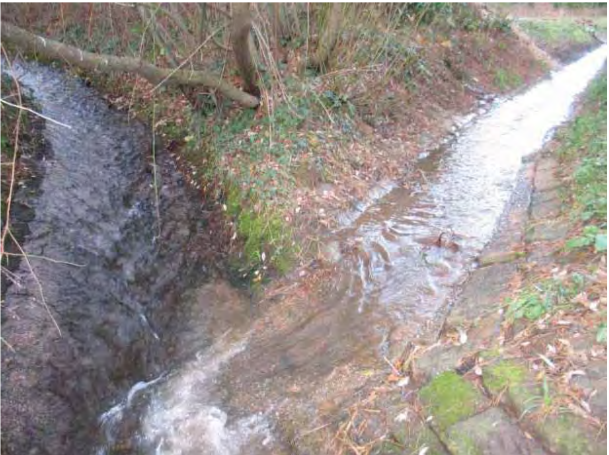
Appendix 5.8: Confluence of the Bye Channel (left) and the Nant Mawr discharge culvert
