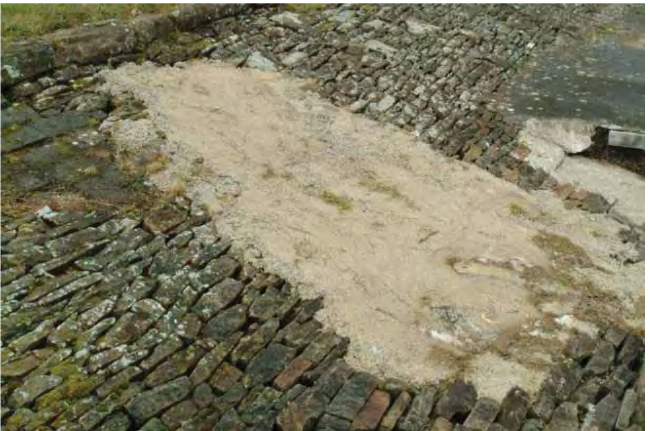
Appendix 5.18: Concrete patch to stone embankment facing, view to the northwest
