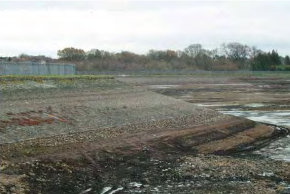
Appendix 5.3: General view of the stone facing to the inner slope of the northern embankment
