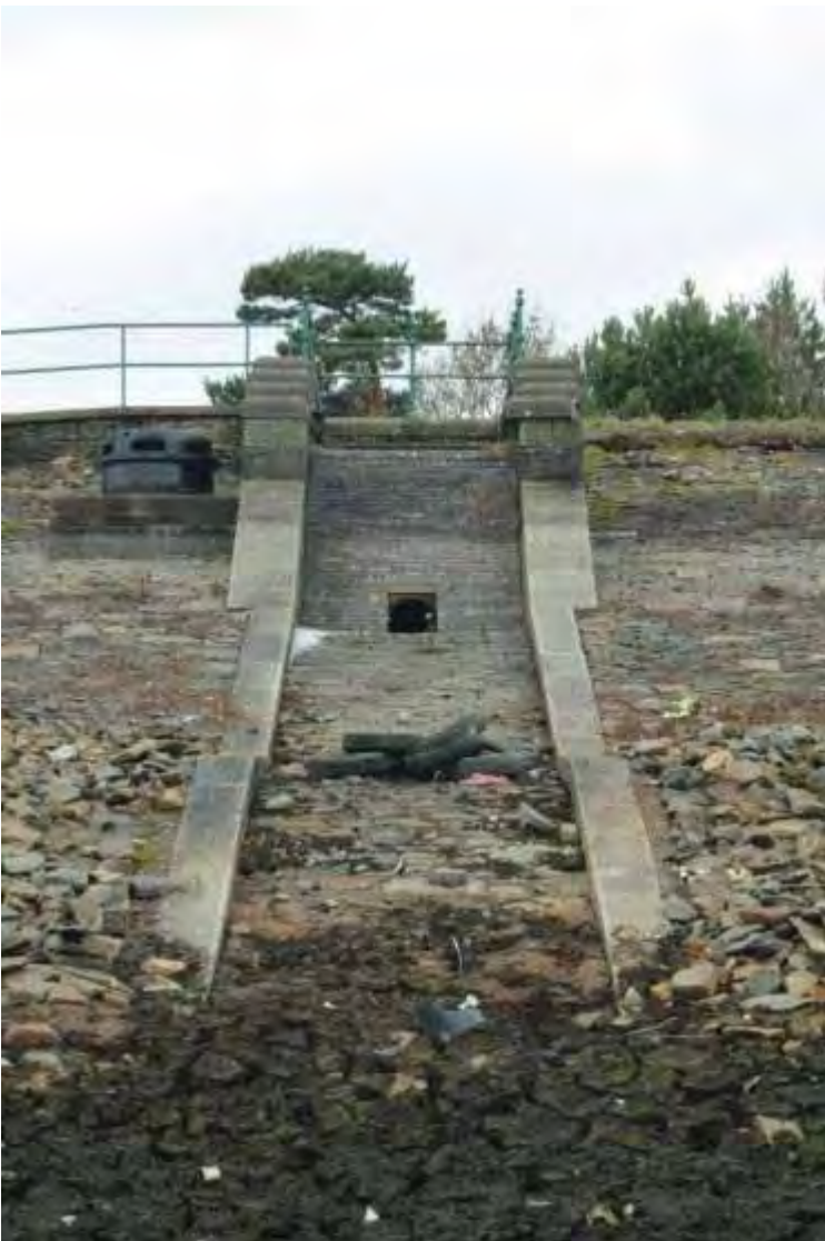
Appendix 5.4: Detail of original inflow, spillway and overflow, view to the west
