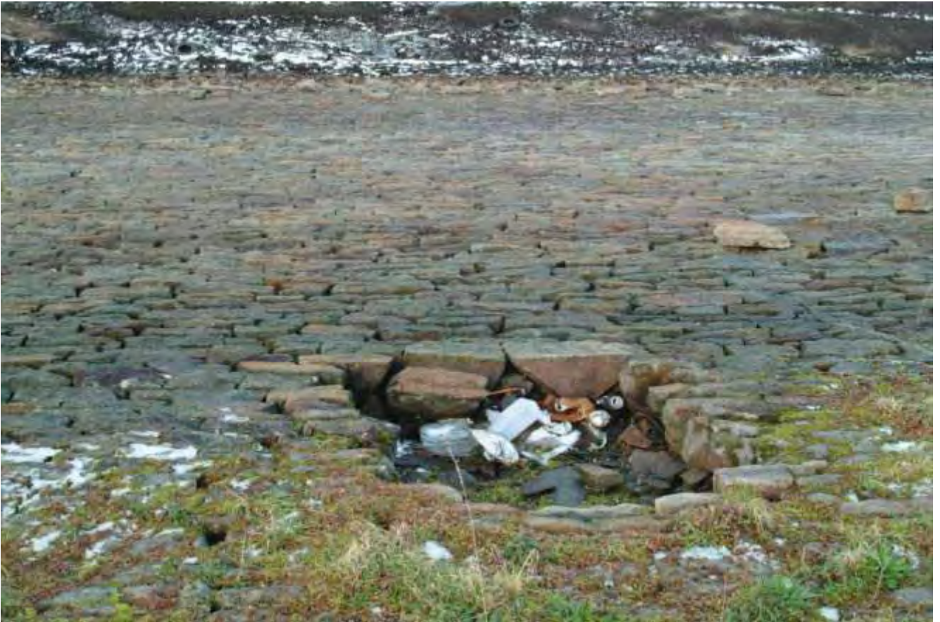
Appendix 5.17: Hole in stone embankment facing, view to the northeast
