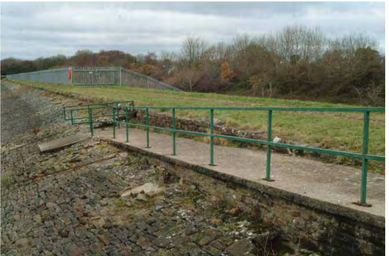
Appendix 5.16: Damaged upper kerb adjacent to the inserted access ramp
