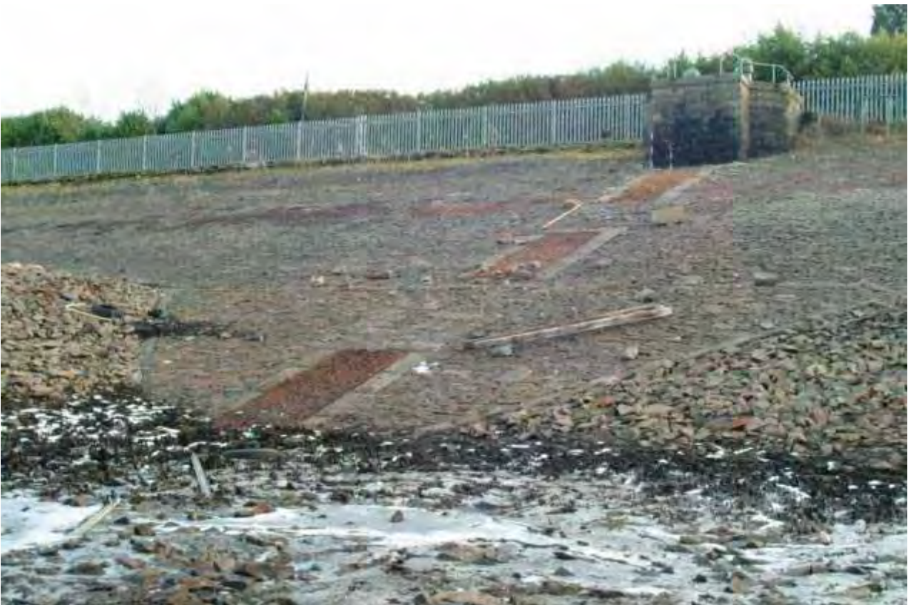
Appendix 4.6: Three tier decanting culverts in southern embankment, view to the southeast
