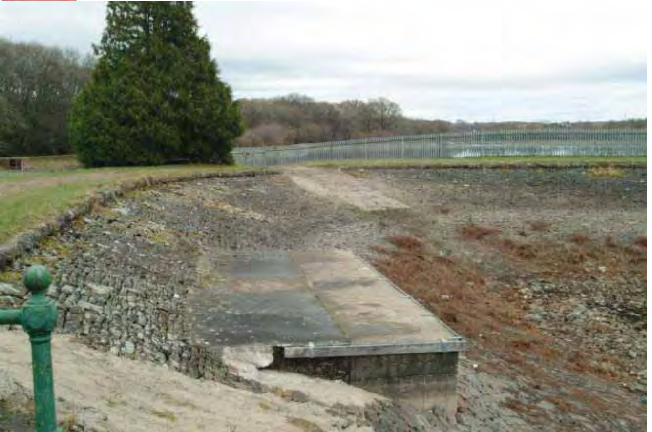
Appendix 5.15: Damaged facing and kerb around concrete jetty and boat slipway, view to the north
