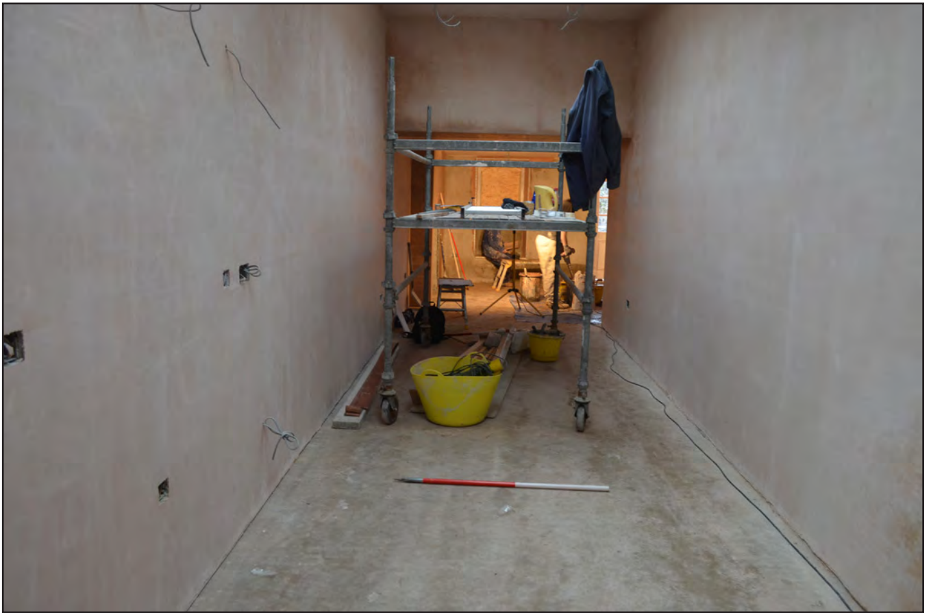
Plate 11: Interior view from the west of the new extension (Scale: 1 x 1m).
