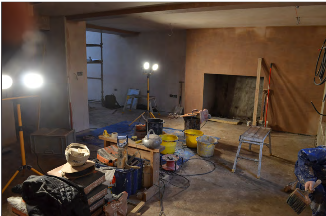
Plate 09: Internal view from southwest of central ground floor during conversion into lounge & dining room at eastern half of the cottage (Scale: 1 x 1.0m)
