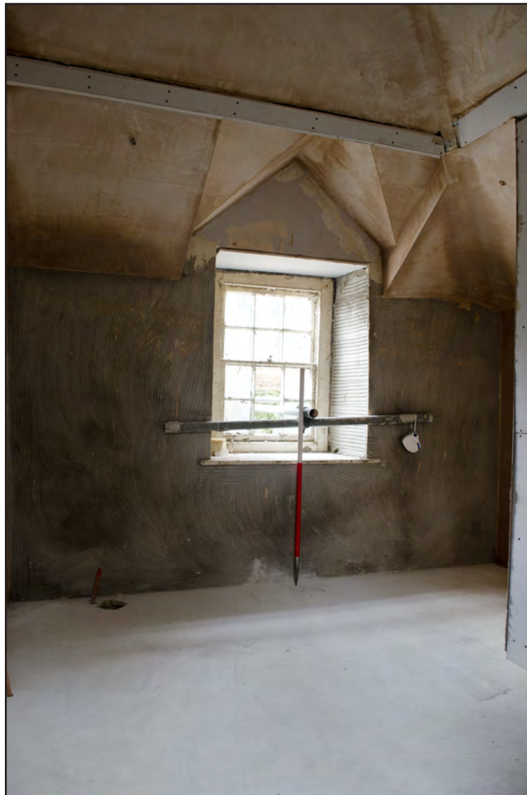
Plate 20: Internal view of first floor window in southern wall of main bathroom (Scale 1 x 1m).
