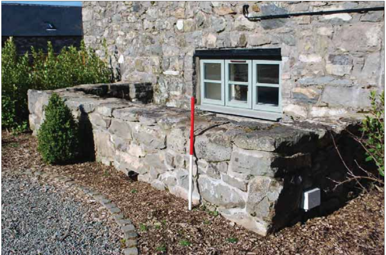
Plate 4 View of the mill-wheel pit at Pistyll Farm from the south east. Scale 1m
