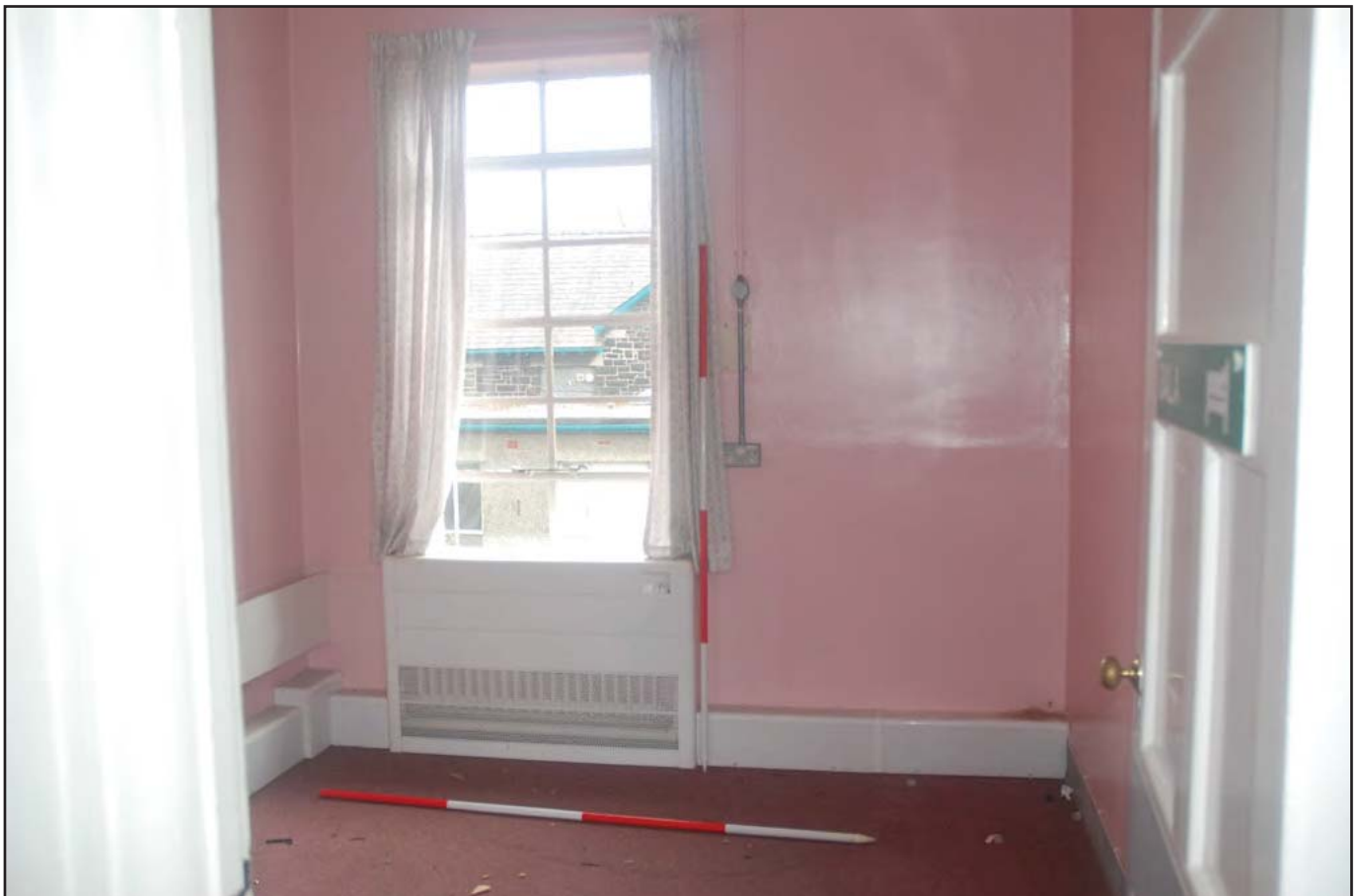
Plate 32: Short Stay Unit (Internal): View southeast of Room G08 detailing current use as a ward. Storage heater visible below original casement window, with boxed in plumbing. Panelled and moulded entrance door visible in image foreground. Rear of Long Stay Unit through window (Scales: 2 x 2.0m)
