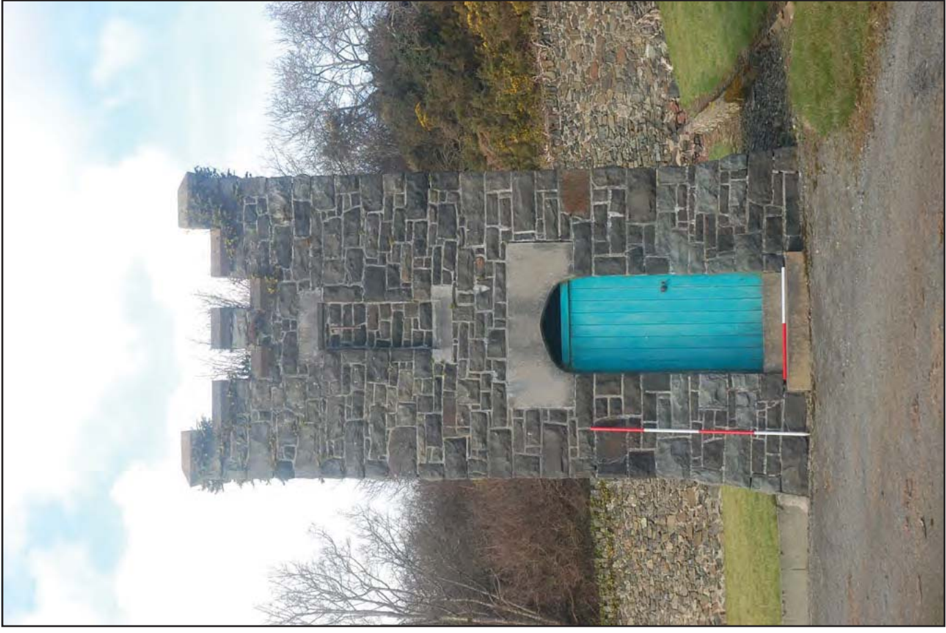
Plate 52: Water Tower - Southeast facing elevation detailing construction form, including crenellated capping, internal buttress and main entrance via pannelled door. Note the boundary wall at rear of image (Scales: 2 x 2.0m).
