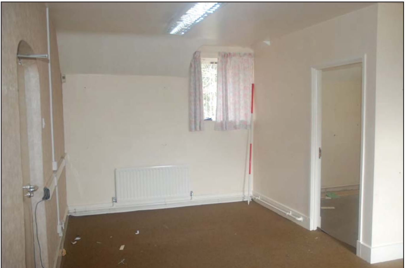
Plate 50: Administration Block (Internal): View northeast of former nurses changing room (Room F03) with the former sister's changing room (Room F04) as a boxed partition at right of image. Room F03 was converted from four rooms into two rooms (F03 and F04), with the removal of a sister's bedroom and a cook's bedroom. The original corridor entrance has been converted into the main entrance for F03 and is approached via a staircase and small landing (cf. Plate 48) (Scales: 1 x 2.0m).
