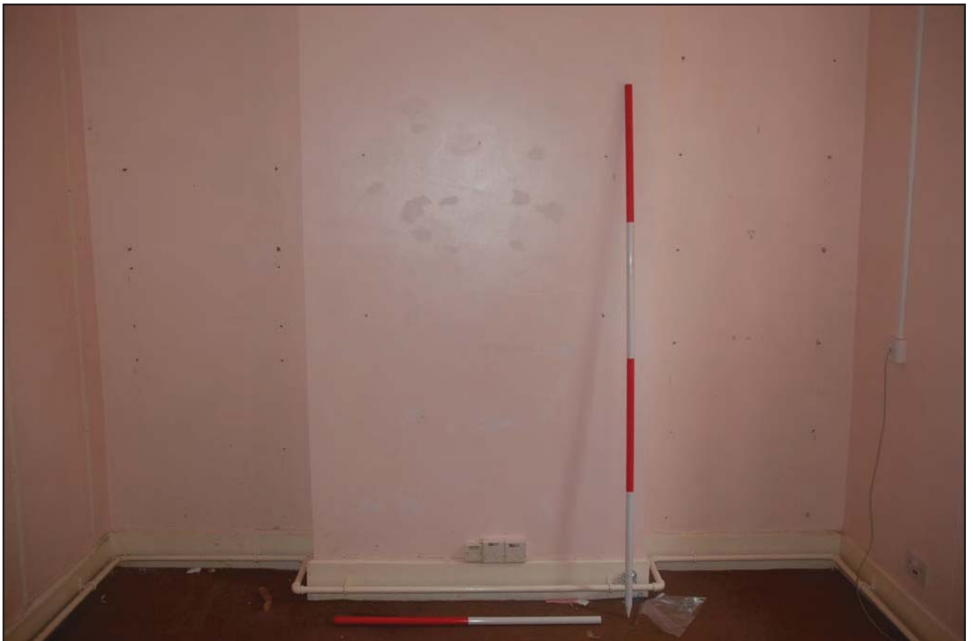
Plate 48: Administration Block (Internal): View northeast of former maid's sitting room (Room G04) detailing redundant fireplace. Scales: 1 x 2.0m and 1 x 1.0m.
