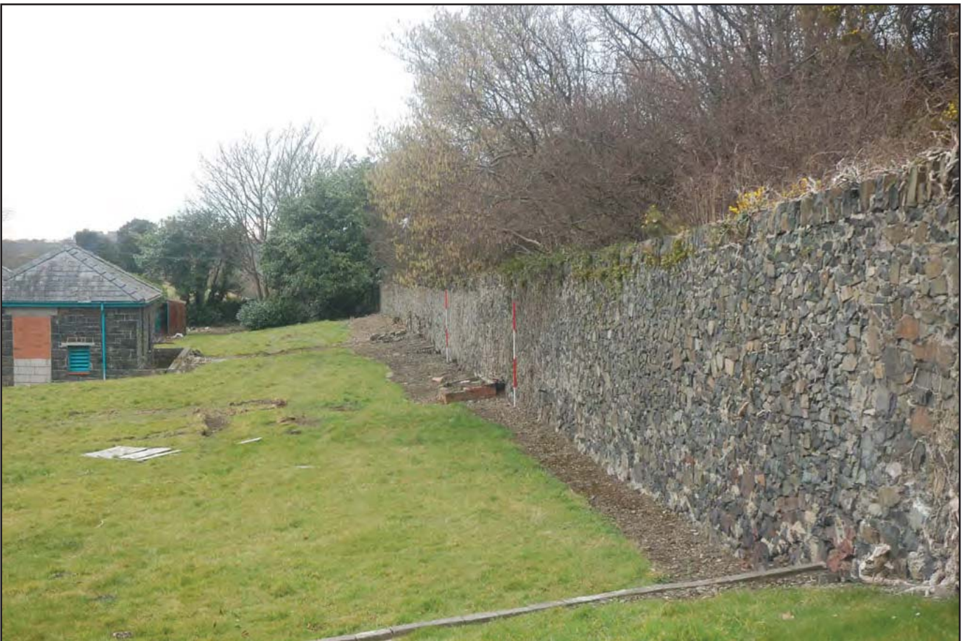
Plate 66: Boundary Wall - View west of rear portion, detailing construction (irregular stones and crenellated surmount) and height (2.50m max). Note the generator in image left and gravel path running along the base of the wall. (Scale: 2 x 2.0m)
