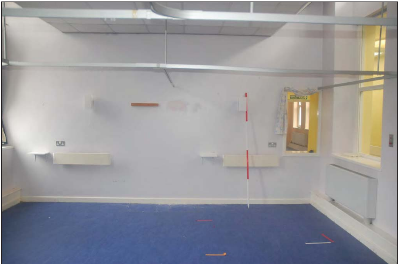
Plate 14: Long Stay Unit (Internal): Room G05 - view southeast detailing former male ward. All doors are fire doors. Bullnose skirting boards are visible. Note: internal corridor visible through openings (Scales: 2 x 2.0m)
