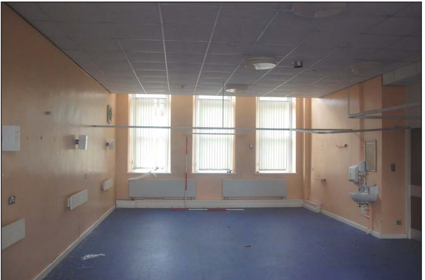
Plate 16: Long Stay Unit (Internal): Room G11 - view southeast of former female ward, detailing window fittings and bullnose skirtings. Original ceiling is disguised by a suspended ceiling (Scales: 2 x 2.0m)
