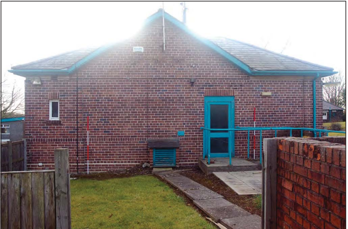
Plate 22: Short Stay Unit: Northeast facing elevation with gable end of the former Day Room (Room G01) visible. The door towards the right of image provides access to the central corridor of the building (Scales: 2 x 2.0m)
