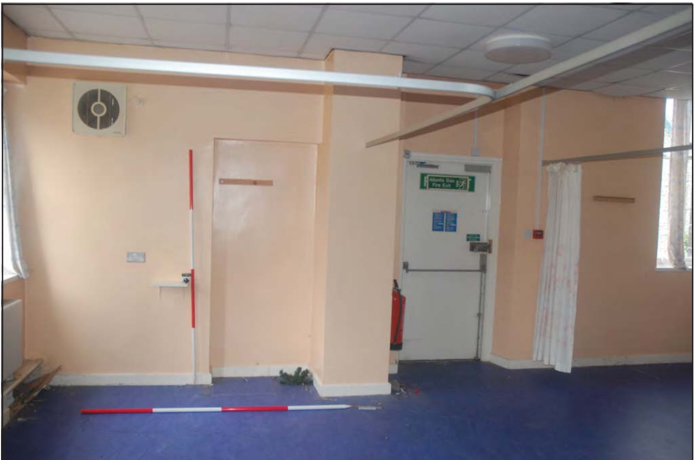
Plate 18: Long Stay Unit (Internal): Room G12 - view northeast of former female ward annexe. This room was created from the conversion and alteration of the former sewing, treatment and linen rooms into one room; therefore, most of the original internal structural elements have been altered and/or disguised. The partition wall separating the sewing and linen rooms can still be seen as a truncated stub; the entrance into the sewing room from outside can be seen as a blocked door. The alterations were completed after 1984 (Scales: 2 x 2.0m)
