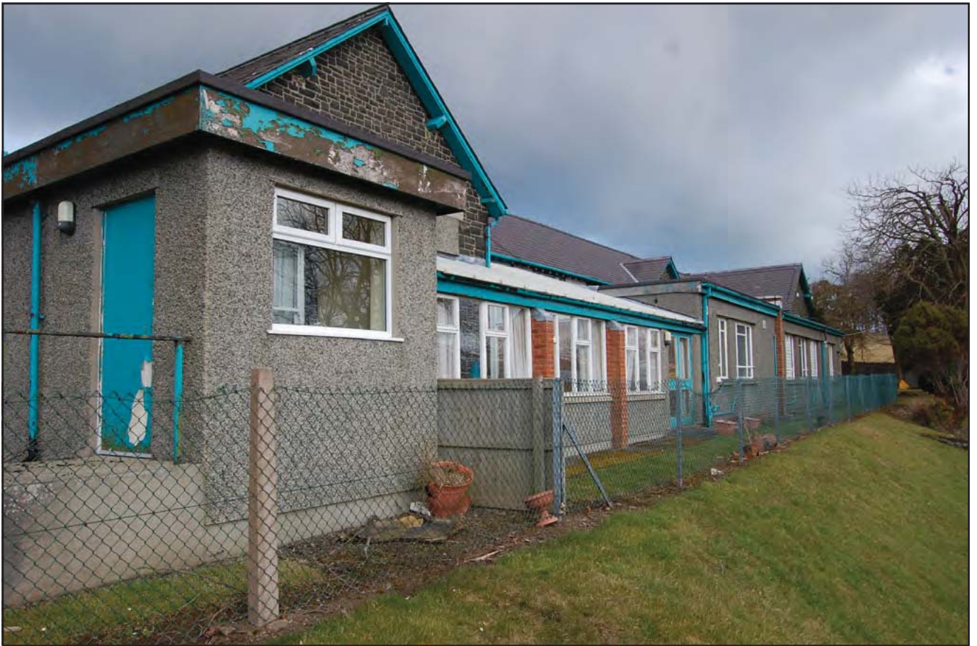
Plate 03: Long Stay Unit (External): Southeast facing elevation detailing late twentieth century veranda extension and flat roof extensions to the original structure. The Link Corridor is in the left foreground of image. The gable end of the male wing is also visible in the foreground, detailing original structural style.
