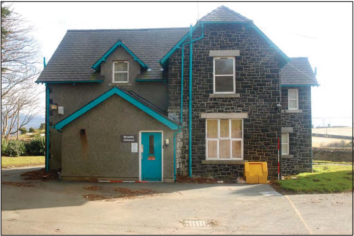
Plate 43: Administration Block: Northwest facing elevation detailing ground floor Room G04 and first floor Rooms F03 to F05. The rear of the property was altered c.1991, with the removal of a ground floor wing that included a kitchen, prep room and store. The kitchen was reduced in size to create the pebbledashed gabled main entrance/photocopy room visible in the image. Remnants of the alteration work can be seen where the main entrance is keyed into the original build. (Scales: 2 x 2.0m)
