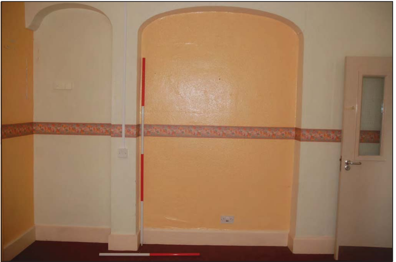
Plate 47: Administration Block (Internal): View northeast of former matron's office (Room G03) detailing redundant archways and modern fire door. Scales: 1 x 2.0m and 1 x 1.0m.
