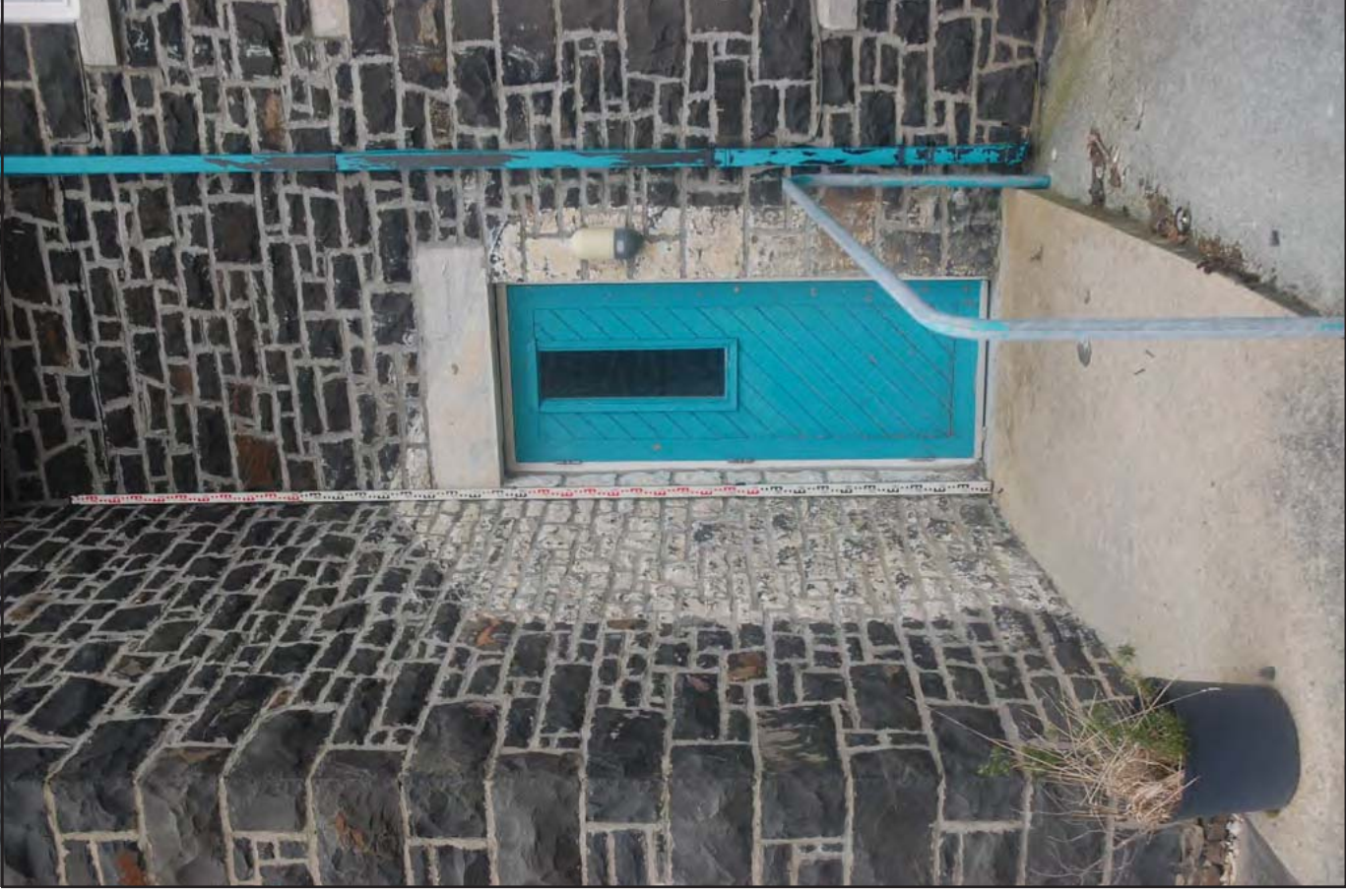
Plate 42: Administration Block: Southeast facing elevation. Ground floor former main entrance (now a fire exit) with a panelled door. Original porch has been removed, but outline is still visible. (Scale 1 x 5.0m).
