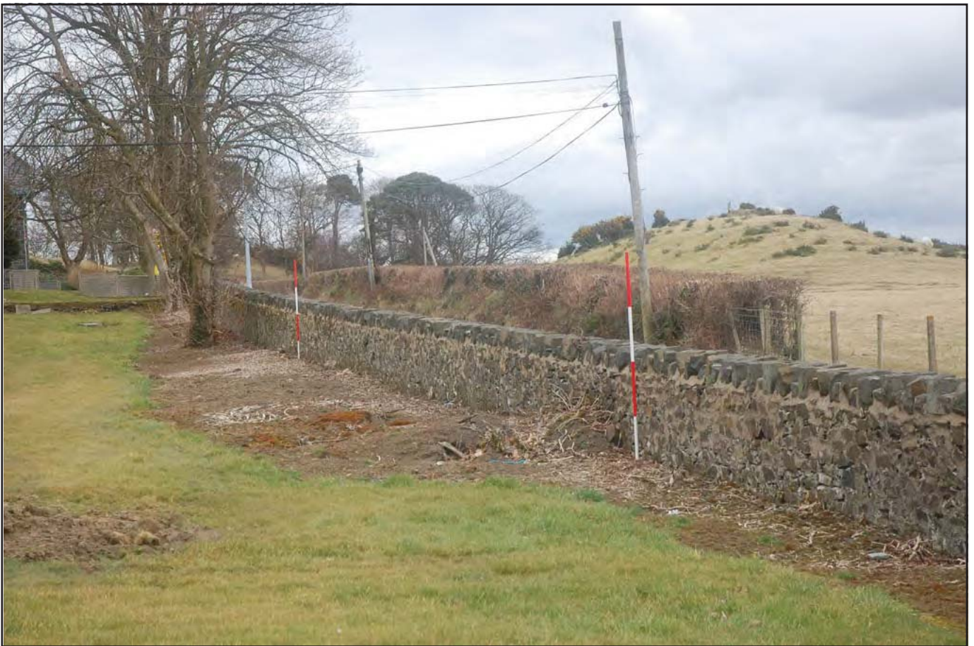
Plate 63: Boundary Wall - view south of portion running parallel to Hendrewen Road. Built from irregular shaped stone with a crenellated surmount. (Scale: 1 x 2.0m)
