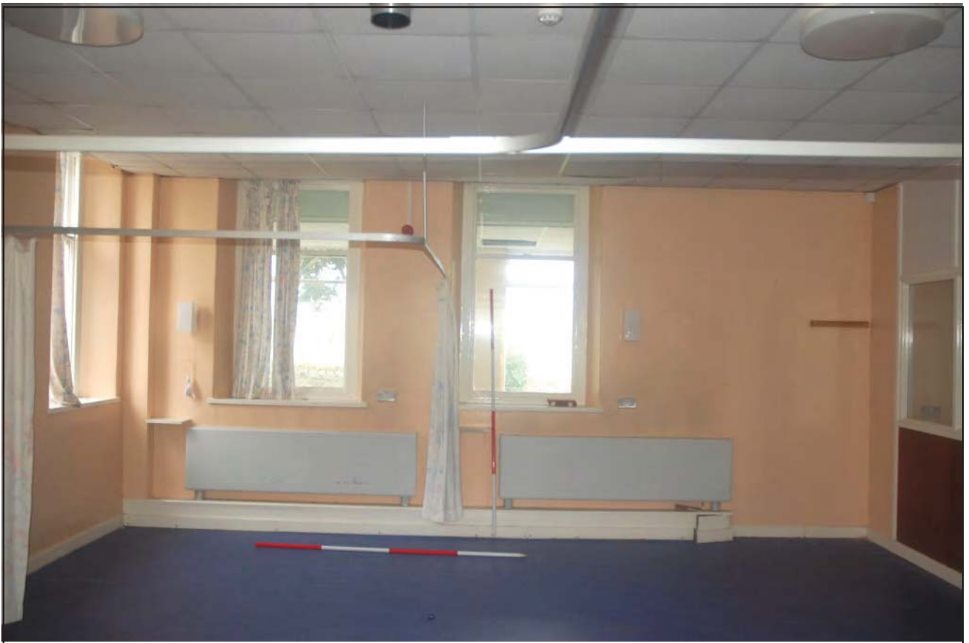
Plate 17: Long Stay Unit (Internal): Room G12 - view southeast of former female ward annexe. This room was created from the conversion and alteration of the former sewing, treatment and linen rooms into one room; therefore, most of the original internal structural elements have been altered and/or disguised. A suspended ceiling is in place and the screen separating Rooms G12 & G11 can be seen to the right of the image (Scales: 2 x 2.0m)
