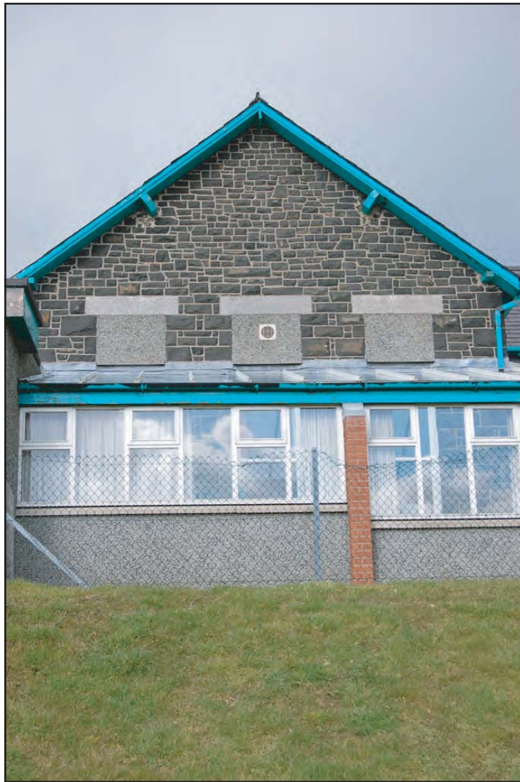
Plate 05: Long Stay Unit (External): Southeast facing elevation detailing late twentieth century veranda extension to the original structure (Rooms G03 and G07). The gable end of the male wing (Room G01) is also visible, detailing original structural style and blocked windows.
