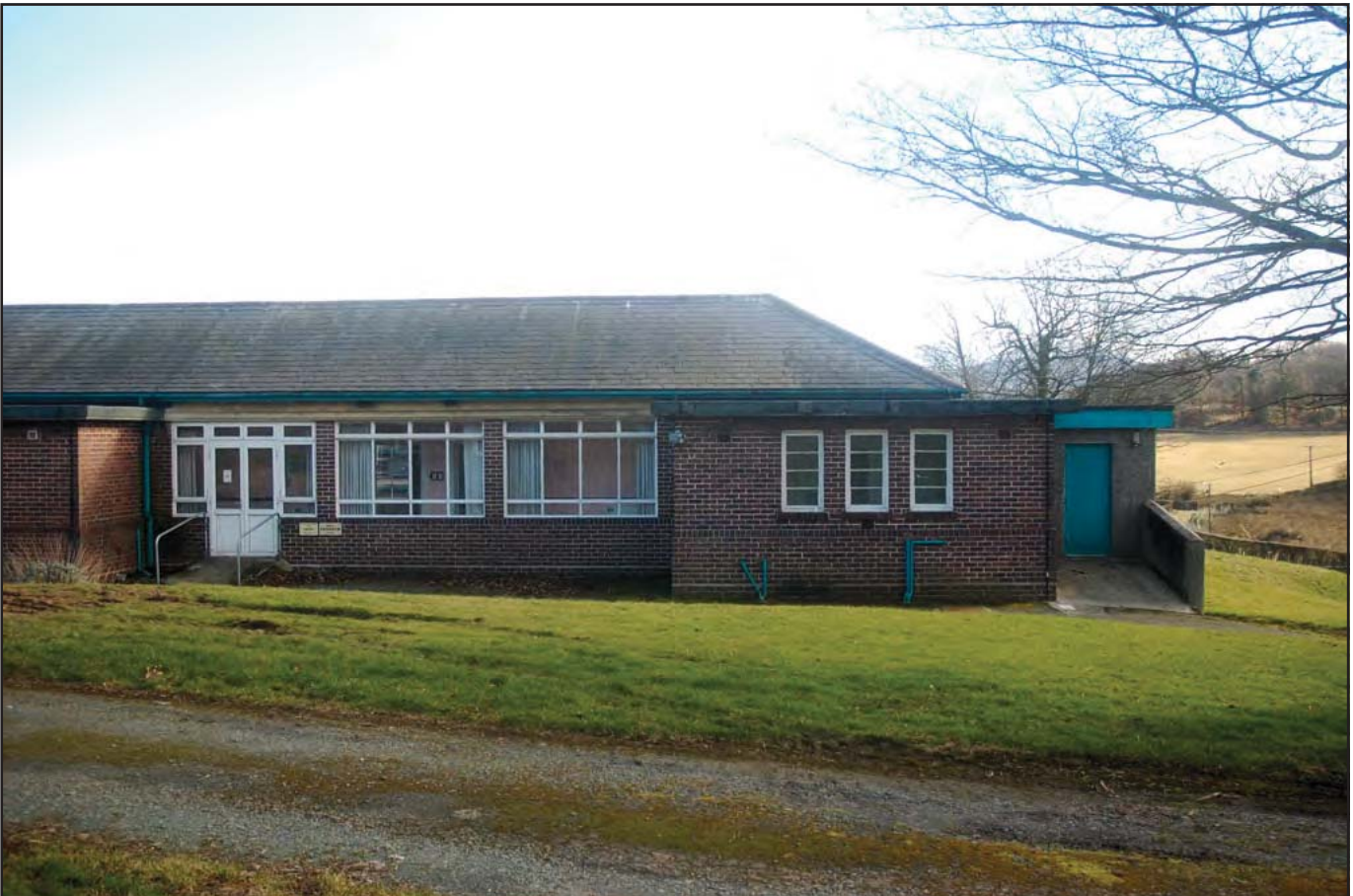
Plate 24: Short Stay Unit: Northwest facing elevation - main entrance and Room G11 (Kitchen); detailing English Garden Wall bond brick style and casement windows. Note the link corridor attached to the southwest facing elevation towards right of image
