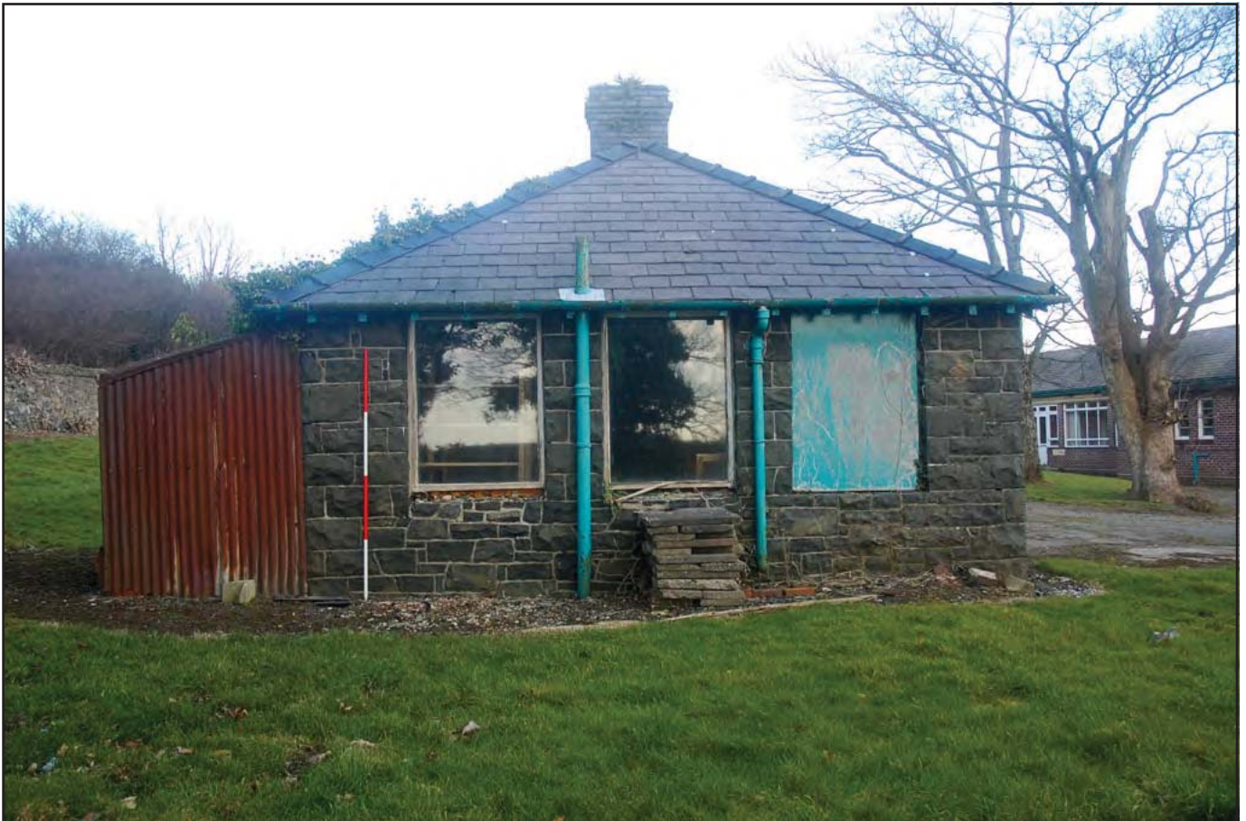
Plate 54: Garage - Southwest facing elevation detailing three fixed windows, hip gable roof and brick built chimney. The corrugated lean to is a later addition (Scale 1 x 2.0m)
