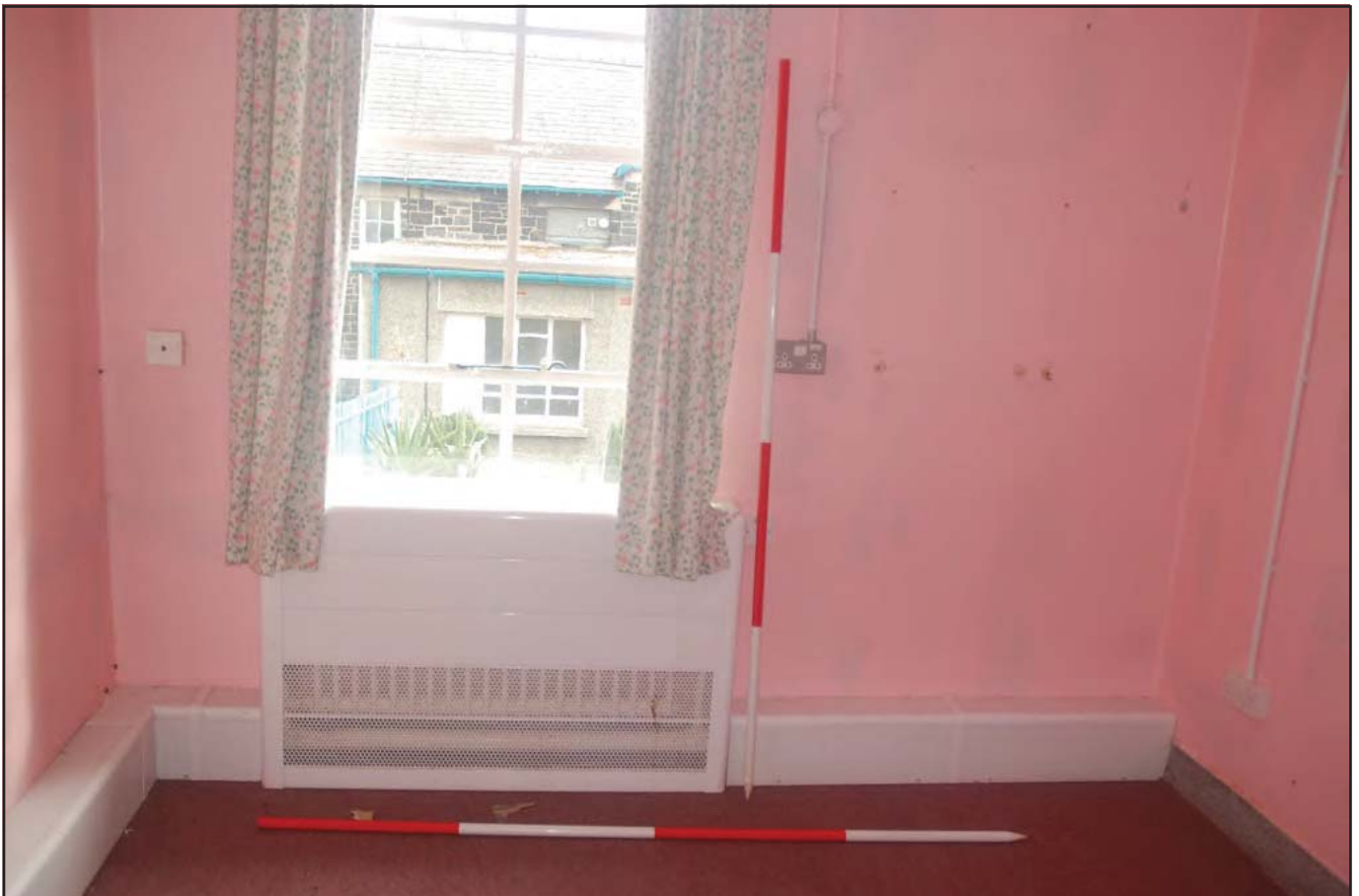
Plate 30: Short Stay Unit (Internal): View south of Room G06 detailing current use as a ward. Storage heater visible below original casement window, with boxed in plumbing (Scales: 2 x 2.0m)
