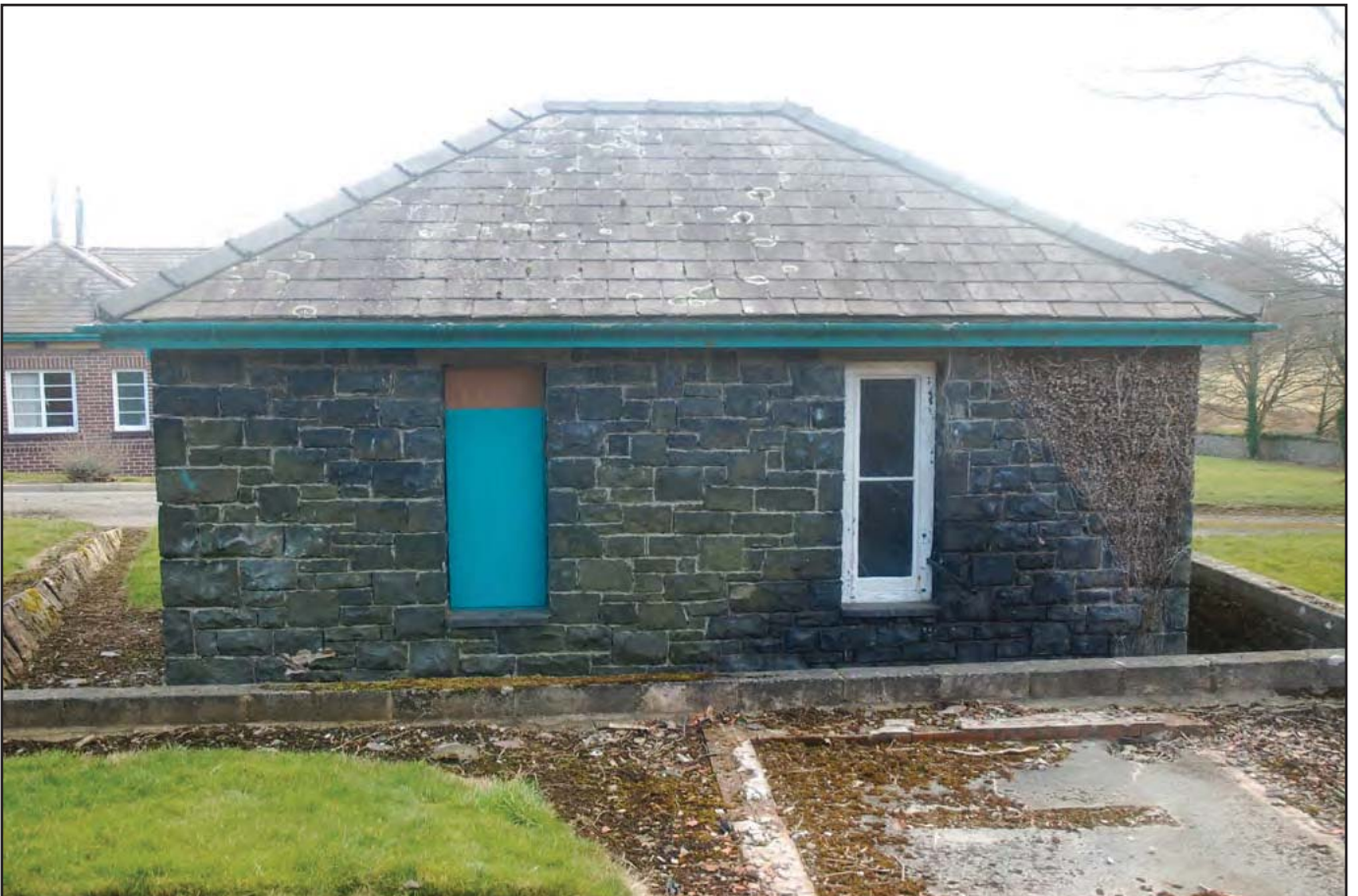
Plate 60: Generator Room: Northwest facing elevation detailing rear. This elevation represents the post-1914 extension, which has been benched into the slope. A later external platform has been built (bottom right of image), with brick surround that may have supported an upstanding piece of equipment. Note the rear of the Short Stay Unit to centre left of image.
