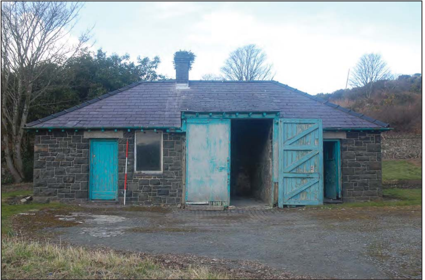
Plate 53: Garage - Southeast facing elevation; detailing main entrance via large panel and brace doors and two side entrances. Part of the original construction phase along with Long Stay Unit, Water Tower and Administration Block, with similar building detail including sub-rectangular stonework, stone lintel and quoin edging. (Scale: 1 x 2.0m)
