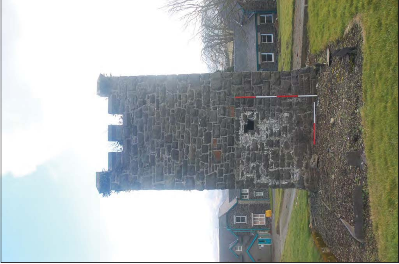
Plate 51: Water Tower - Northwest facing elevation detailing construction form, including crenellated capping and an internal buttress. Note the external slate defined area that appears to have functioned as a possible small garden area, note also the administration block in the left background and the Long Stay Unit in the right background (Scales: 2 x 2.0m).
