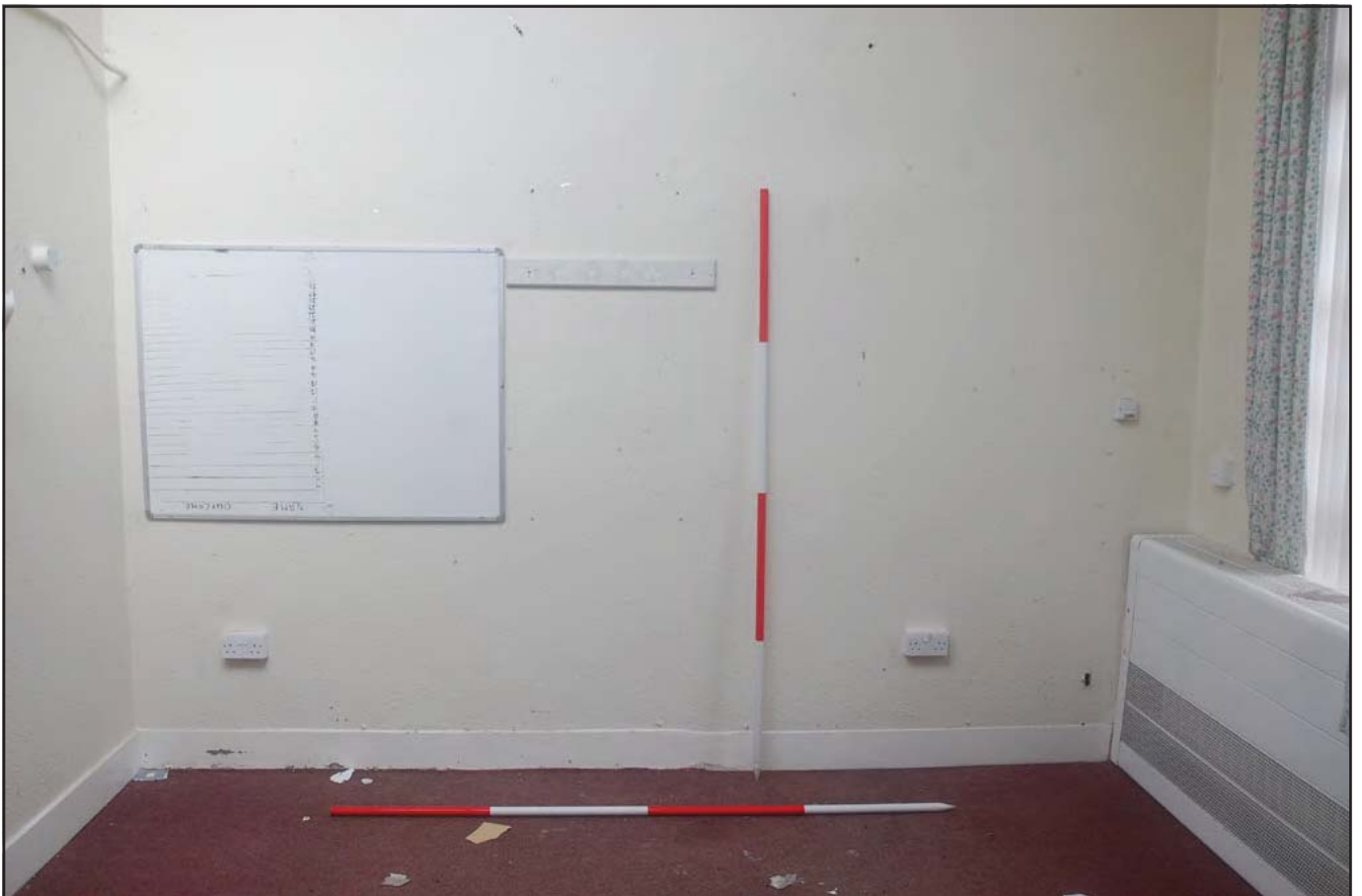
Plate 34: Short Stay Unit (Internal): View east of Room G10 detailing current use. Storage heater visible below original casement window, bullnose skirtings extant. (Scales: 2 x 2.0m)
