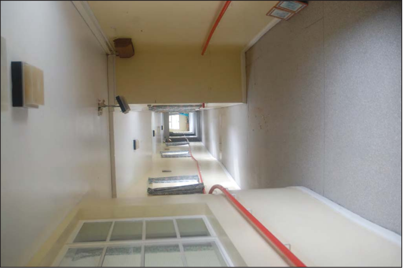
Plate 39: Link Corridor connecting Long and Short Stay Units (Internal): View southeast. Former exterior window of Room G12 visible in left foreground.
