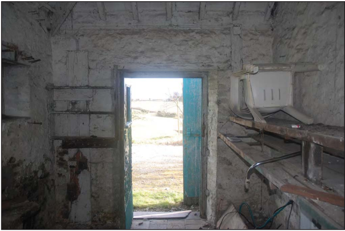
Plate 55: Garage (Internal): View south of side entrance room (cf. external view Plate 50) detailing interior finish and usage. Roughcast walls, whitewashed and exposed rafters visible. Various fittings also present facilitating it's use as a store.
