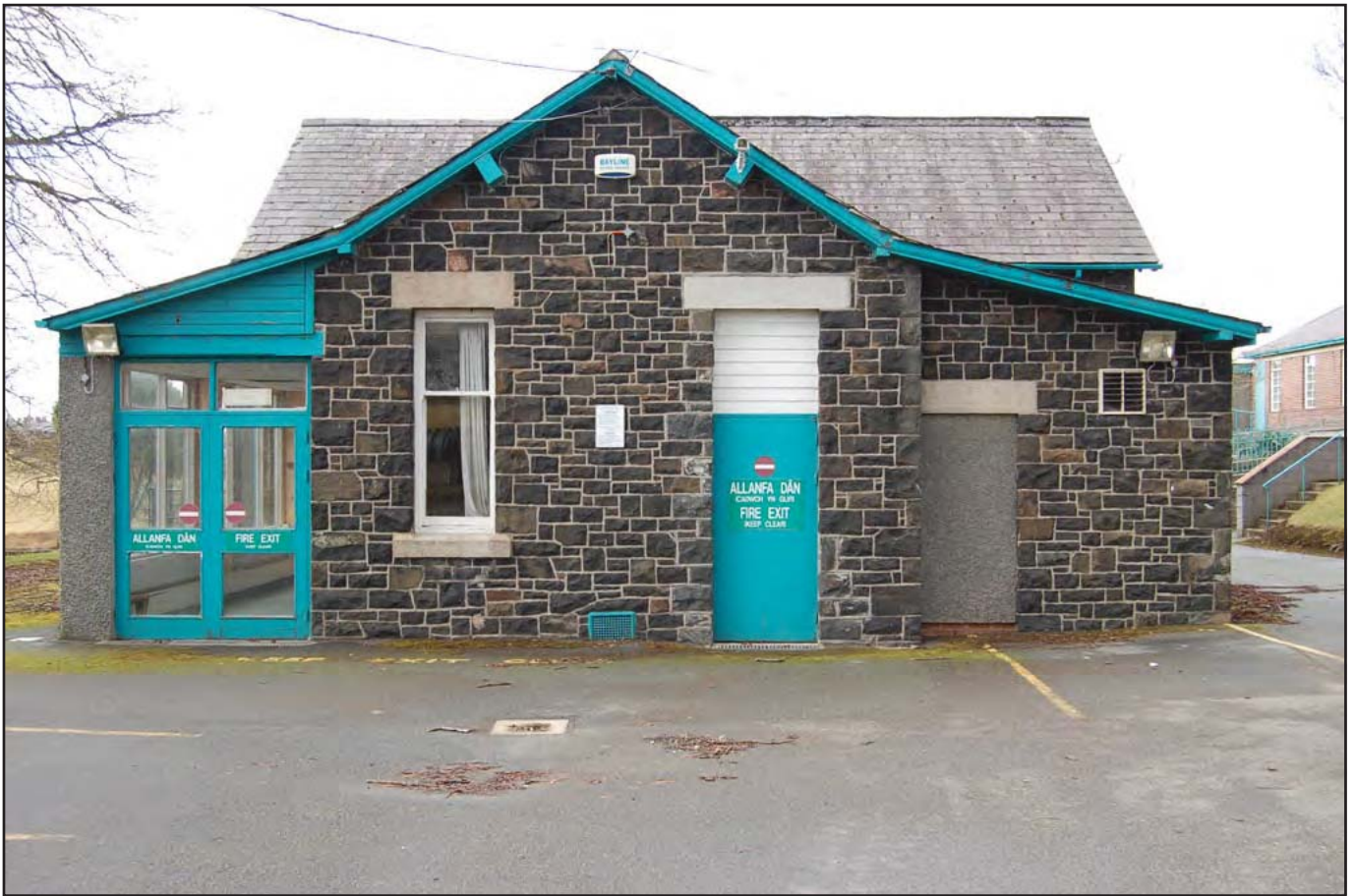
Plate 07: Long Stay Unit (External): Northeast facing elevation of early twentieth extension (Room G12), detailing the use of sub-rectangular stonework and quoin edging. The roof of the female wing (Room G11) is in the background.
