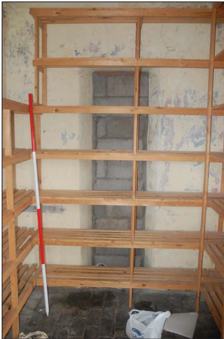
Plate 61: Generator Room (Internal) - View northeast of interior room, detailing decor and usage. Interior view of extension room. Note blocked window, visible from the outside in Plate 59. The floors are quarry tiles; the walls are rendered. Wooden shelving throughout room. (Scale: 1 x 2.0m)
