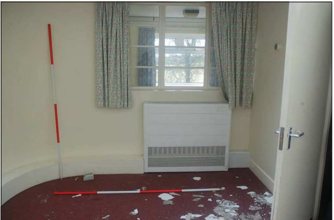
Plate 36: Short Stay Unit (Internal): View southwest of Room G12 detailing current use and original casement window fitting. Formerly a treatment room. Curved floor plan indicates former shape of the southwestern end of the building now disguised by the link corridor (visible through the casement window). Particleboard door in use rather than original panelled door seen elsewhere within the structure as room size was reduced and a new partition fitted. (Scales: 2 x 2.0m)
