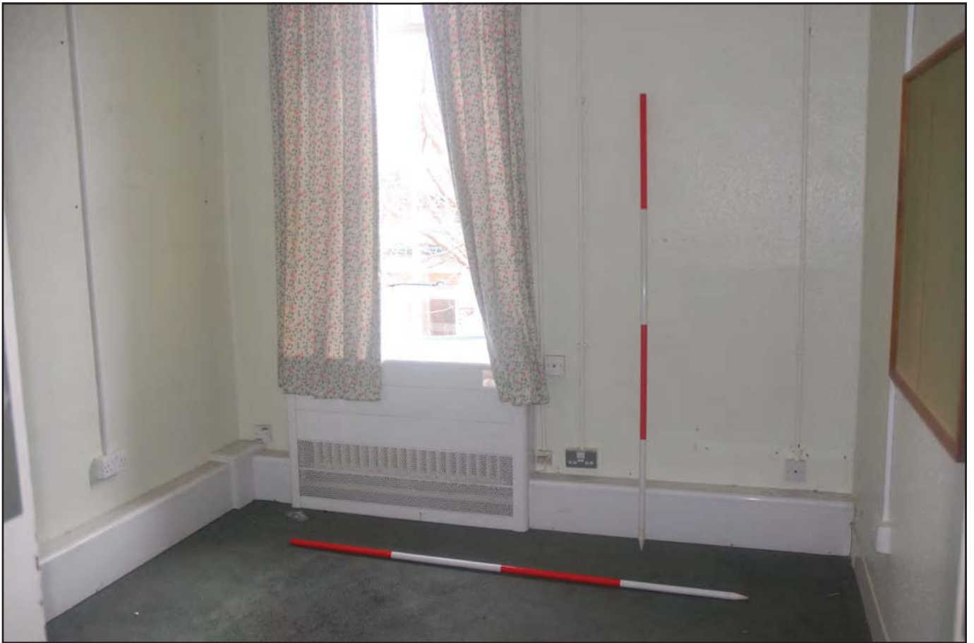
Plate 33: Short Stay Unit (Internal): View southeast of Room G09 detailing former use as a ward. Storage heater visible below original casement window, with boxed in plumbing (Scales: 2 x 2.0m)
