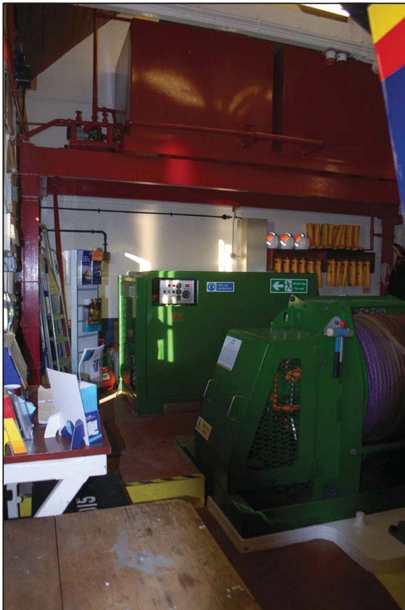
Plate 14 – Hydraulic winding gear and generator
