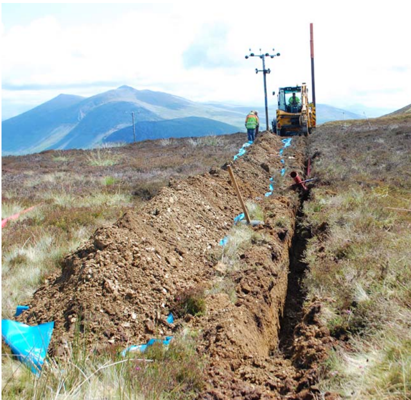
Below: Plate 01 - Cable trench excavation looking toward pole 25A. View from the west
