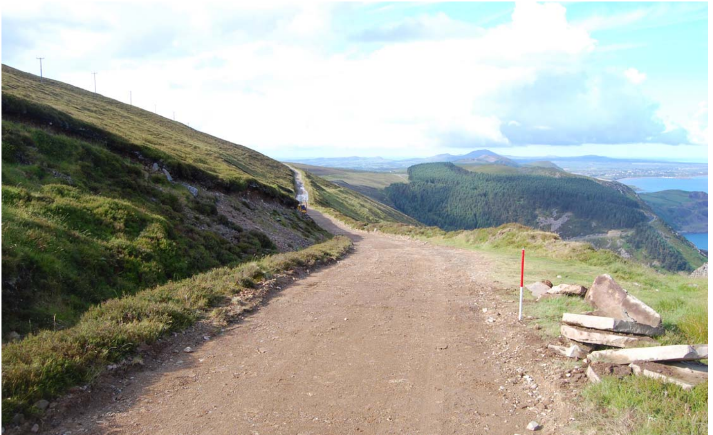
Above: Plate 04 - Re-instated section of trackway with bur- ied cable below. View from the north. Scale 1m
