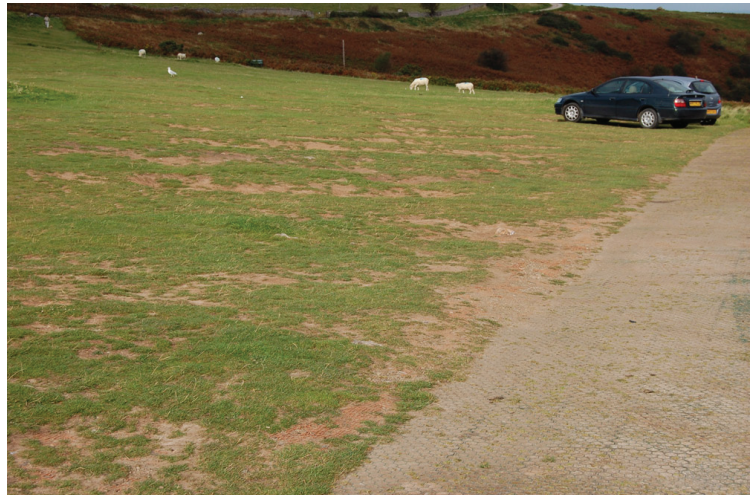
Plate 2: Erosion on site of new car park, from SE
