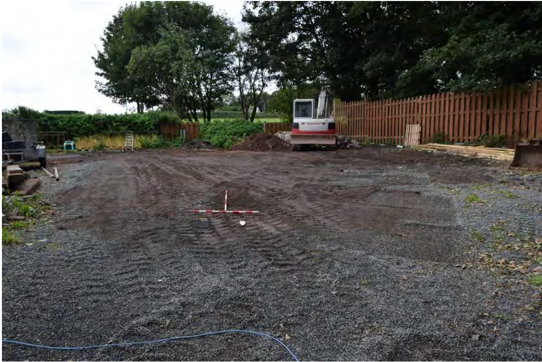
Photo 11: SSW facing shot showing the proposed development area after the trenches had been backfilled. 2m & 1m scales.
