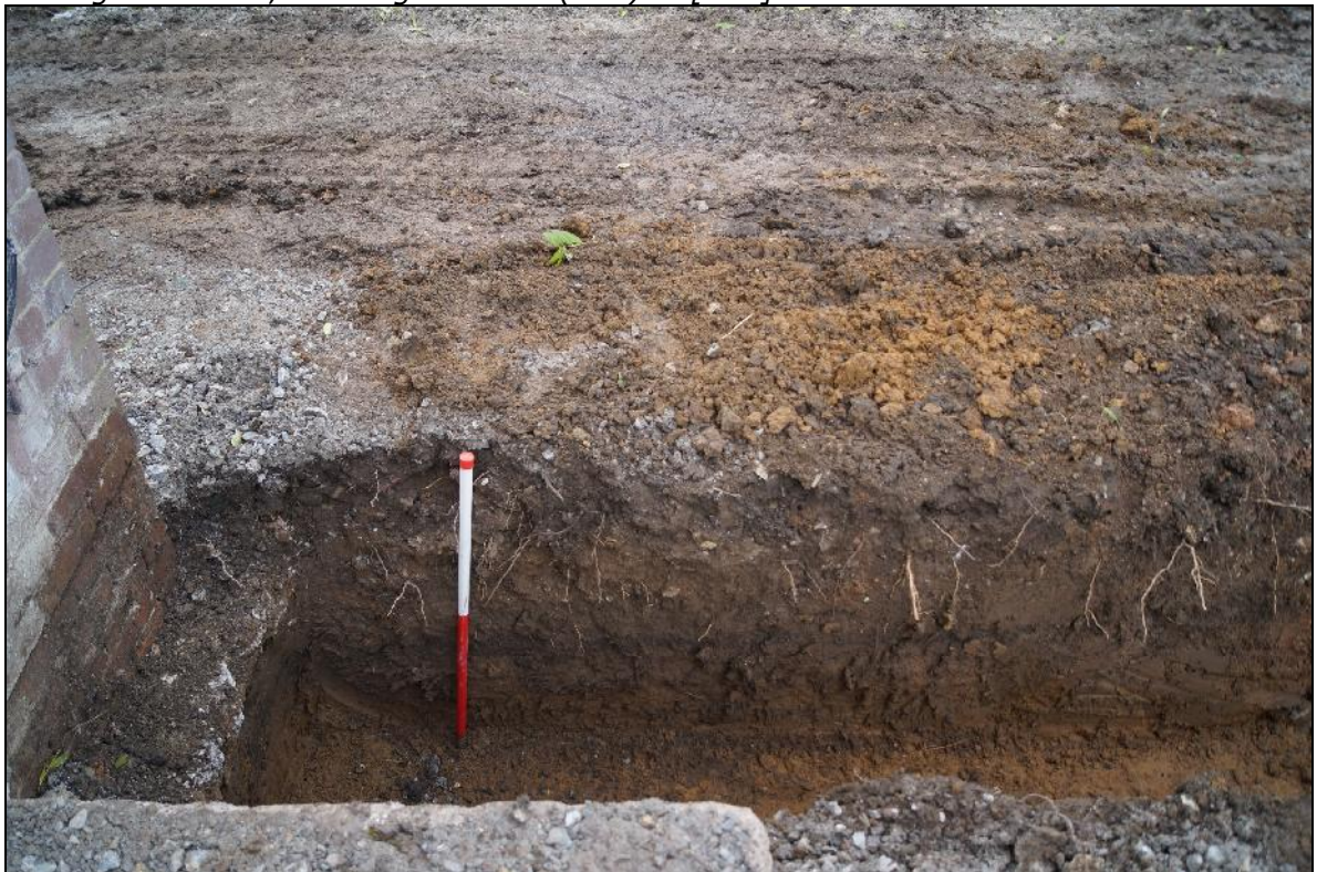
Plate 12: RCH2018_112, Southern end of the western part of the foundation trench, looking west northwest.
