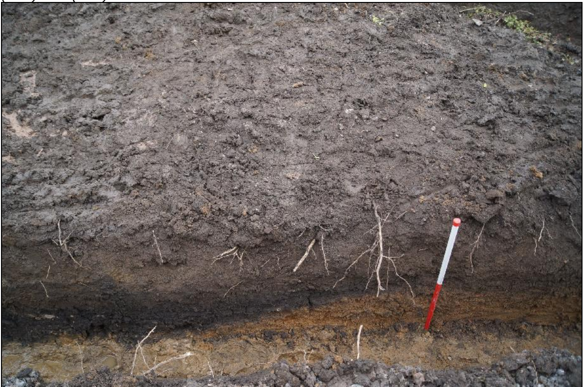
Plate 10: RCH2018_110, Northern part of the foundation trench, looking northeast with the eastern part of (007) and [008] clearly visible in the northern section, overlain by (002) and (001)
