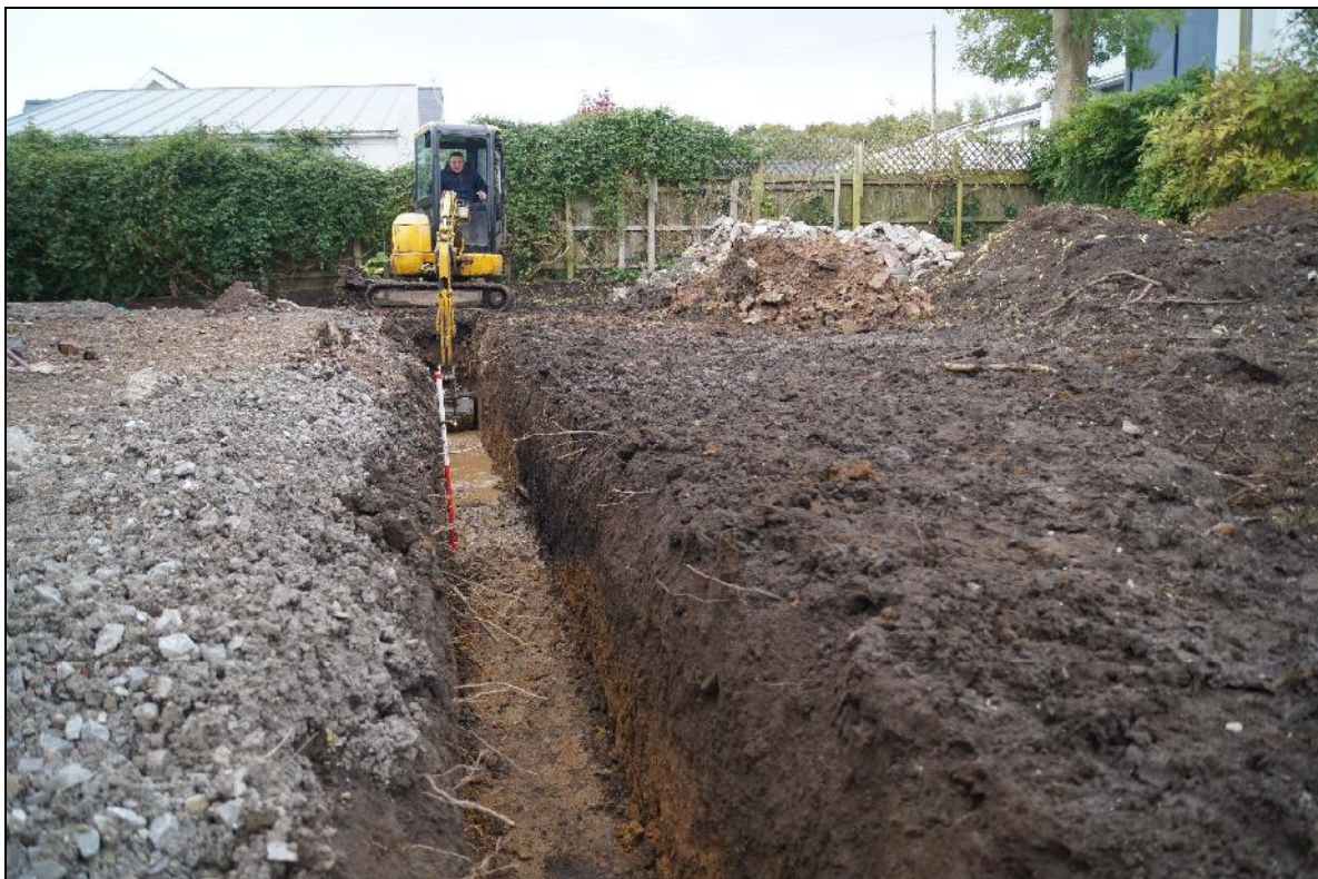
Plate 4: RCH2018_104, Northern part of the foundation trench, looking west northwest, with (007) clearly visible in the northern section.
