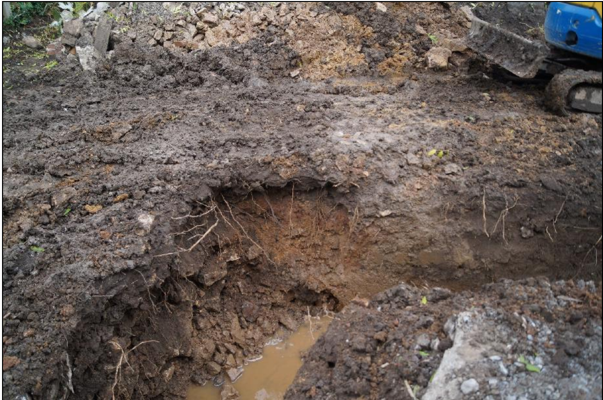
Plate 7: RCH2018_107, Northern corner of the foundation trench, looking north, showing (001) overlying (003) and [004].
