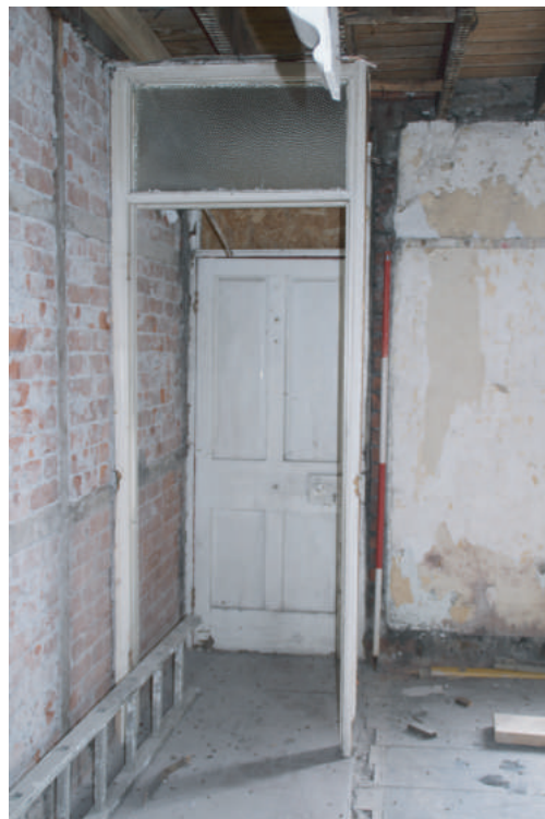
Plate 22. London House, Beach Road, Penclawdd. Internal view of House doorway. Looking north.
