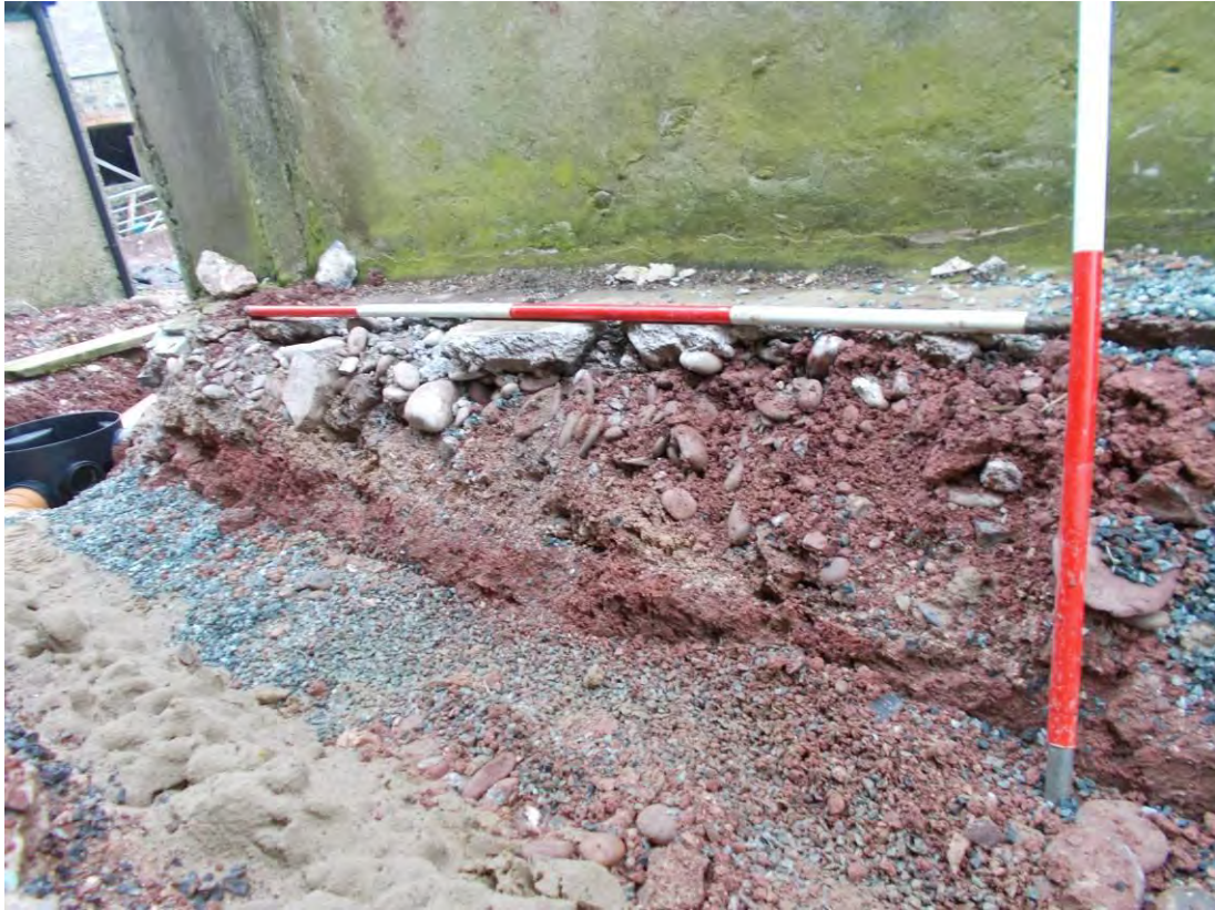
Photo 93: Service trench excavations - trench through passageway between Farmhouse and Cart Shed, north facing section. 1m & 2m scales.
