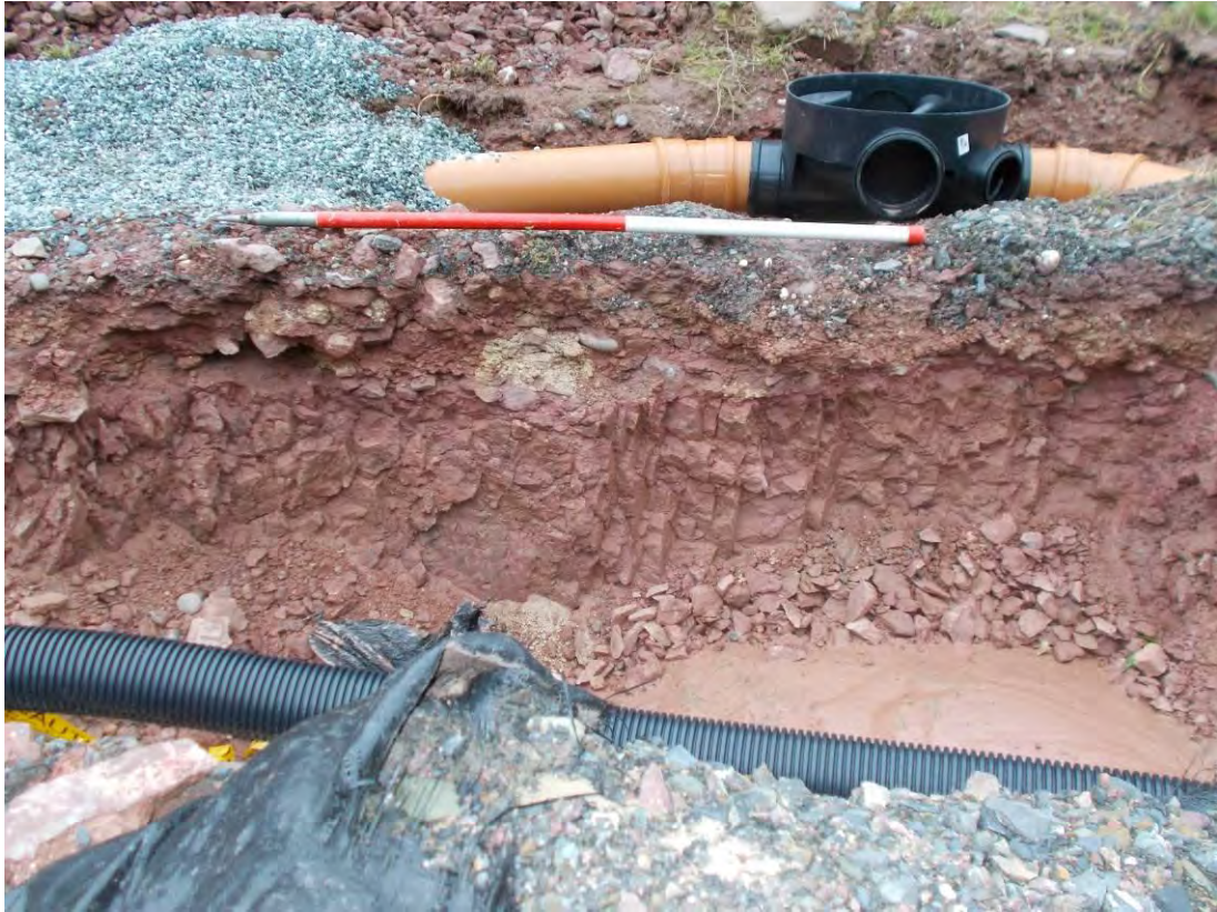
Photo 91: Service trench excavations - trench through farmyard to the south of the Farmhouse, north facing section. 1m scale.
