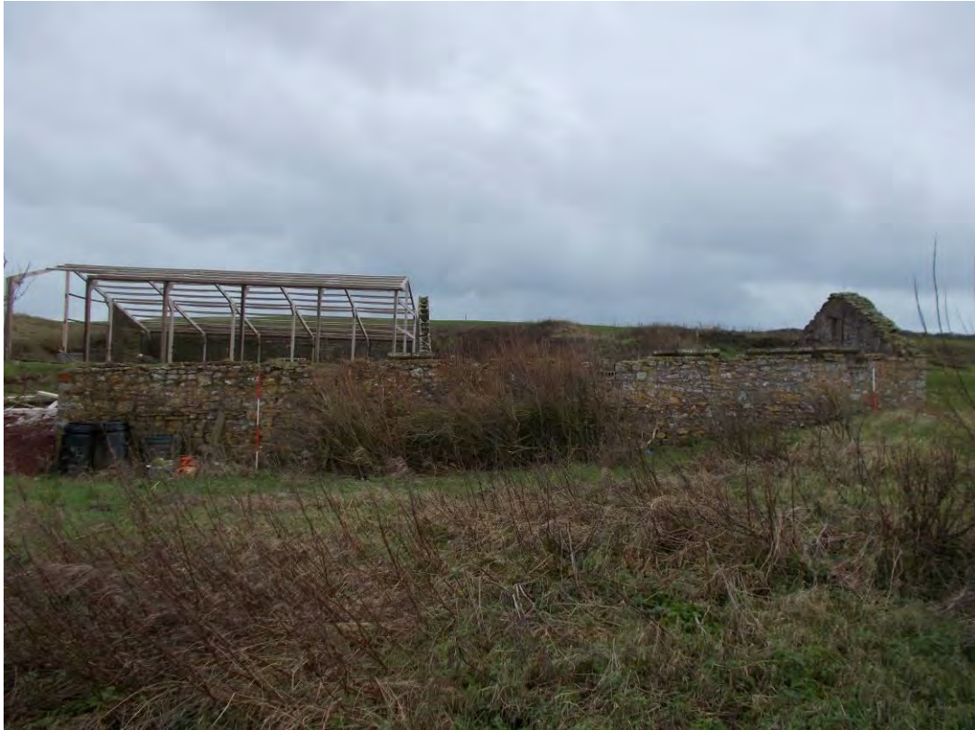
Photo 87: Detached ruinous structure at the western end of the farmstead, external face of northern elevation. Straw & Implement building to the rear. Looking South. 1m & 2m scales.
