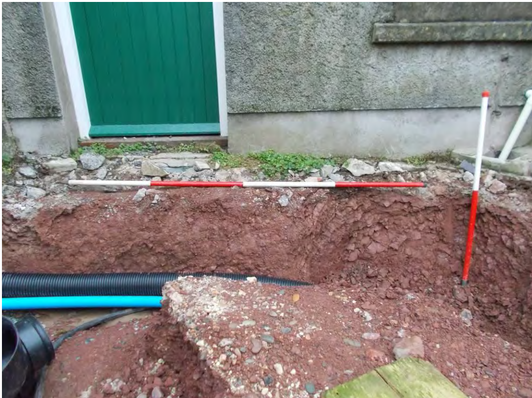
Photo 92: Service trench excavations - trench through farmyard to the south of the Farmhouse, south facing section. 1m & 2m scales.
