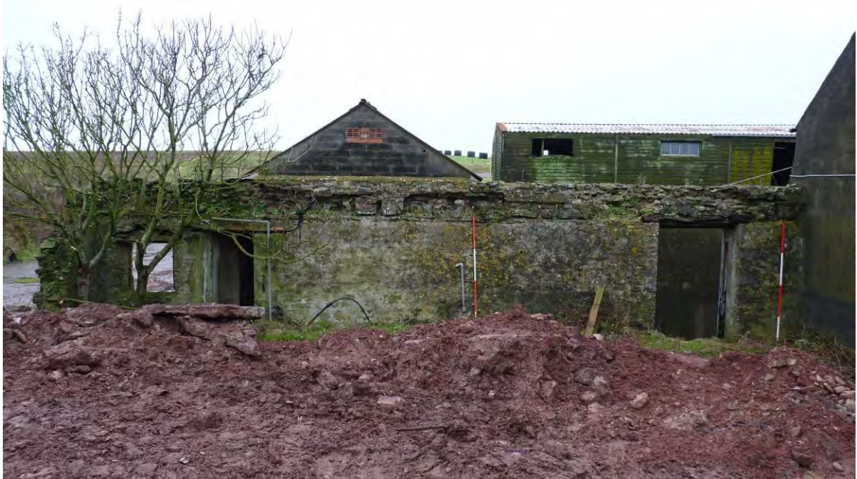
Photo 85: Ruinous structure, attached to the west side of the Farmhouse, internal face of wall. Looking North. 2m scales.
