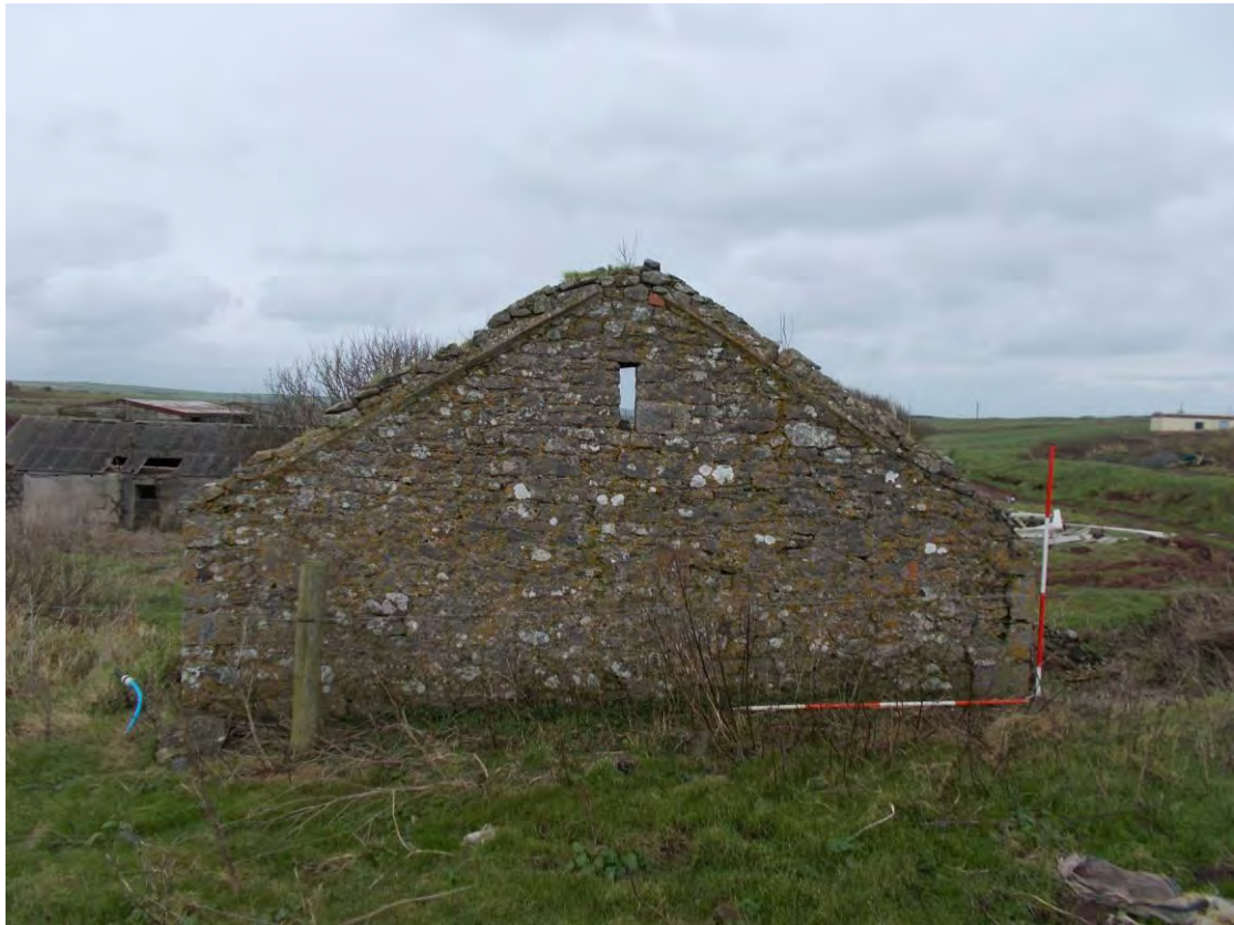
Photo 89: Detached ruinous structure at the western end of the farmstead, western (gable) elevation. Looking East. 2m scales.
