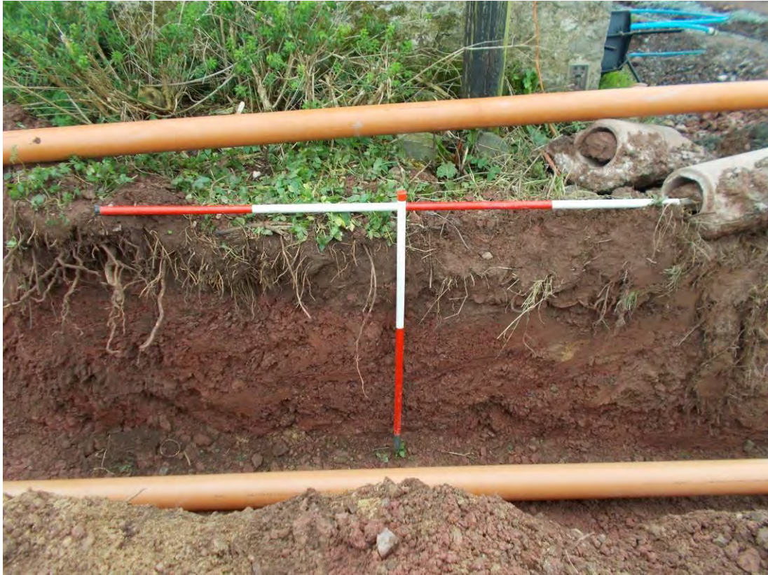
Photo 97: Service trench excavations - trench through eastern area in front of the Cow Shed, east facing section. 1m & 2m scales.
