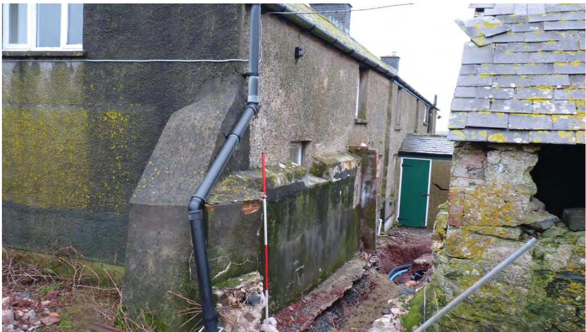
Photo 6: The Farmhouse, passageway between the farmhouse on the left and the Cart Shed on the right. Looking Northeast. 2m scale.
