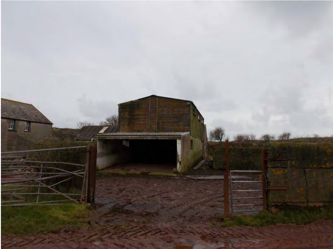
Photo 79: The Milking Parlour, Building 2, eastern elevation and circular animal enclosure. Looking West-southwest.
