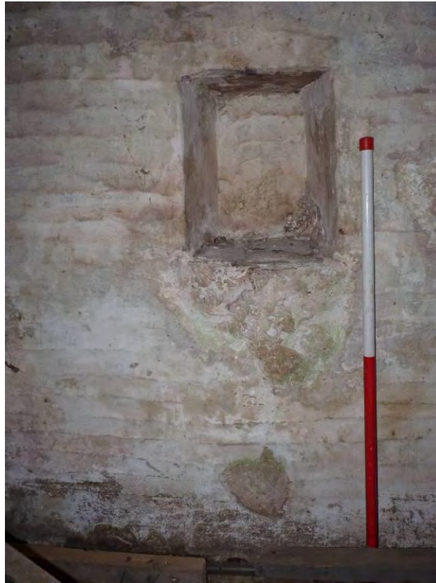
Photo 69: The Cart Shed, interior, southern room. Recess in southern gable wall. Looking South. 1m scale.
