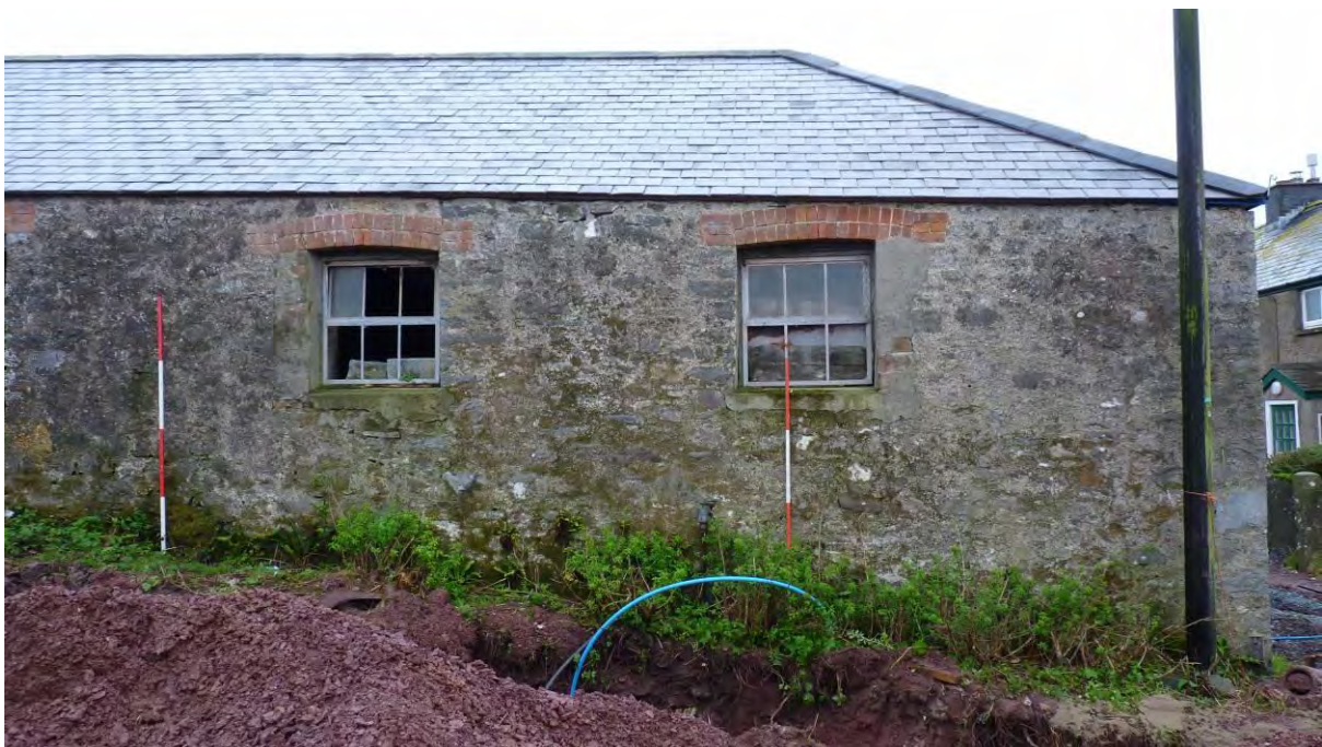
Photo 54: The Cow Shed, eastern elevation, windows of northern southern room. Looking West. 2m scales.
