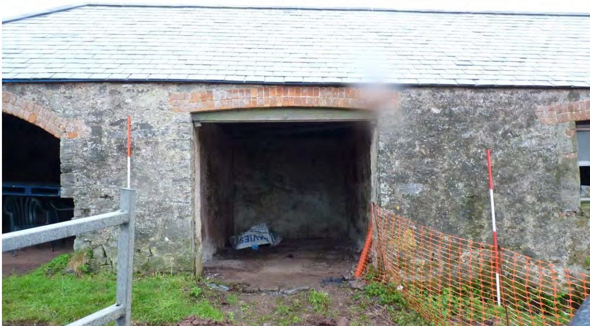
Photo 52: The Cow Shed, eastern elevation, entrance to central room. Looking West. 2m scales, in 0.5m segments.
