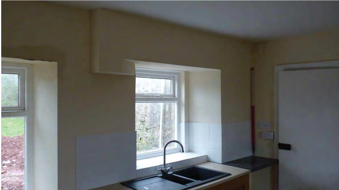
Photo 18: The Farmhouse interior, Room 3. Showing protruding wall and lintel above inserted kitchen units. Looking Southwest. 1m scales.
