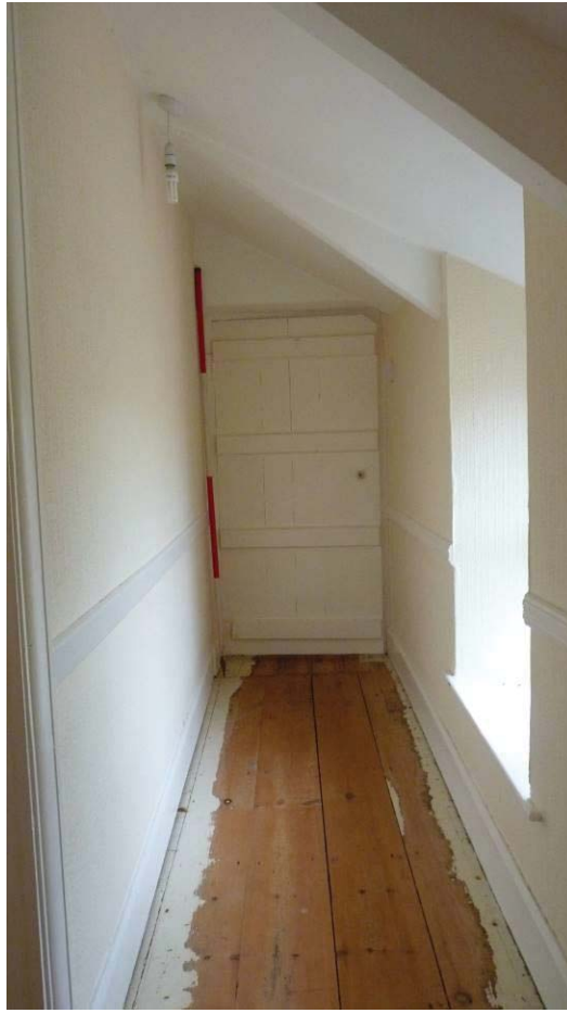
Photo 23: The Farmhouse interior, 1 st floor, corridor behind Room 7. Looking West. 2m scale.
