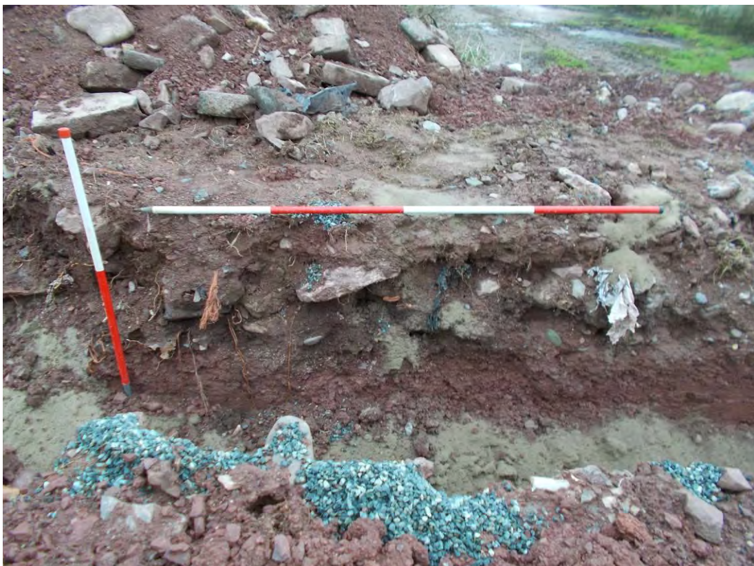
Photo 96: Service trench excavations - trench through western area, south facing section. 1m & 2m scales.
