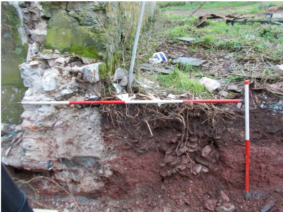
Photo 94: Service trench excavations - trench immediately to the west of the Cart Shed, showing wall [107] and drain [109]. North facing section. 1m & 2m scales.
