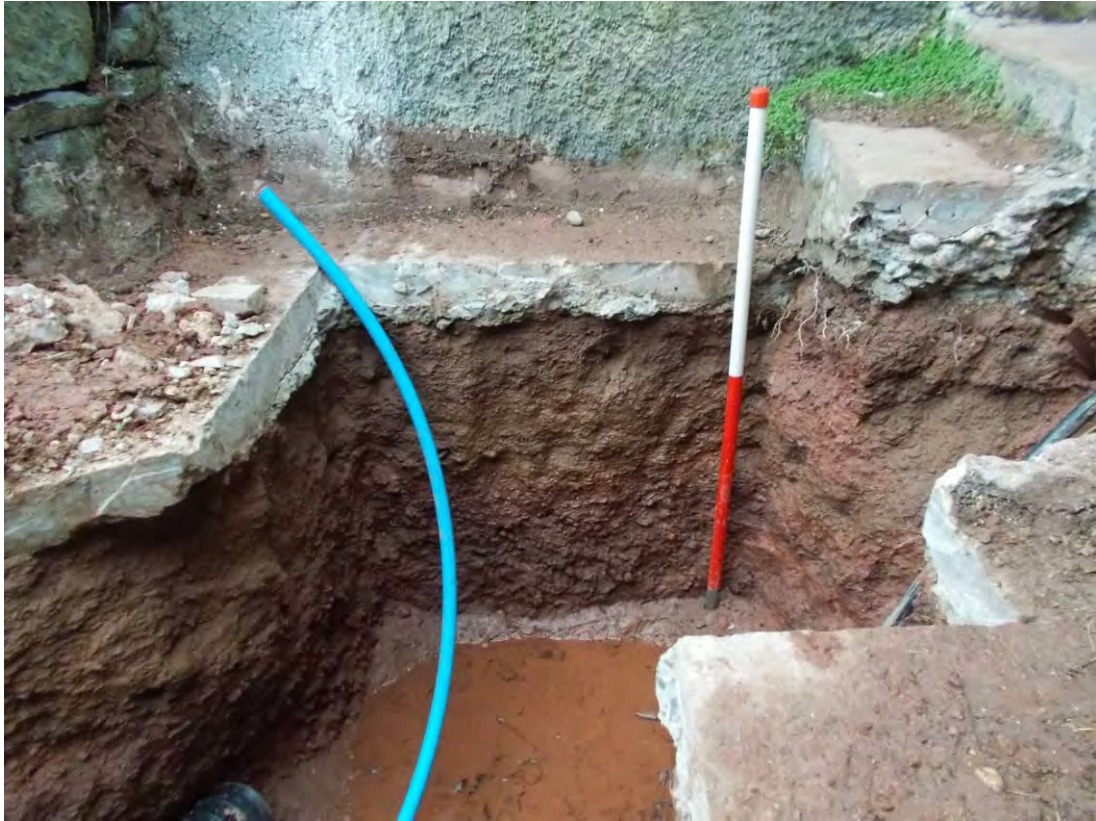
Photo 99: Service trench excavations - trench through northern area immediately to the northwest of the Farmhouse. North facing section. 1m scale.
