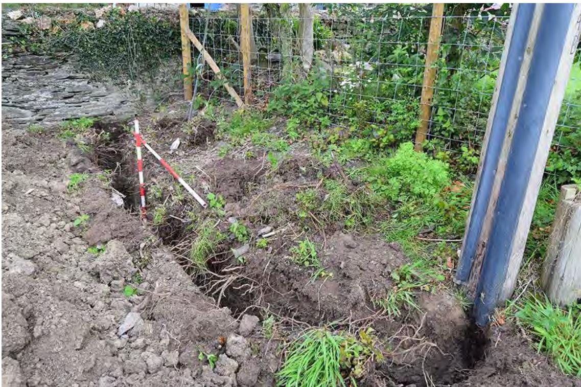
Plate 2: North facing view of trench excavation on the south-eastern side of the development (1m and 2m scale).
