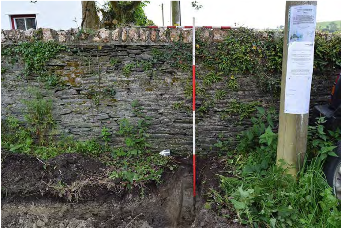
Plate 3: View of trench excavation on western side of garden/field wall (2m & 1m scale).
