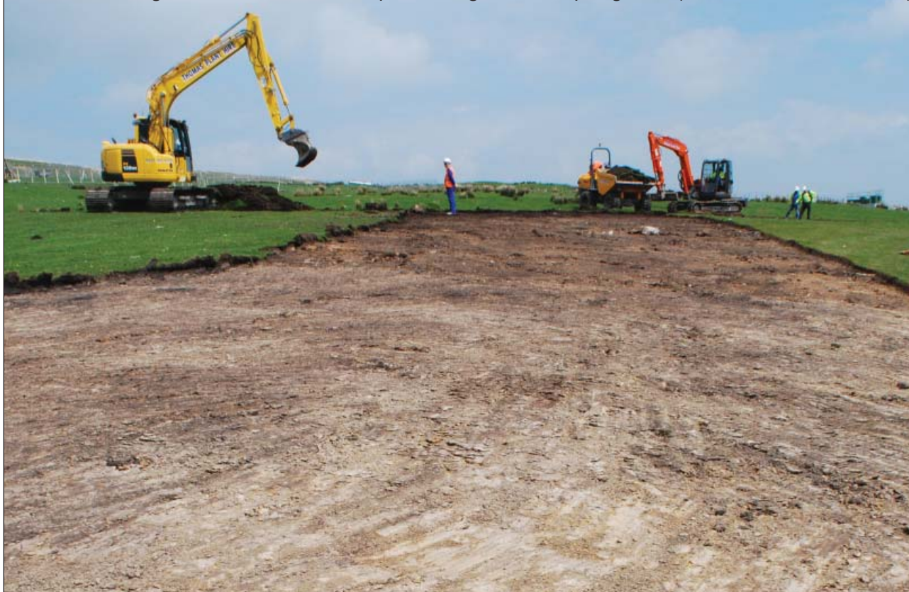
Plate 3: Working shot of the earthworks processing and stockpiling area (view from the Southeast)
