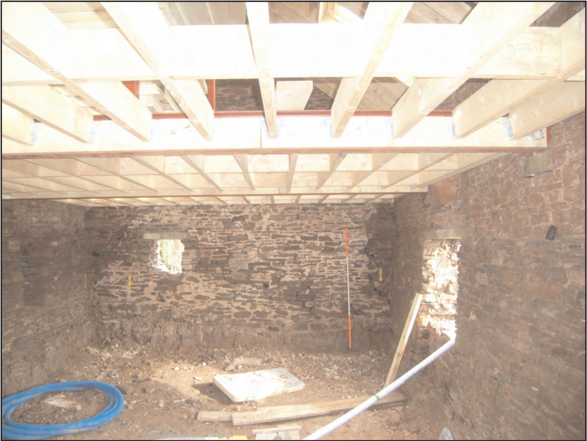
Plate 9 North gable interior showing footings resting on ridges of bedrock, looking north-east
