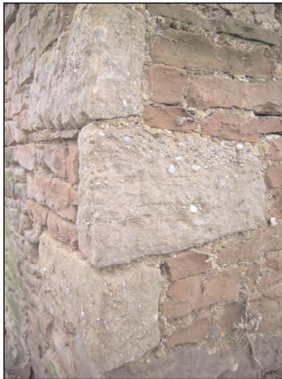
Plate 15 Corner of north gable wall showing Sandstone Conglomerate quoins at upper level, looking south
