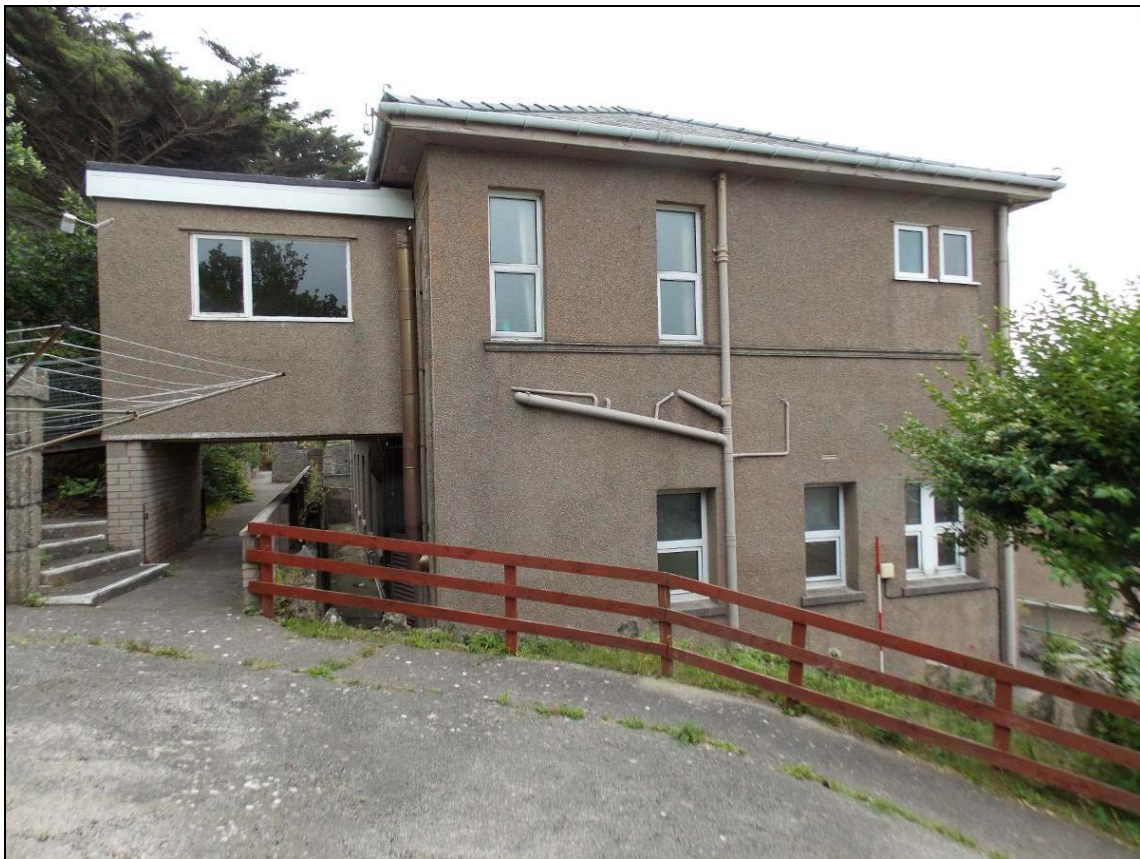
Plate 5: Detail of the projecting walkway to the north, looking east (scale 2m).
