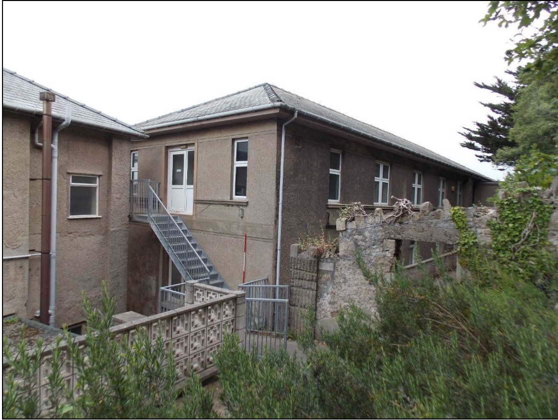
Plate 8: General view of the north and east elevations, looking south-west (scale 2m).
