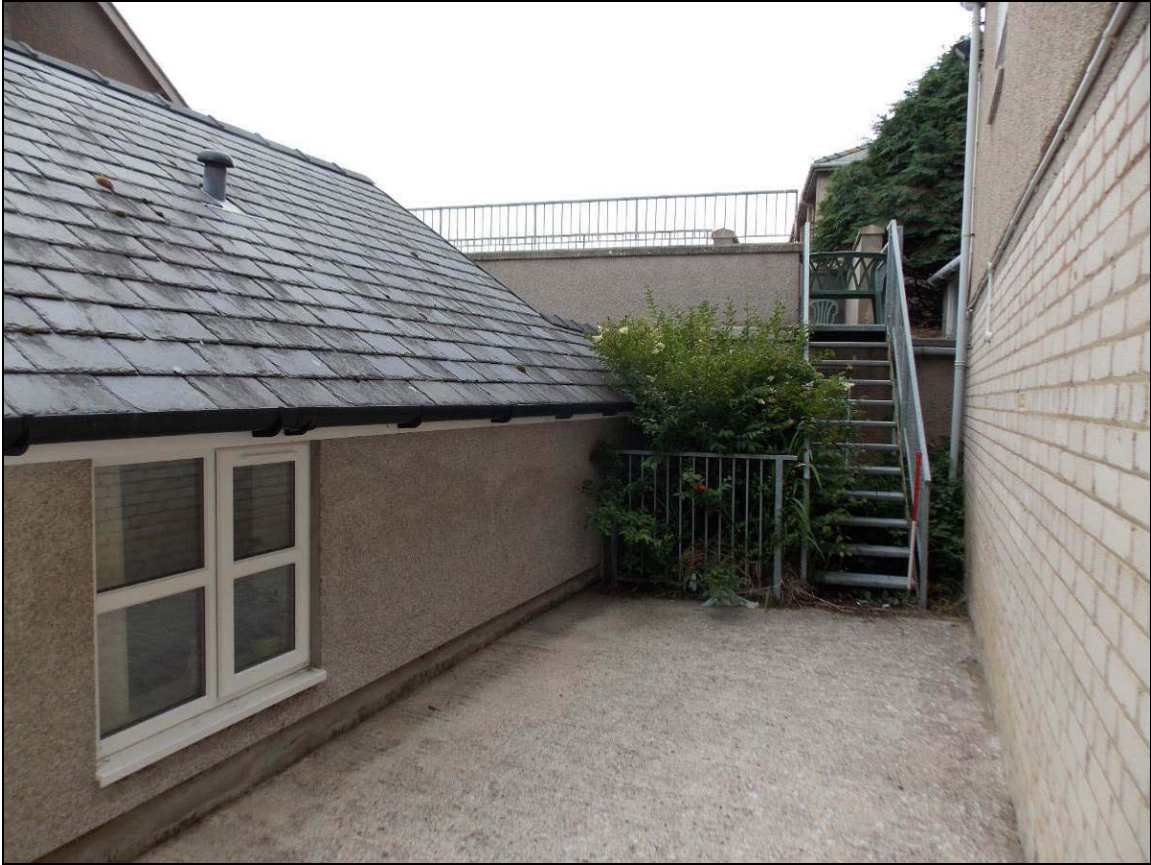
Plate 60: Western end of the north elevation with stairs to walkway, looking west (scale 1m).
