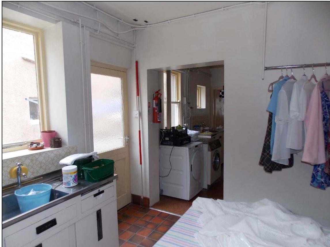
Plate 46: Inserted doorway within the dividing wall of the laundry, looking south-east (scale 2m).
