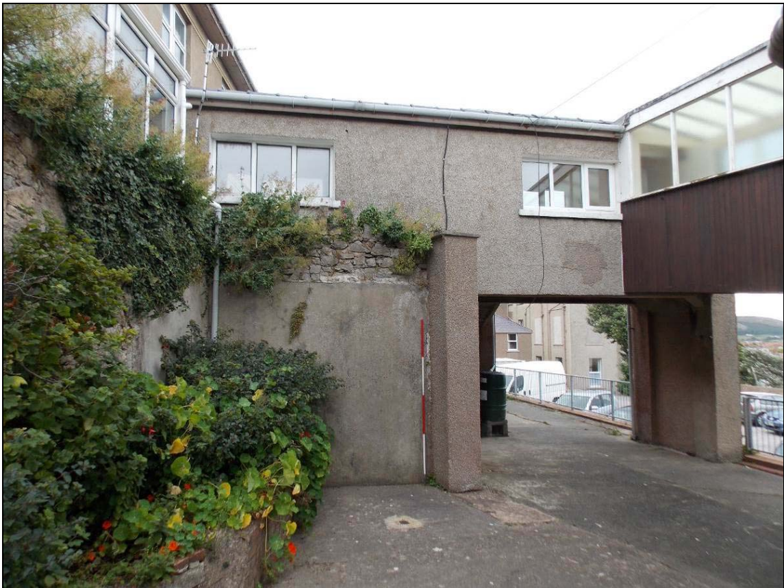
Plate 34: West elevation of the walkway linking Buildings A and B, looking east (scale 2m).
