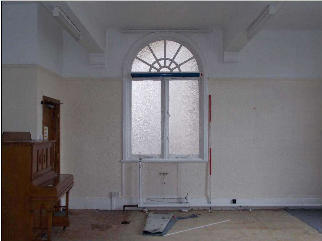
Plate 14: Detail of window opening with semi-circular arched head, looking east (scale 2m).
