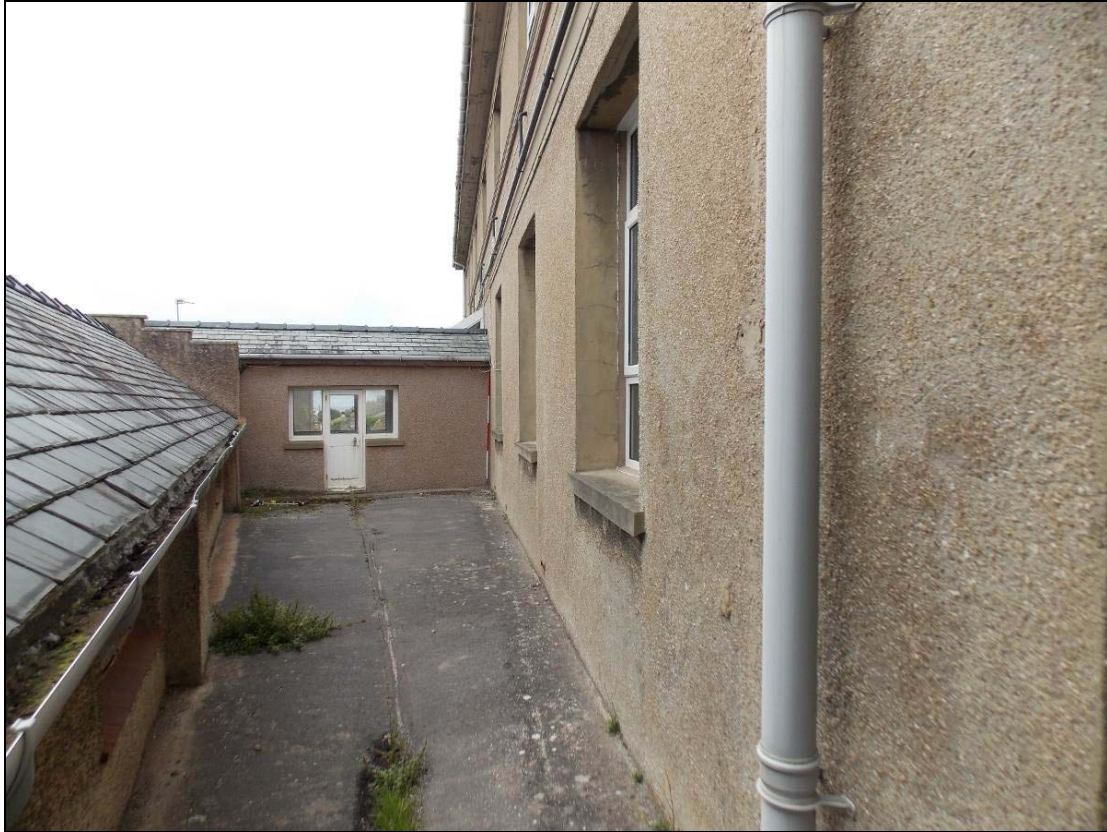
Plate 10: Eastern side of the first floor of the south elevation, looking west (scale 2m).
