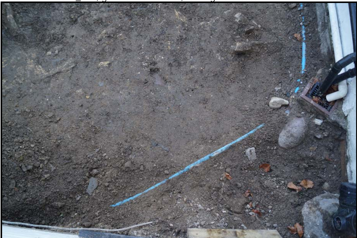
Plate 12: RCL2017_112, the modern water pipe (002) and [003] at southwestern end of site, looking northeast.
