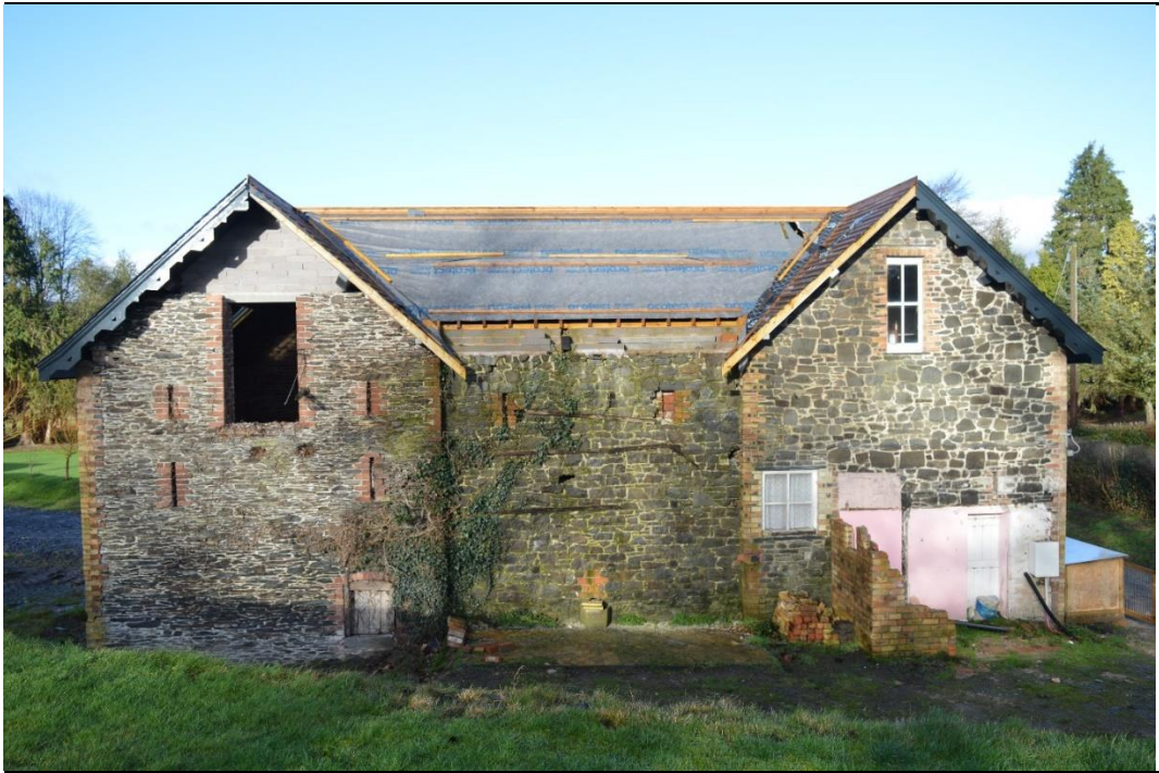
Figure 3. The rear of the Coach House showing the difference in building stone utilised in each gable. CPAT image 4592-0015.
