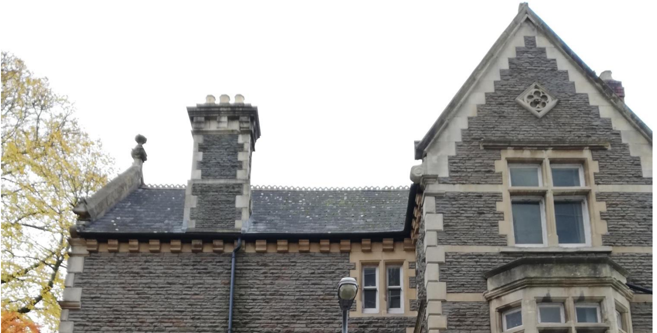
Plate 12: Roof details to 29 Cathedral Road including stone chimney with quoins, natural slates, decorative ridge tiles.
