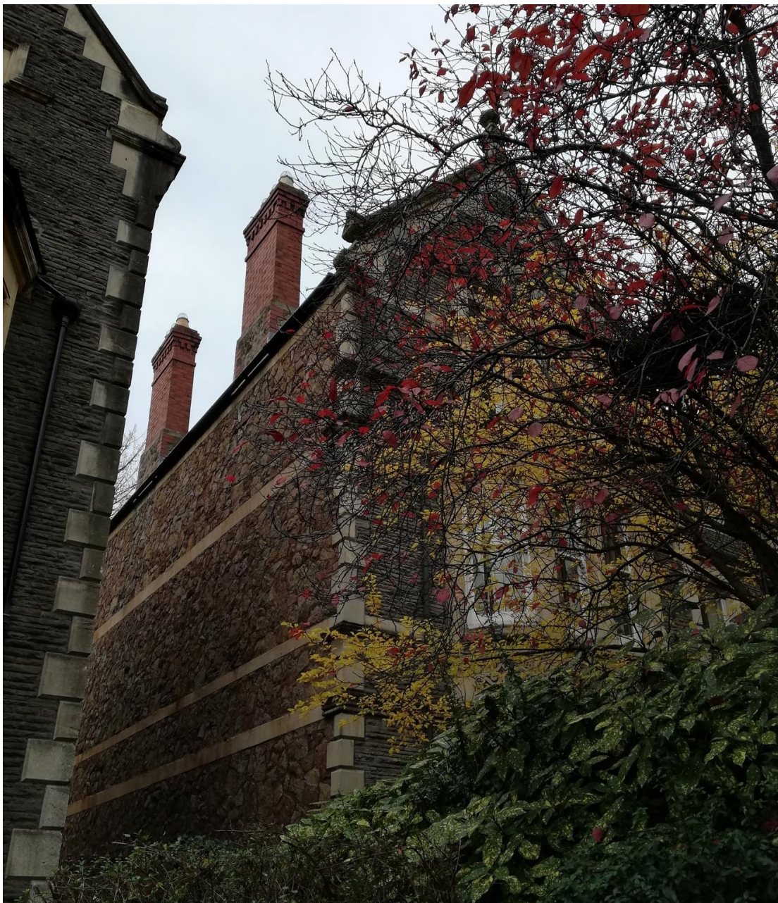
Plate 8: S elevation of 29 Cathedral Road, showing variety of stone use and coursing with brick chimneys
