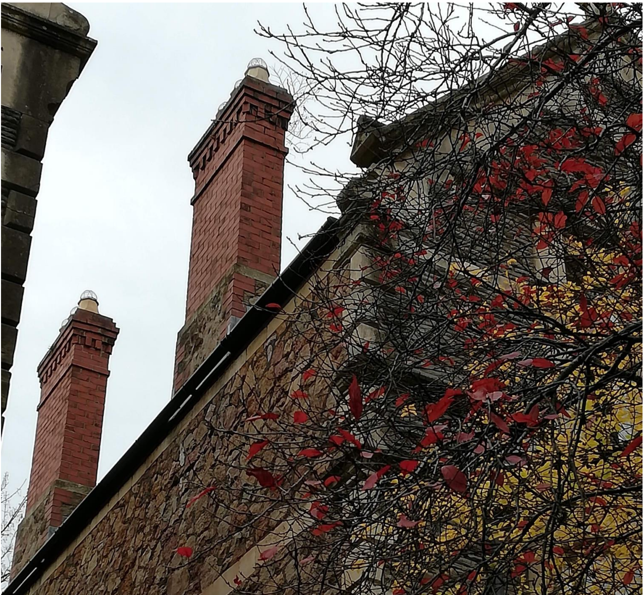
Plate 11: Details of roof to 27 Cathedral Road, including brick and stone chimneys and verge details.
