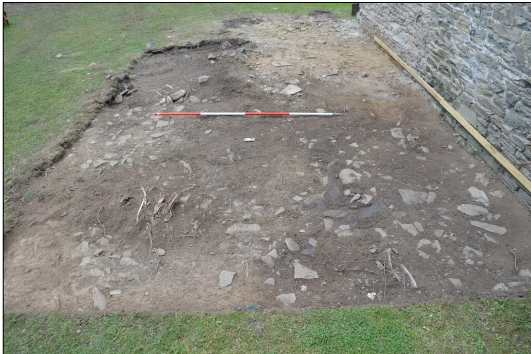
Fig. 3 Excavated footprint for the proposed extension, Peace Cottage. Viewed from the west. Photo CPAT 4524-0001
