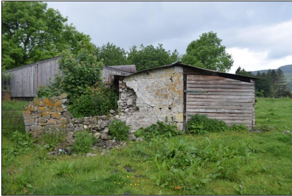
Fig. 15: View of the outbuilding to the north of the cottage, from the east. Photo CPAT 4653-0006
