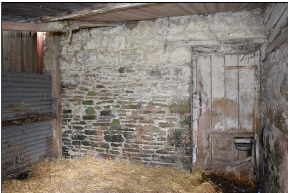
Fig. 6: The former garden wall within the outbuilding, showing the added courses. CPAT 4653-0005
