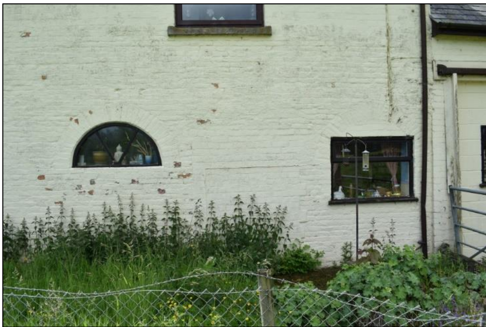
Fig. 12: The arched openings in the north wall of the cottage, the one to the right partially blocked. Photo CPAT 4653-0046
