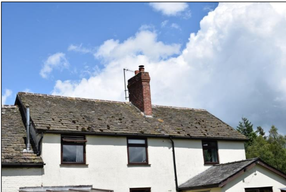
Fig. 10: The stone roof tiles on the south side of the cottage. These were no doubt reused after the roof height of this part was raised. Photo CPAT 4653-0059
