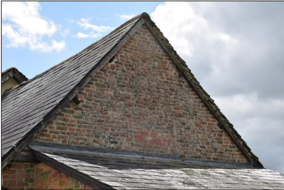
Fig. 9: The western gable of the cottage, probably a surviving portion of an earlier version of the building, showing its appearance and roof line. The north side, to the right, has stone roof tiles while the south side is slated; the same is true of the rest of the cottage. Photo CPAT 4653-0054
