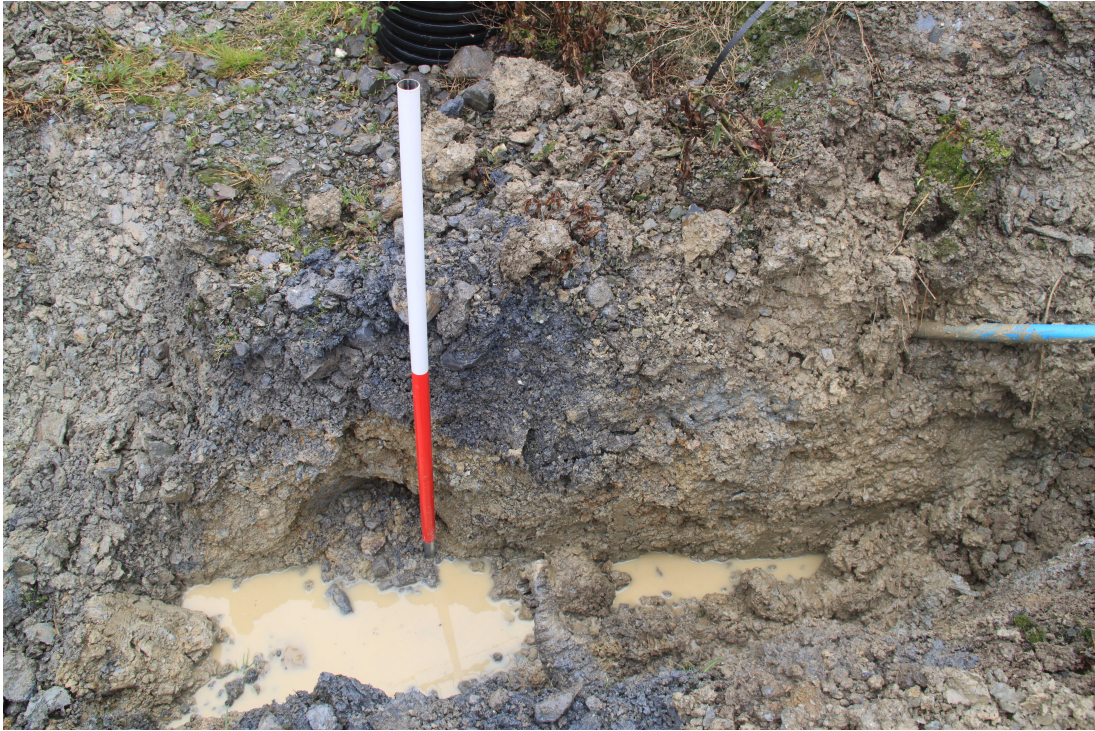
Plate 5 - AD007-1_005 - Cut of existing, disused service conduit.
