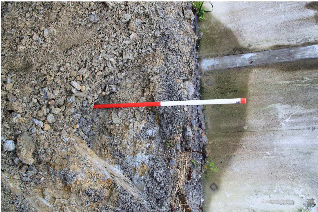
Plate 4 - AD007-1_004 - View north-west, showing clayey subsurface with stone scalping cover. Milking parlour behind.
