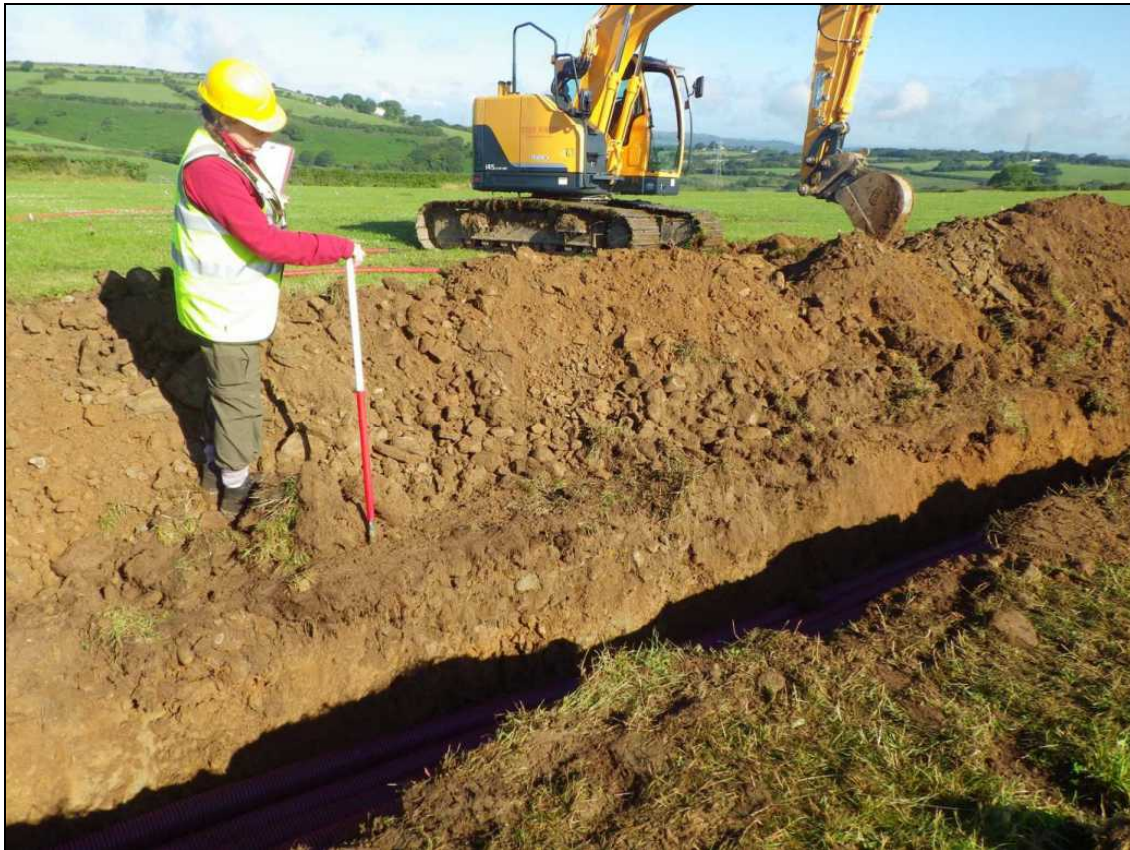
Plate 5: PFL2014_105, the main cable trench showing cables laid at SN5347708352, looking northwest.
