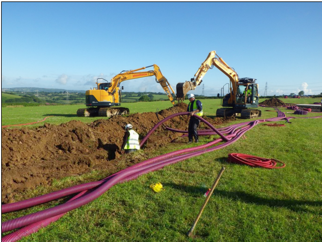
Plate 4: PFL2014_104, the main cable trench being cut at SN5350908619, at the same time as spur trenches are opened and cable-laying is undertaken. Looking northwest.
