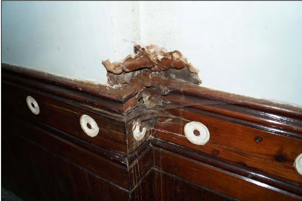
Plate 118: BTC2017_118, wet rot in the outer lobby panelling, looking southeast. Note the decorative, white-painted roundels, which feature throughout the chapel.
