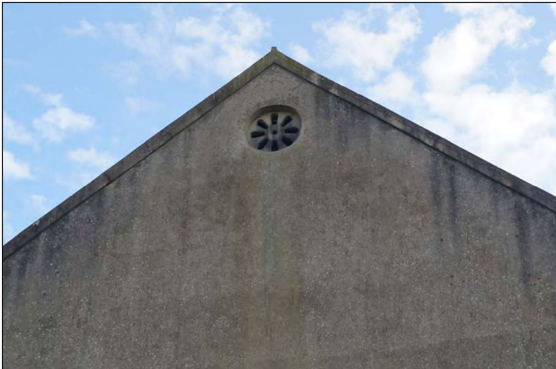
Plate 14: BTC2017_014, A ventilation aperture in the peak of the north elevation of the chapel, looking south.
