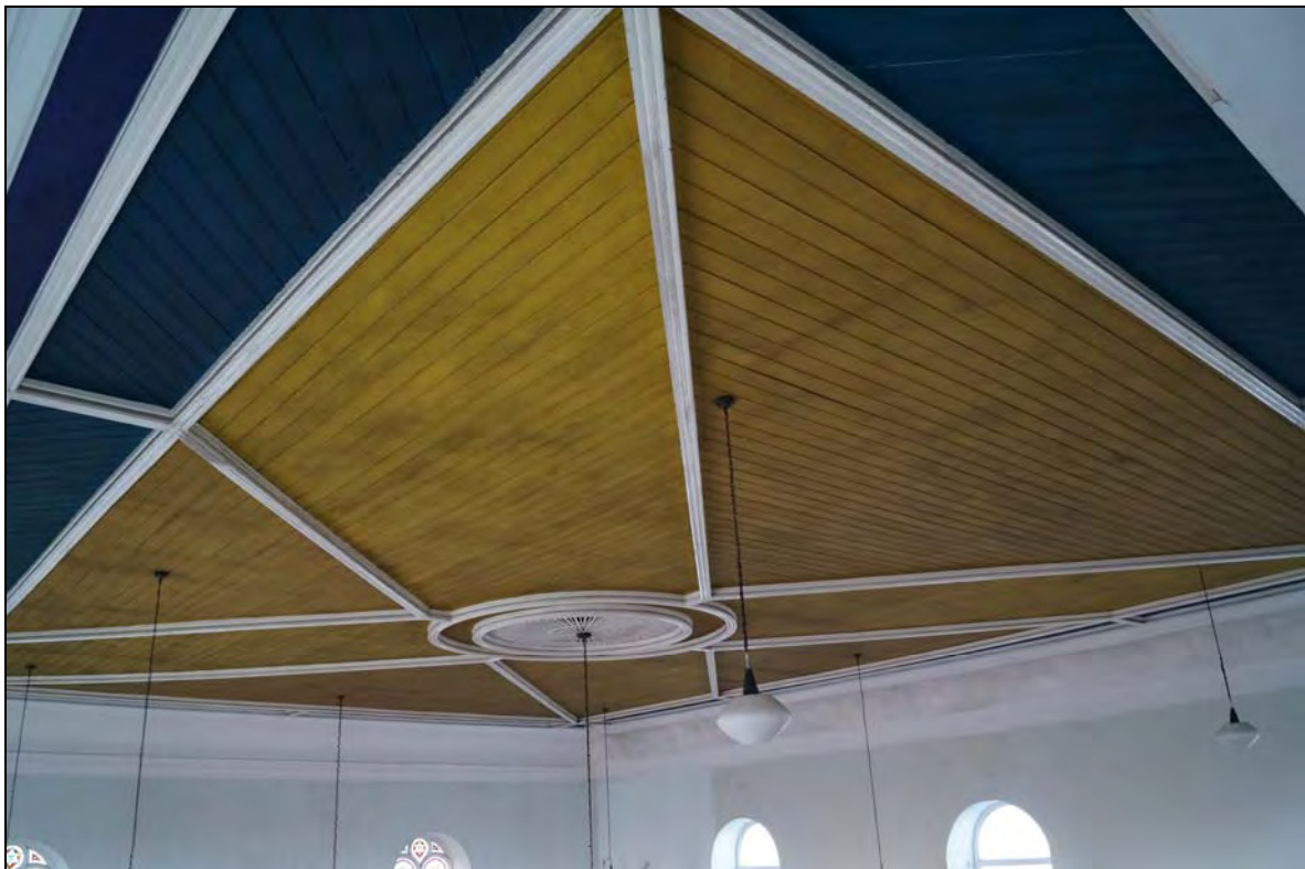
Plate 91: BTC2017_091, a view of the chapel ceiling from the gallery, looking northeast.
