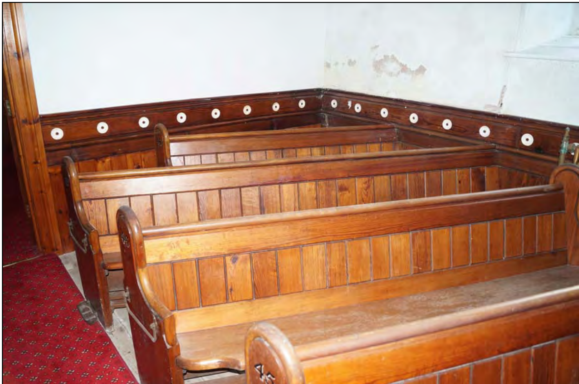
Plate 119: BTC2017_119, the pews in the southwest corner of the chapel. The furthest pew has been truncated to fit into the new layout created when the inner lobby was added. Looking southwest.
