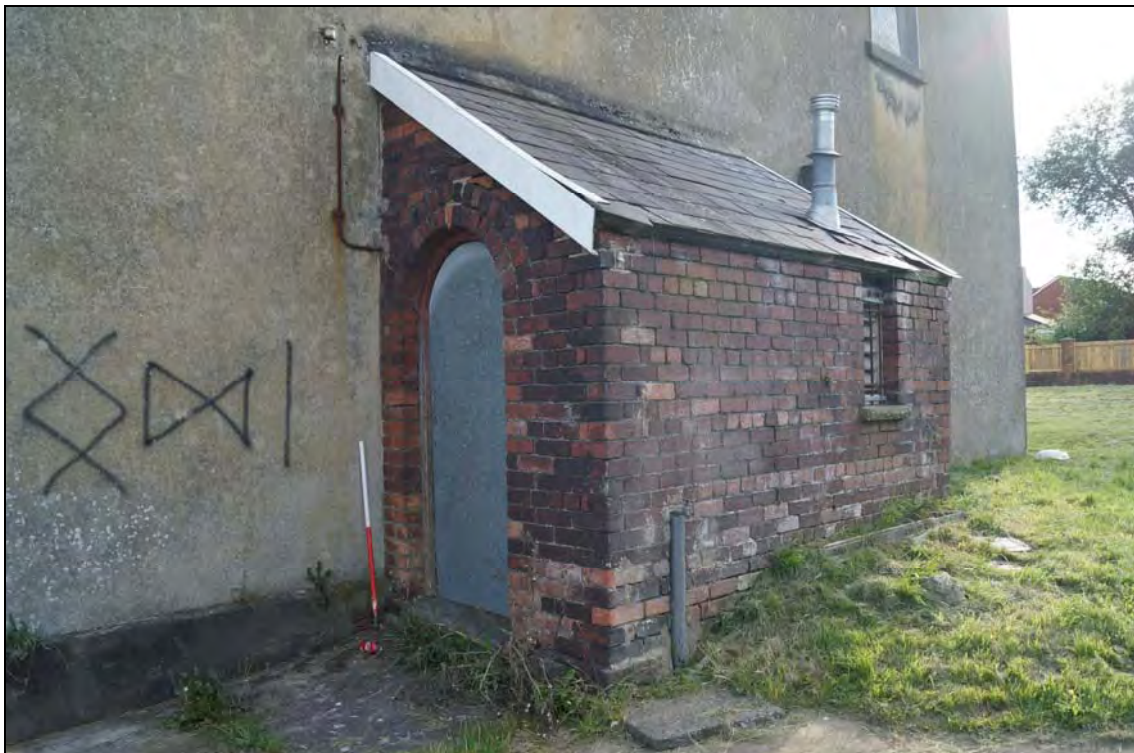
Plate 6: BTC2017_006, external view of boiler house attached to north side of chapel, looking southwest.
