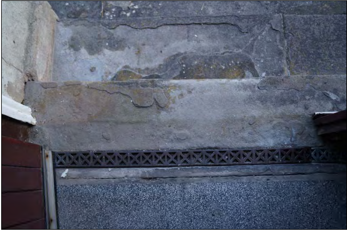
Plate 122: BTC2017_122, a view of the decorative metal grill in the threshold of the chapel entrance door, looking south-southwest.
