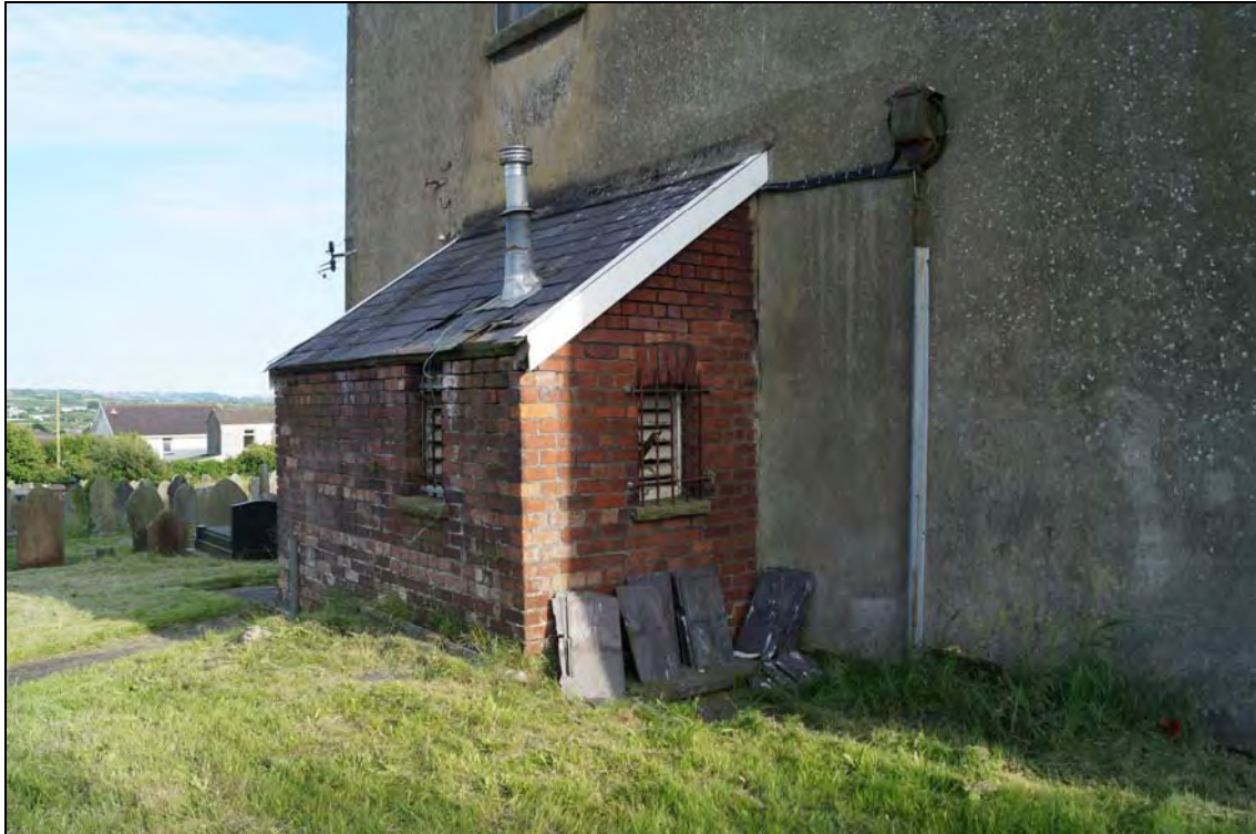
Plate 9: BTC2017_009, External view of boiler house attached to north side of chapel, looking southeast.
