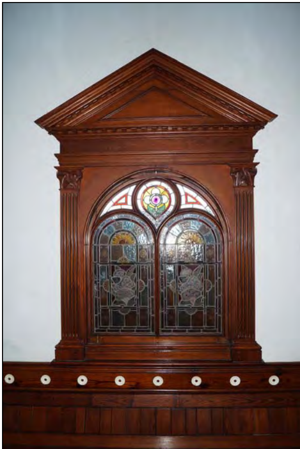
Plate 63: BTC2017_063, the highly decorative, stained-glass window in the wall which originally separated the entrance lobby from the main body of the chapel, looking south-southwest.
