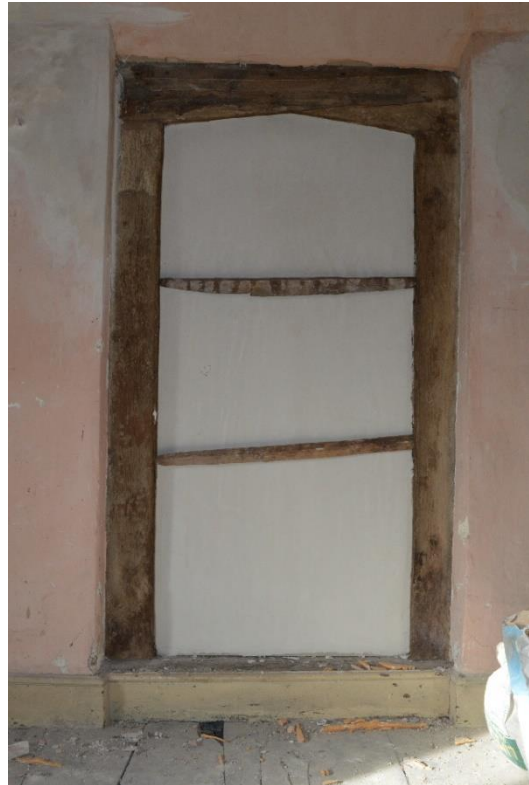
Fig. 6 The blocked dorrway on the second floor of the 17 th -century range. Photo CPAT 4246-0073
