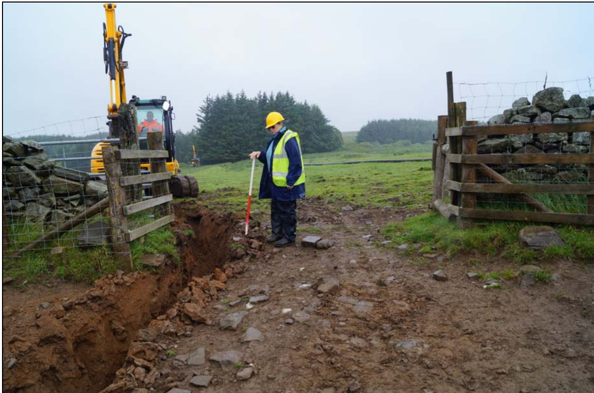
Plate 2: CNX2016_124. Excavation of the waterpipe/cable trench through the gateway to the east of the access track, looking northeast. The trench was at the northern side of the gateway, and avoided the tramway which passed 1 metre or so to the south.
