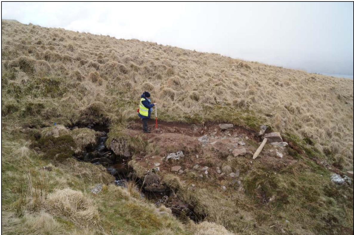
Plate 2: CNX2016_102, Cut created in slope to the southwest of the micro hydro intake, CNX2016_001, on the Nant Cnewr Fach to take the bypass water pipe when the intake was being built, looking southwest.
