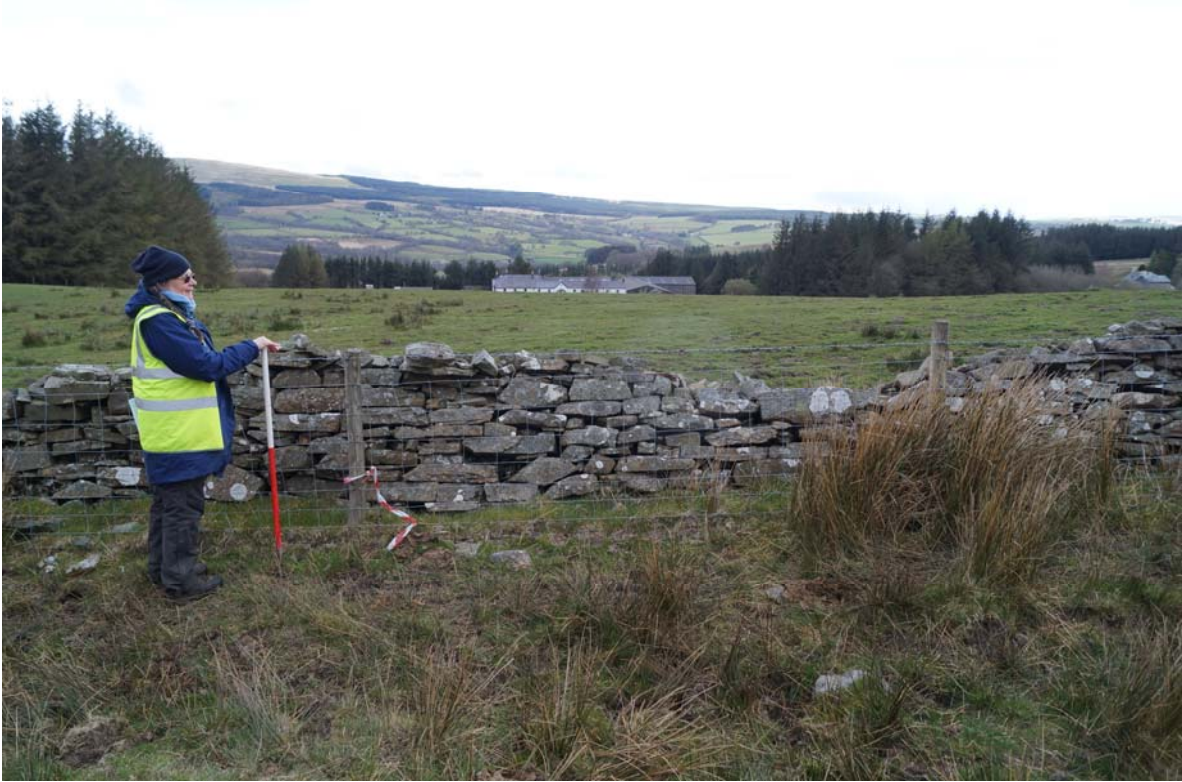
Plate 9: CNX2016_109, Boundary wall, CNX2016_005, at approximate location that the pipeline will pass through it, looking northwest.
