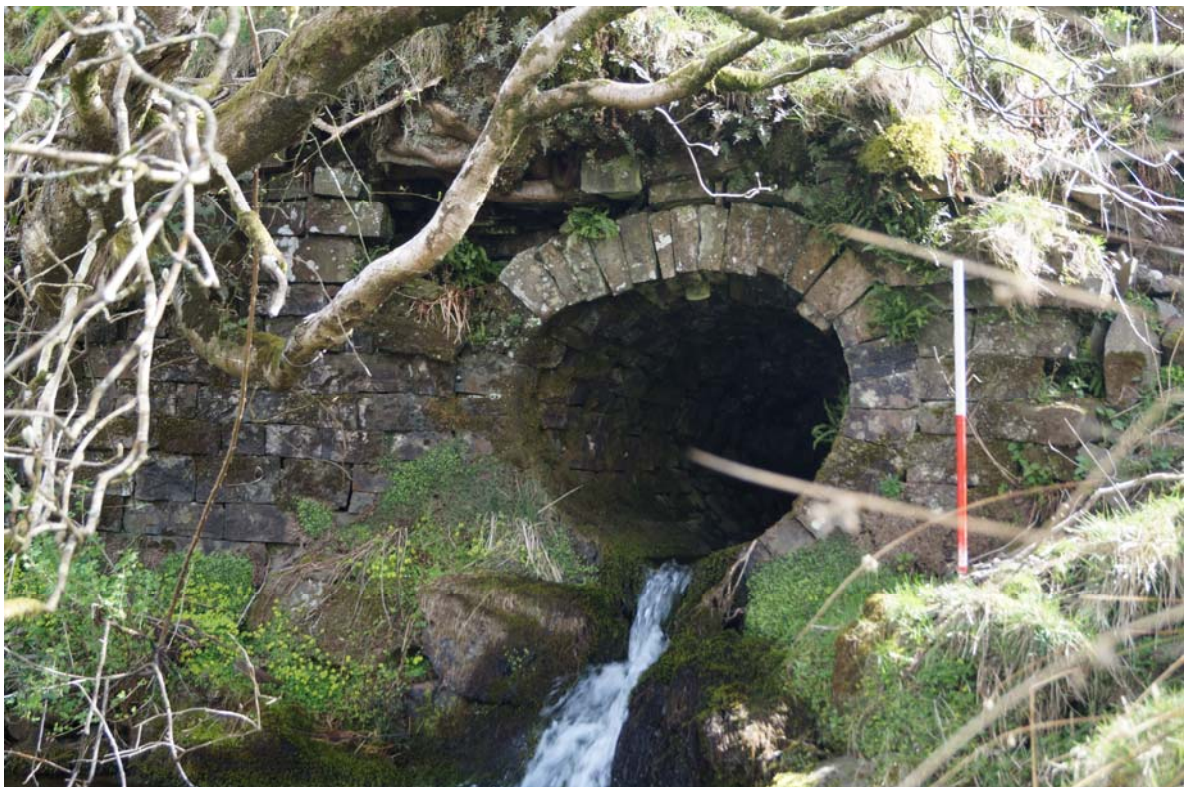
Plate 20: CNX2016_120, Detail of stone-built culvert pipe within the earth bridge CNX2016_010, looking east,
