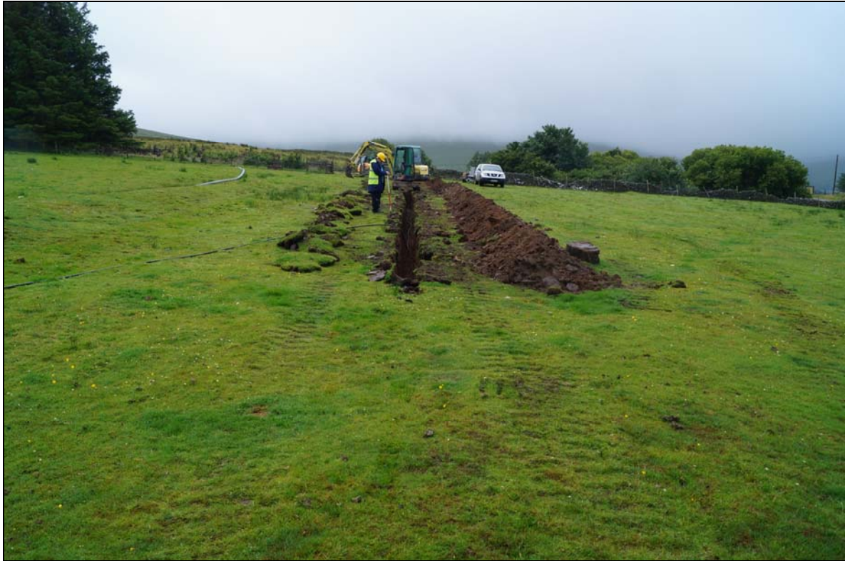
Plate 1: CNX2016_123. Excavation of the electricity cable trench, looking south southwest. The cable trench is to the north of the tramway.
