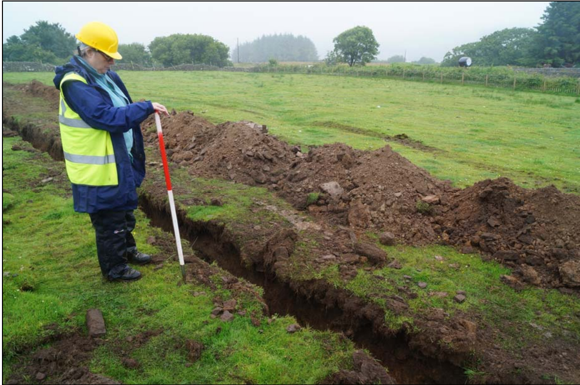
Plate 3: CNX2016_125. The excavated electric cable trench where it crossed the line of linear feature, CNX2016_009, looking southwest. Although the feature can be clearly seen crossing the field north of the trench, nothing was visible in the trench itself. Presumably the feature was shallow and had not cut the subsoil.
