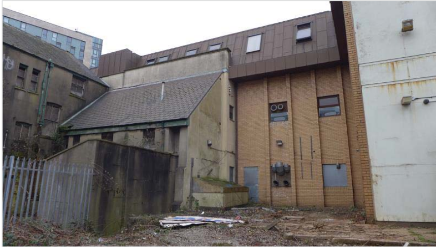
Figure 2.8: Rear façade of the Former Custom House showing late 20 th century structure
