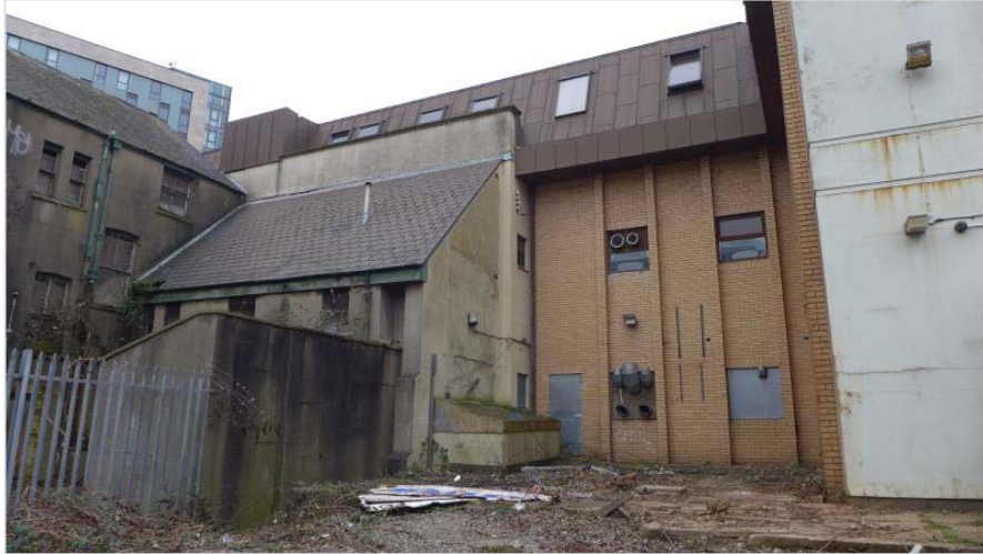
Figure 2.8: Rear façade of the Former Custom House showing late 20 th century structure
