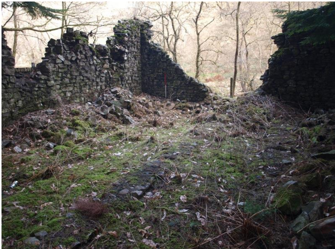
Fig. 24. Magazine (B1). Interior view looking north-east, showing the internal sleeper walls and collapse of the eastern wall.
